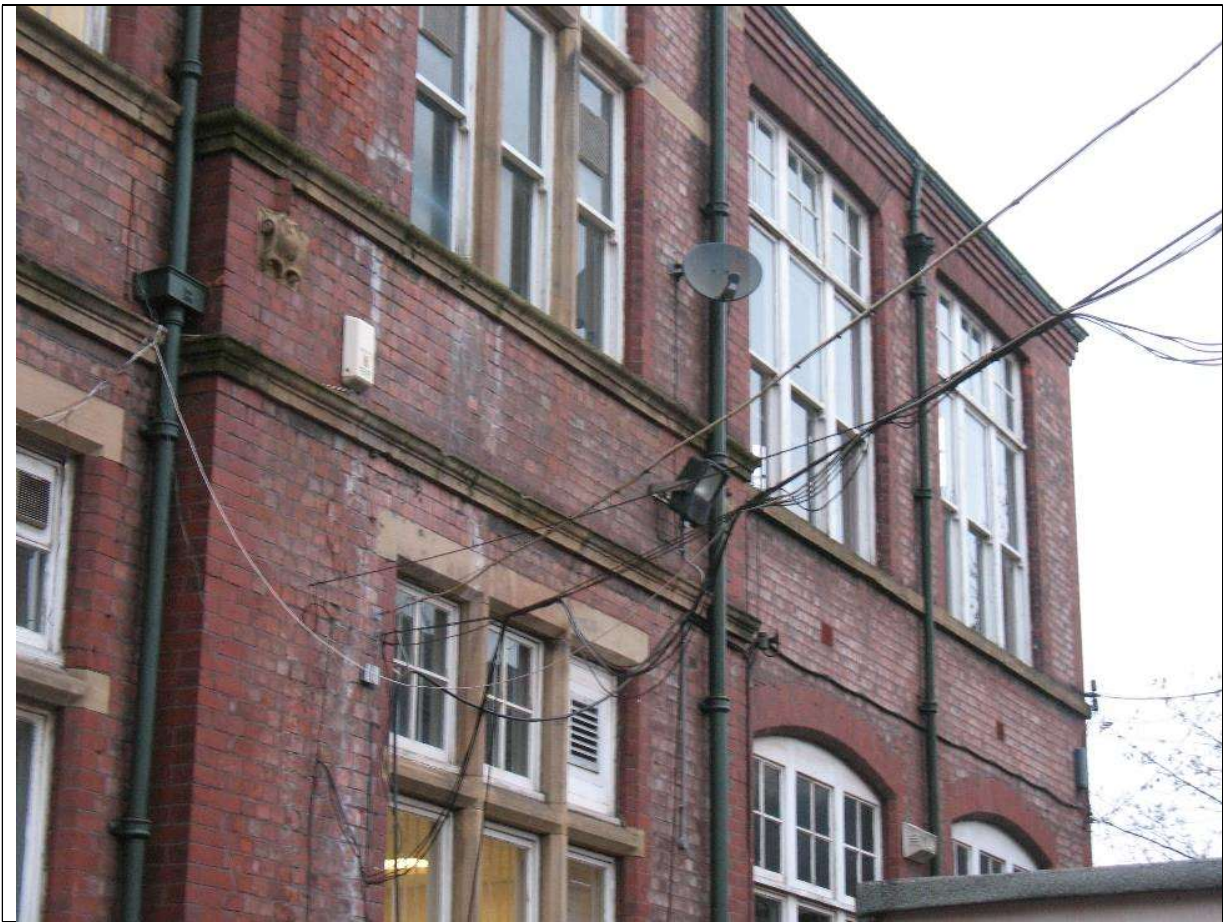
Photograph: 6 - Existing external intruder alarm sounder
