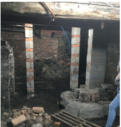
06 THE LEVEL 00 FLOOR IS SUPPORTED FROM VARIOUS AD-HOC STRUCTURAL SUPPORTS THAT HAVE BEEN DEEMED NOT FIT FOR PURPOSE BY THE STRUCTURAL SURVEY. THESE WILL BE REPLACED WITH NEW STRUCTURAL ELEMENTS TO BE SYMPATHETIC TO THE ORIGINAL FABRIC.
