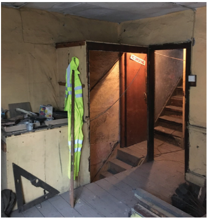
04 ORIGINAL TIMBER ENCLOSURE AROUND THE LEVEL 01 STAIR. THIS DOES NOT COMPLY WITH CURRENT BUILDING REGULATIONS (AD PARK B AND K) AND AS SUCH IS PROPOSED TO BE REPLACED WITH A FULL HEIGHT PARTITION.
