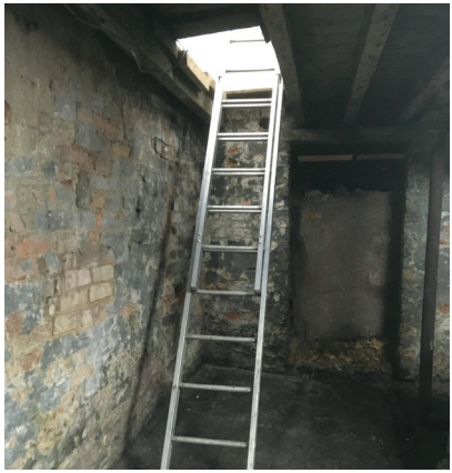
01 THERE IS CURRENTLY NO SAFE, BUILDING REGULATIONS COMPLIANT ACCESS TO THE BASEMENT LEVEL. THIS PHOTOGRAPH ILLUSTRATES THE CURRENT TEMPORARY ACCESS PROVISION VIA A LADDER
