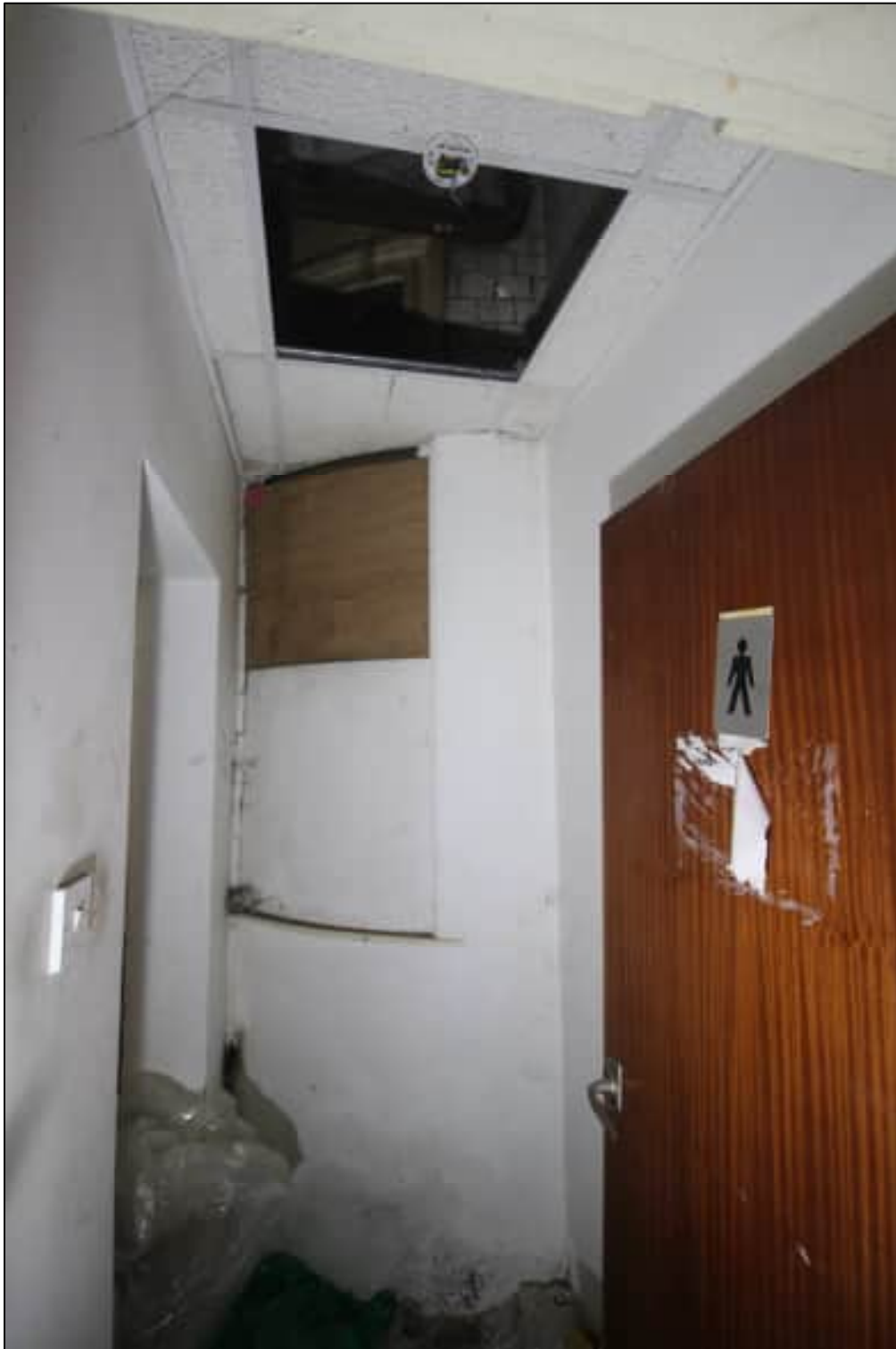
Plate 35: General view of Room 4, looking east
