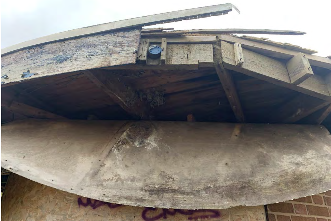
Photograph 17 - Gaps into roof timbers on southern aspect of B1
