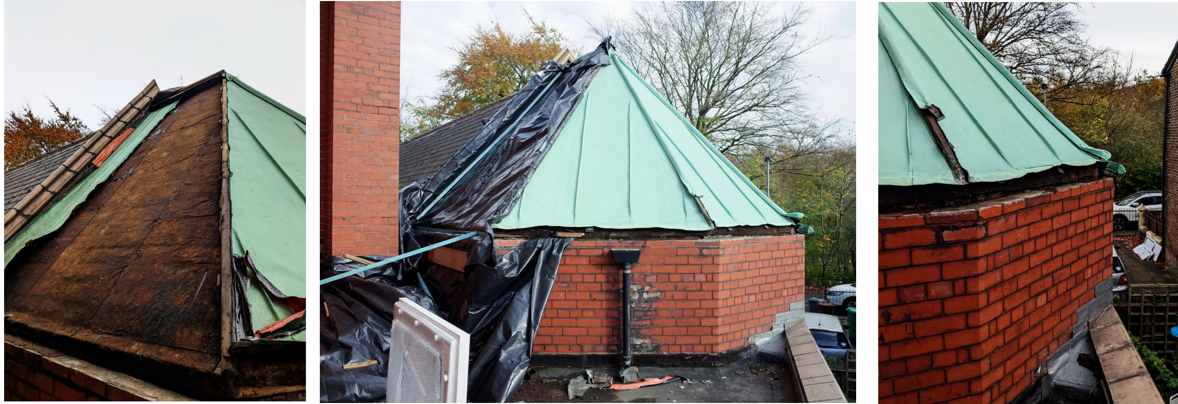
Condition following ongoing theft
