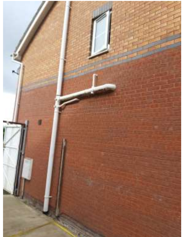
Above: Side View showing meter behind gate
