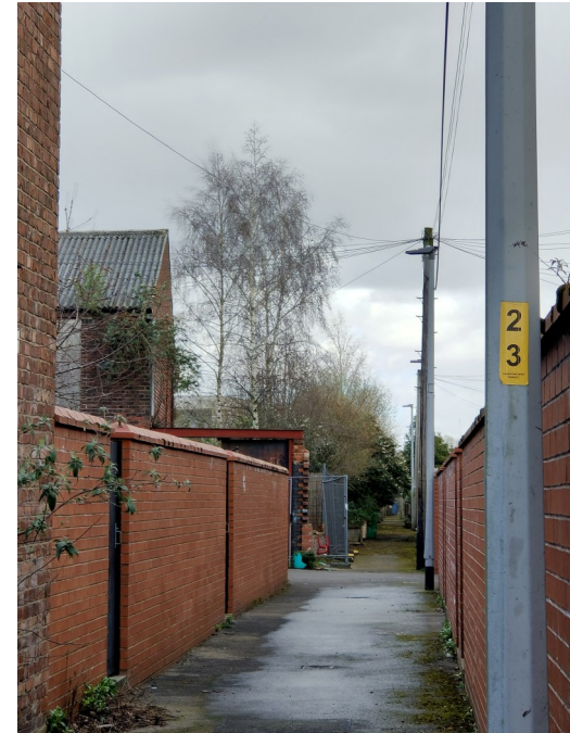
Below—View down alley showing dilapidated yard wall protected by herras fencing
