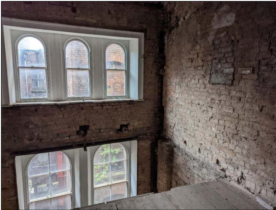
Plate 87: Southwest corner showing removed floor
