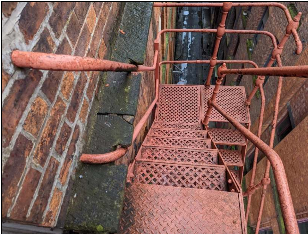
Plate 109: Inserted fire escape to Reyner Street cutting sandstone string course
