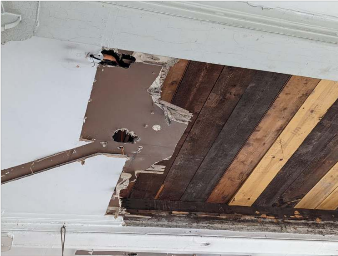
Plate 73: Original lath and plaster with modern boards shown above
