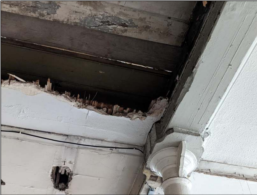
Plate 69: Broken lath and plaster ceiling
