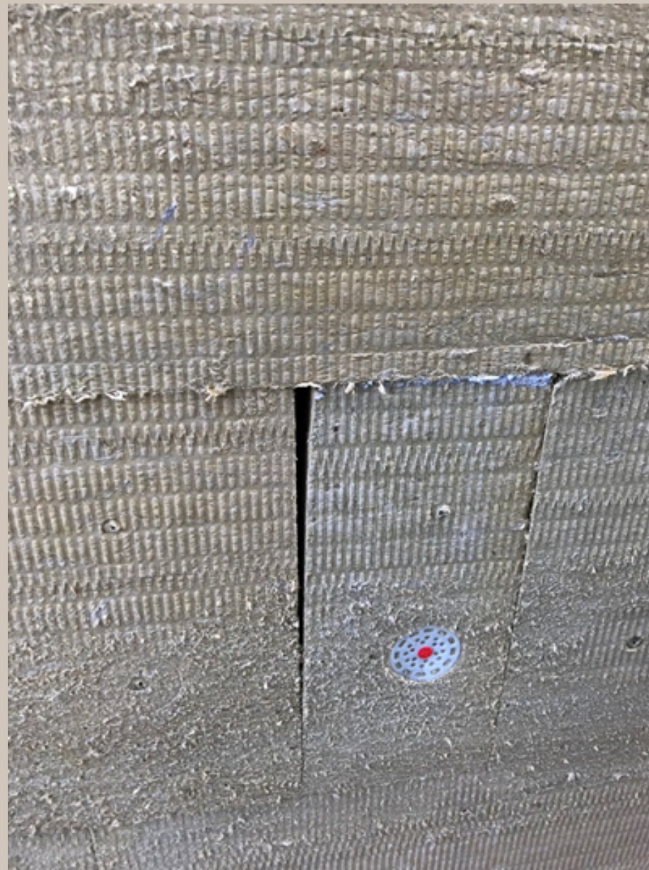
Gaps within boarding
