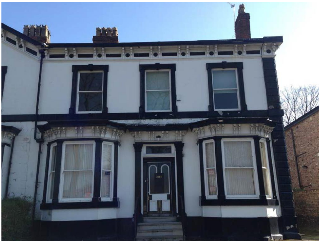
Plate 1: Front Elevation, provided by Orco Heritage Statement 2014 (revised 2016) showing poor condition of building prior to conversion to flats
