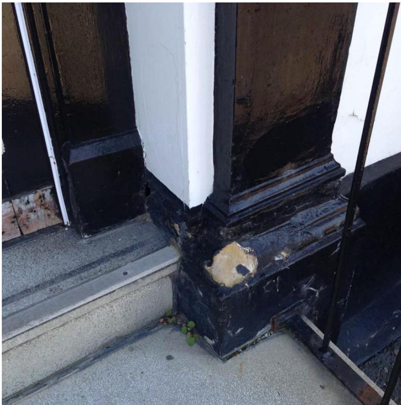
Plate 15: Detail of Facade, provided by Orco Heritage Statement 2014 (revised 2016), showing poor condition of exterior prior to conversion
