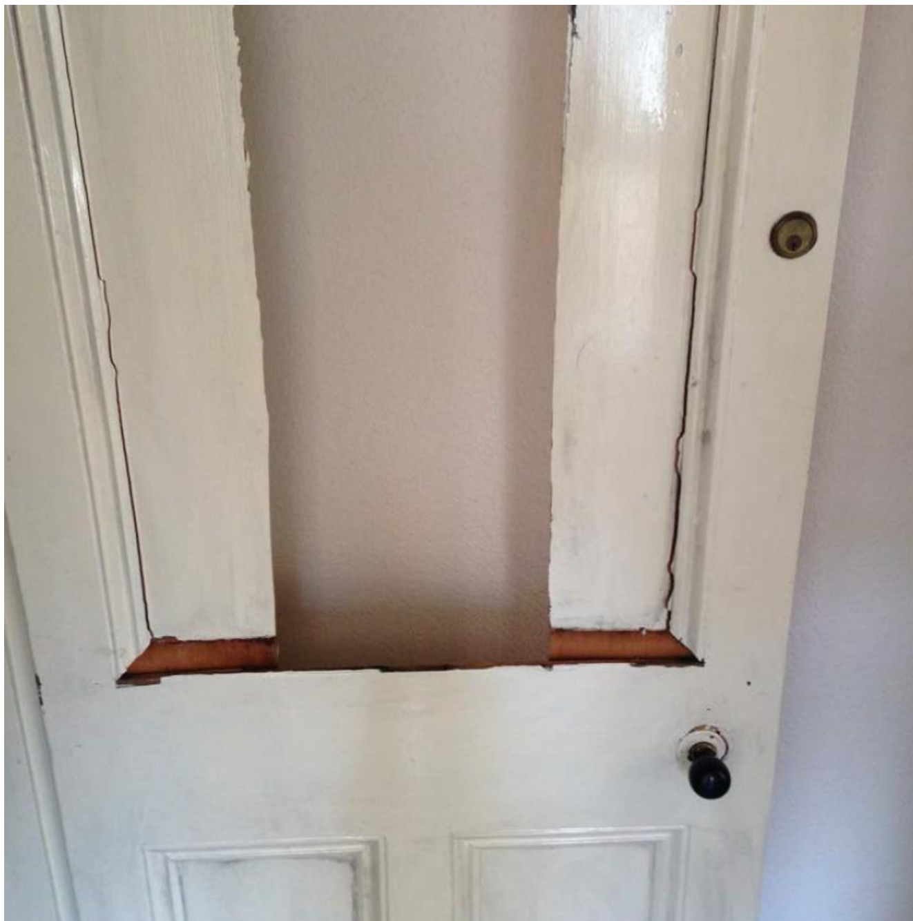
Plate 10: Damaged Door, provided by Orco Heritage Statement 2014 (revised 2016)
