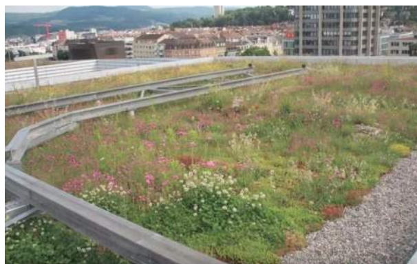
Figure 6—2 Jakob Burkhardt biodiverse roof (Basel, Switzerland)
