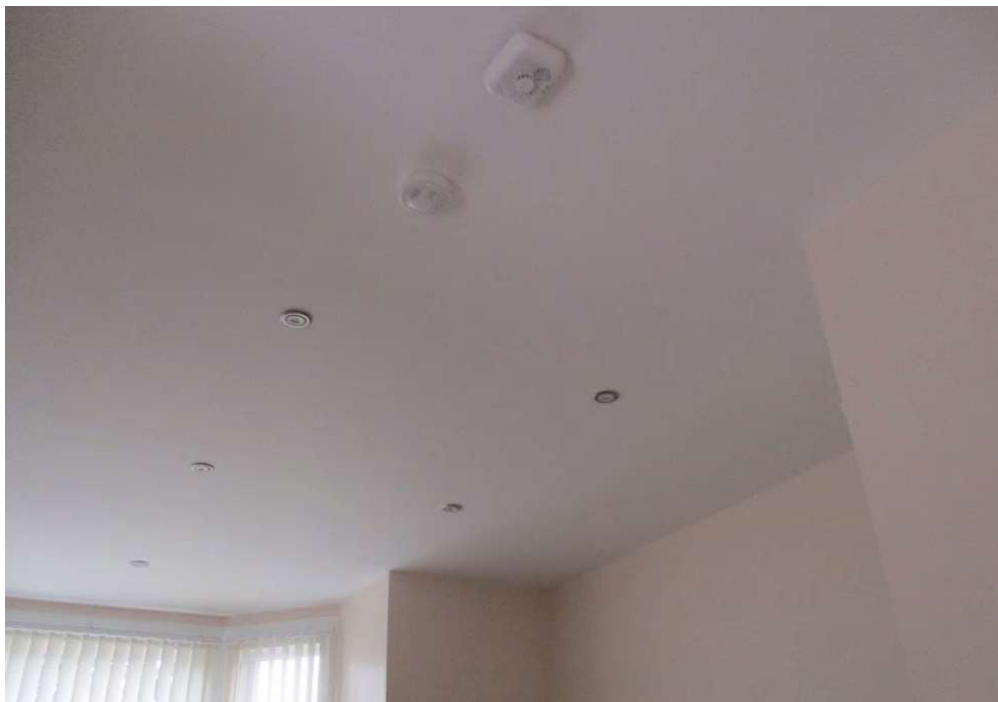
Fig 5. Internal room with bay window showing lowered ceiling and loss of original height, decorative cornice and timber panelling.
