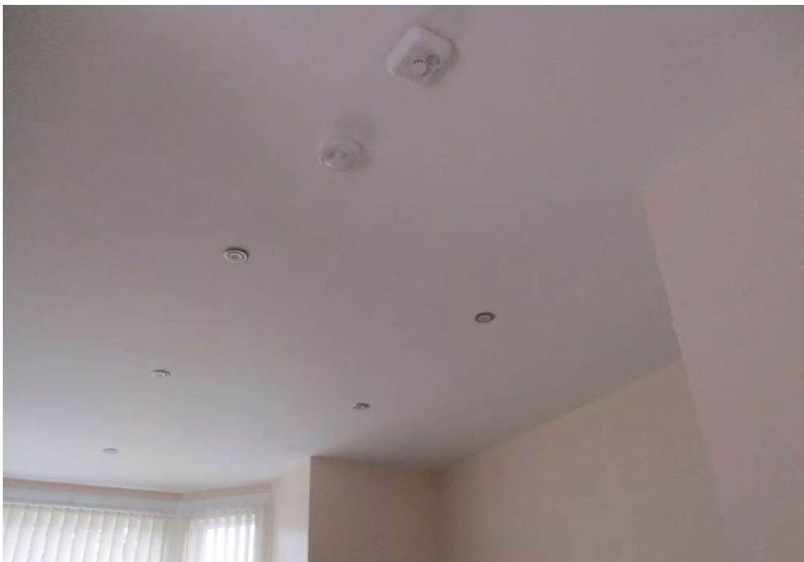
Fig 28. Internal view of principle rooms at No. 363 showing removal timber panelling and lowered ceiling and subsequent loss of detailing and features.
