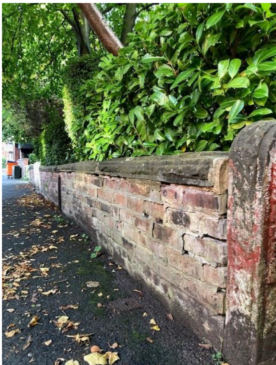
Figure 3: Damaged wall, view facing southeast.
