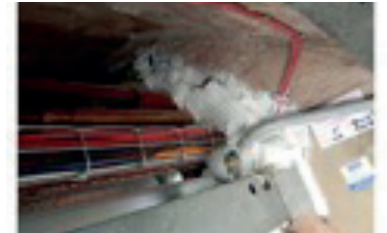
Example location where the existing fire stopping needs to be replaced. New matching brickwork may be required if the extent of the batt can be reduced and brick reinstated instead.
