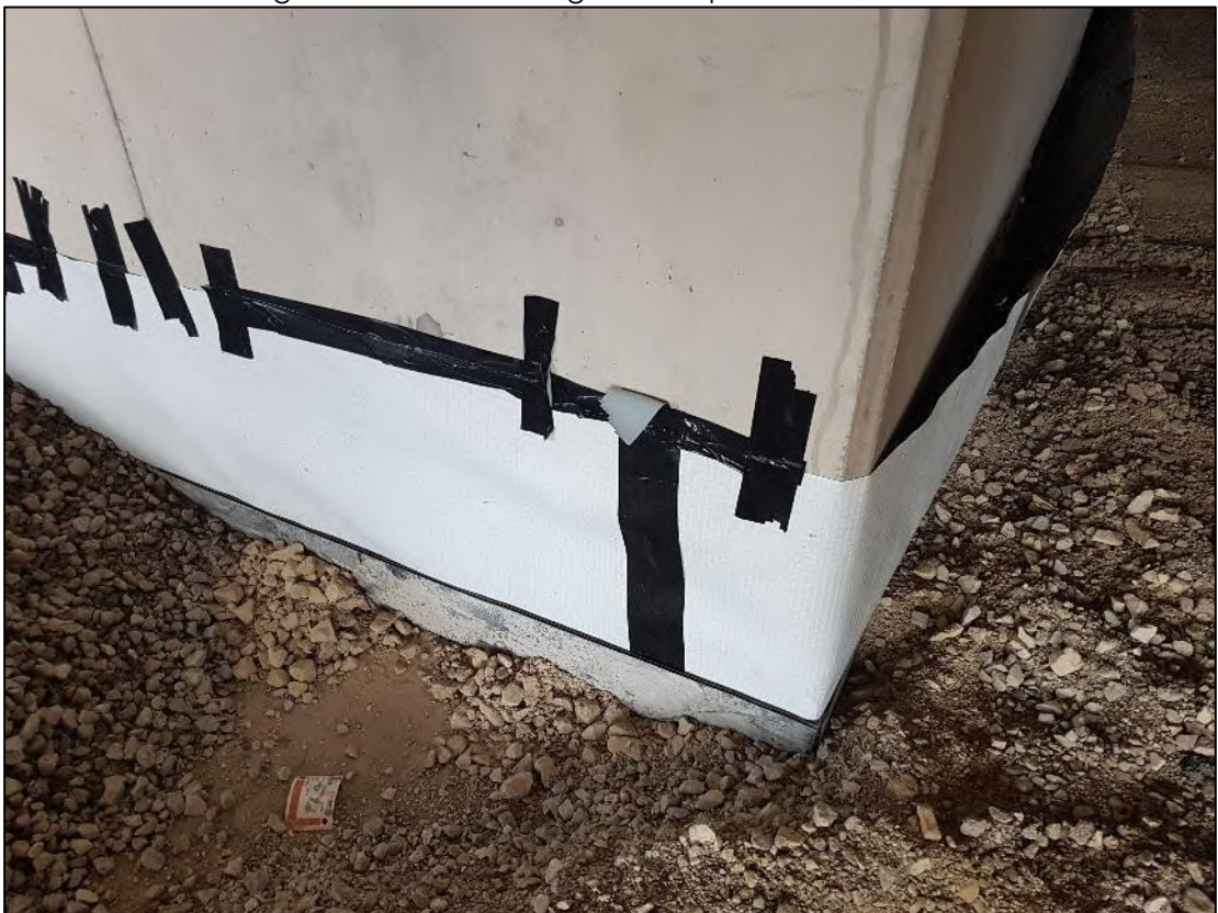
Figure 2: Photo showing southern area prior to installation
