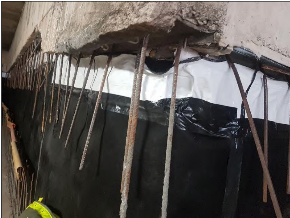
Figure 20: Membrane installation on central corner needed repair
