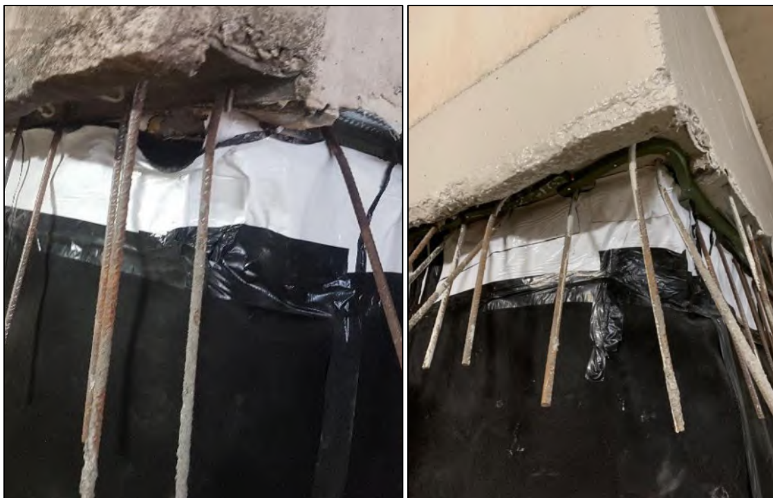
Figure 2: Photos showing defect and repair on corner of contiguous pile wall.
