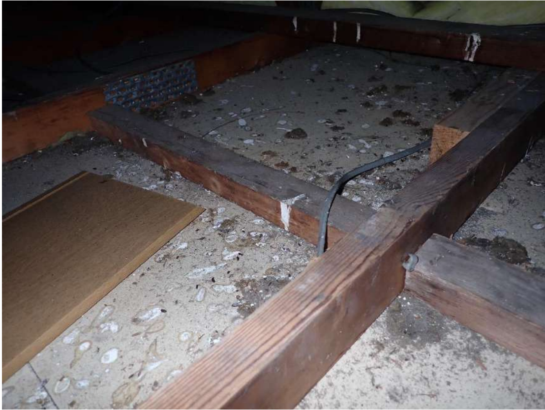
Photograph 17. The bird droppings in the loft space of Flat 9.
