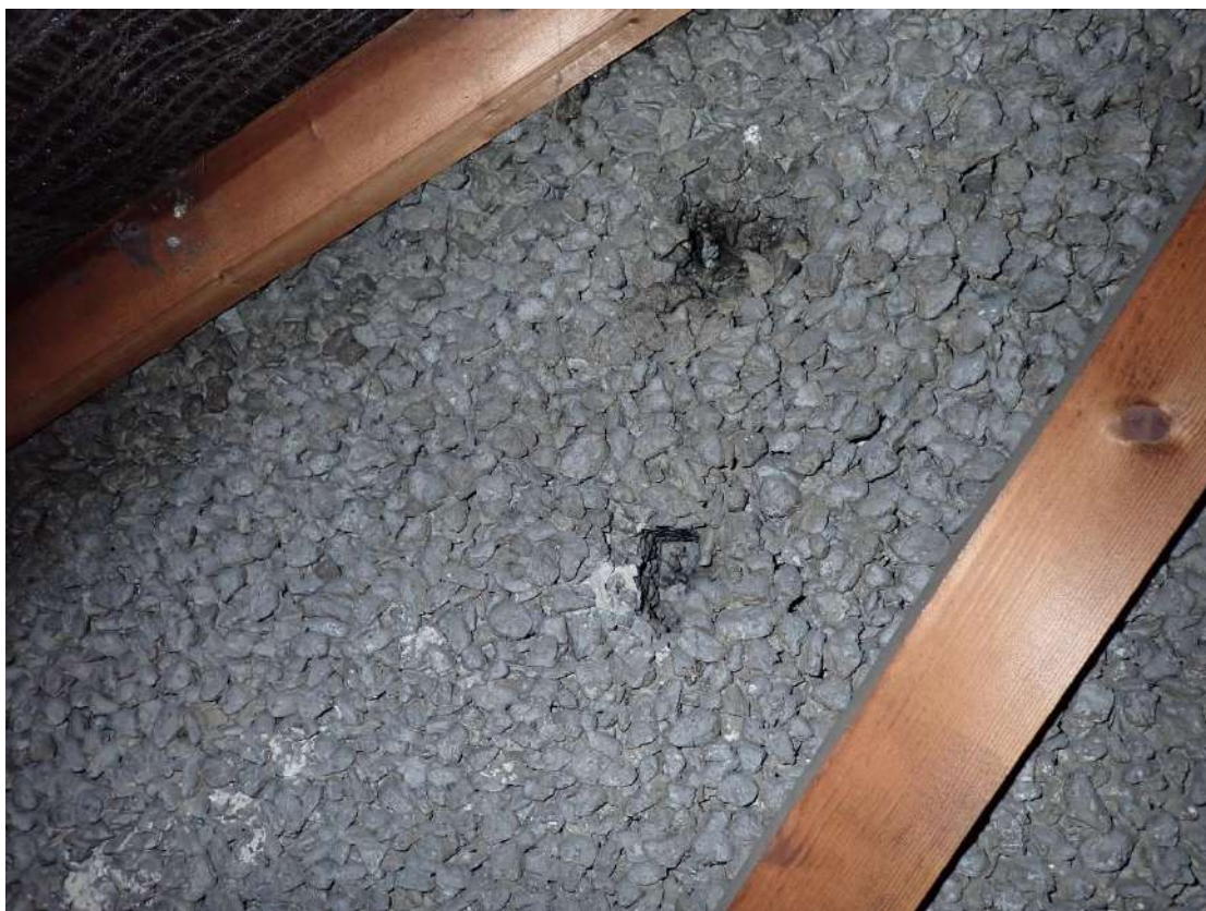
Photograph 15. The cavities in the stone render wall, in the loft space of Flat 9.
