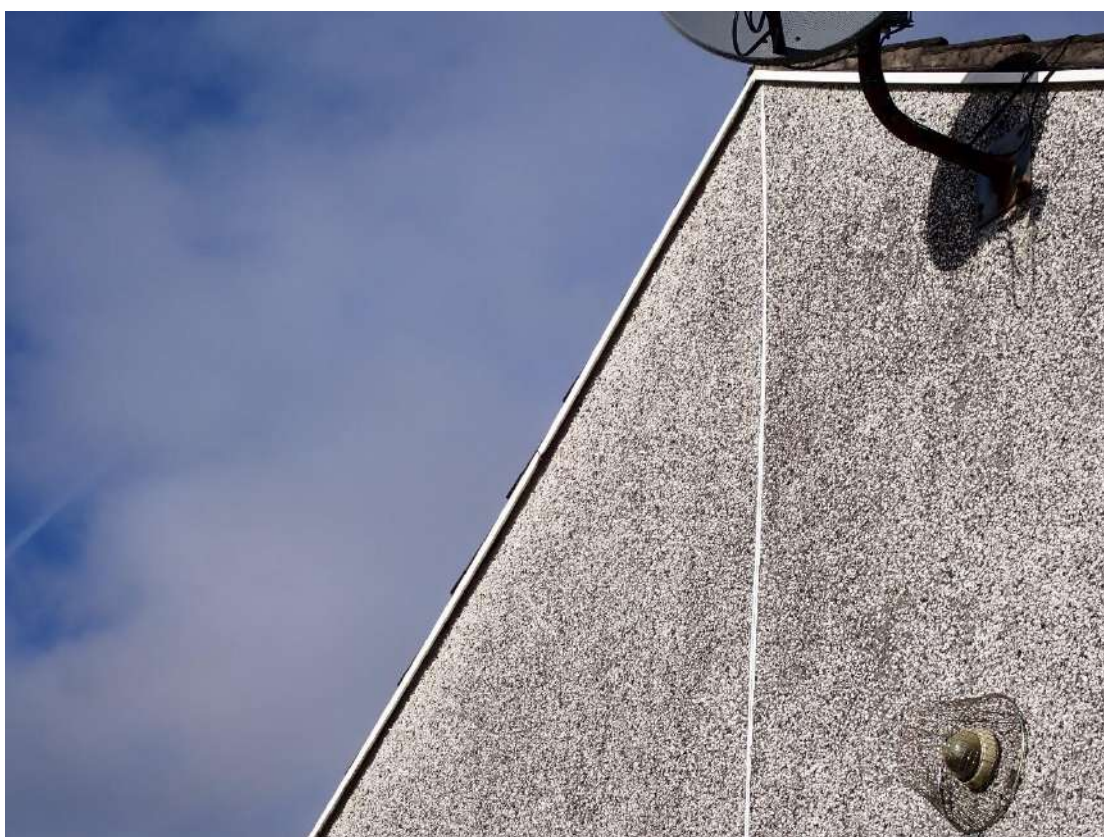
Photograph 8. The gaps underneath the PVC capping on the southern aspect of the building.
