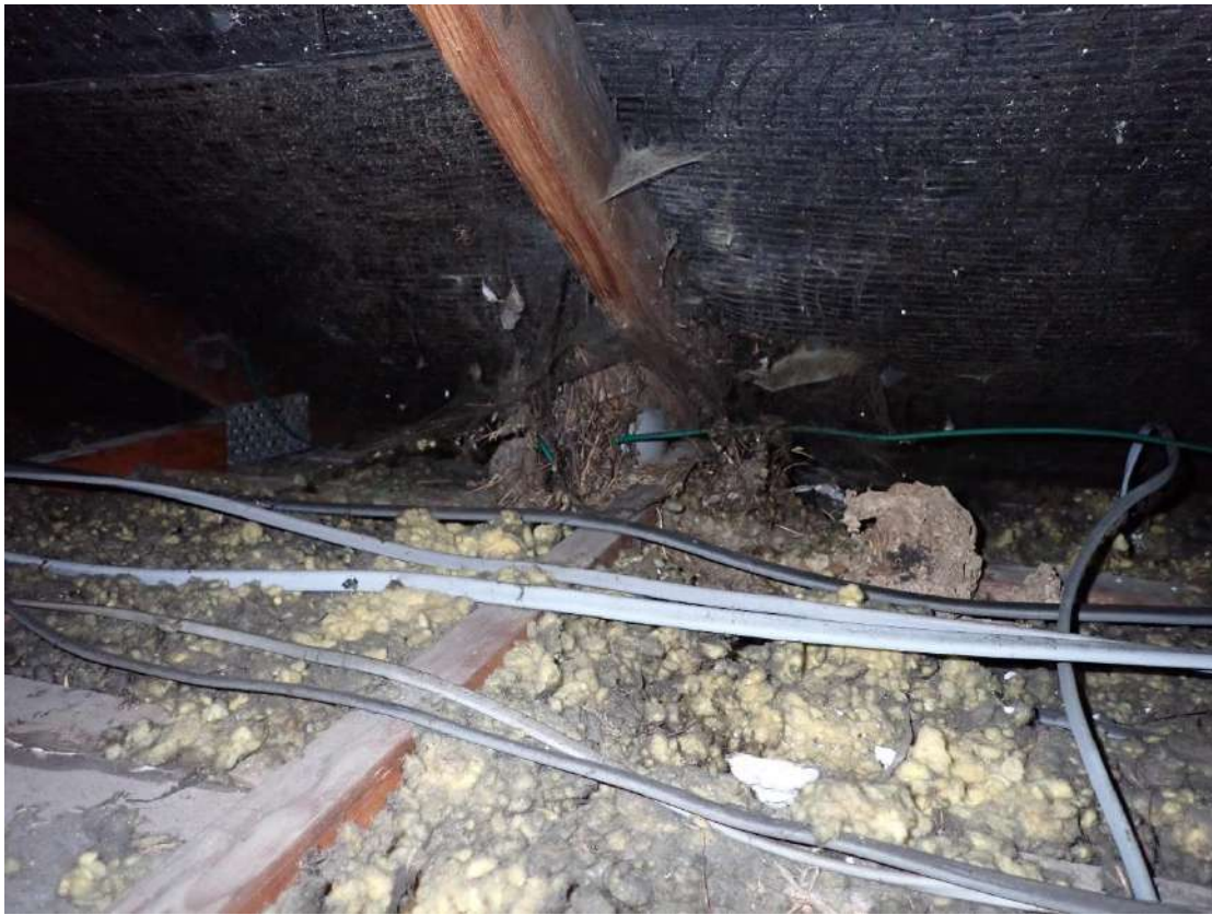
Photograph 19. House sparrow nest identified in the loft space of Flat 11.
