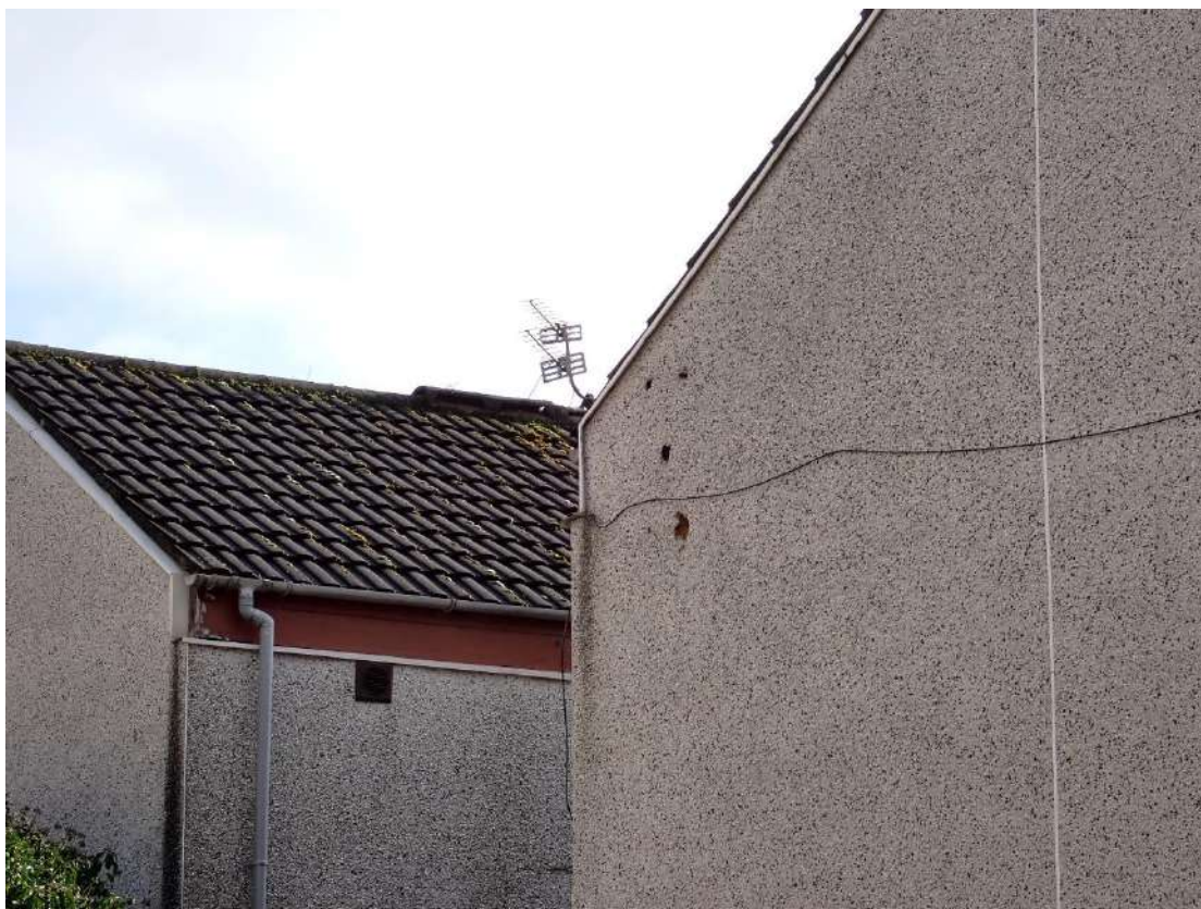
Photograph 11. Four holes located on the northern aspect of the building.
