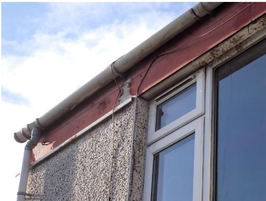
Photograph 9. A small gap between the wooden barge board and the top of the wall plate on the eastern aspect.
