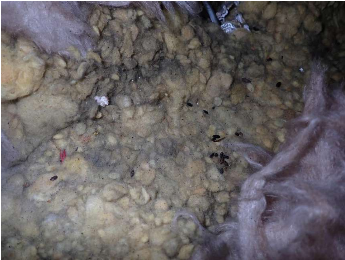
Photograph 22. Mouse droppings identified in the loft space of Flat 13.
