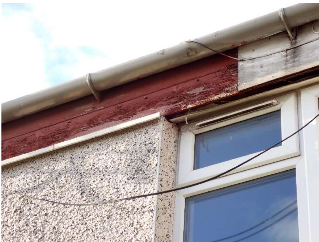
Photograph 10. A gap between the top of the wall plate and barge board on the eastern aspect.
