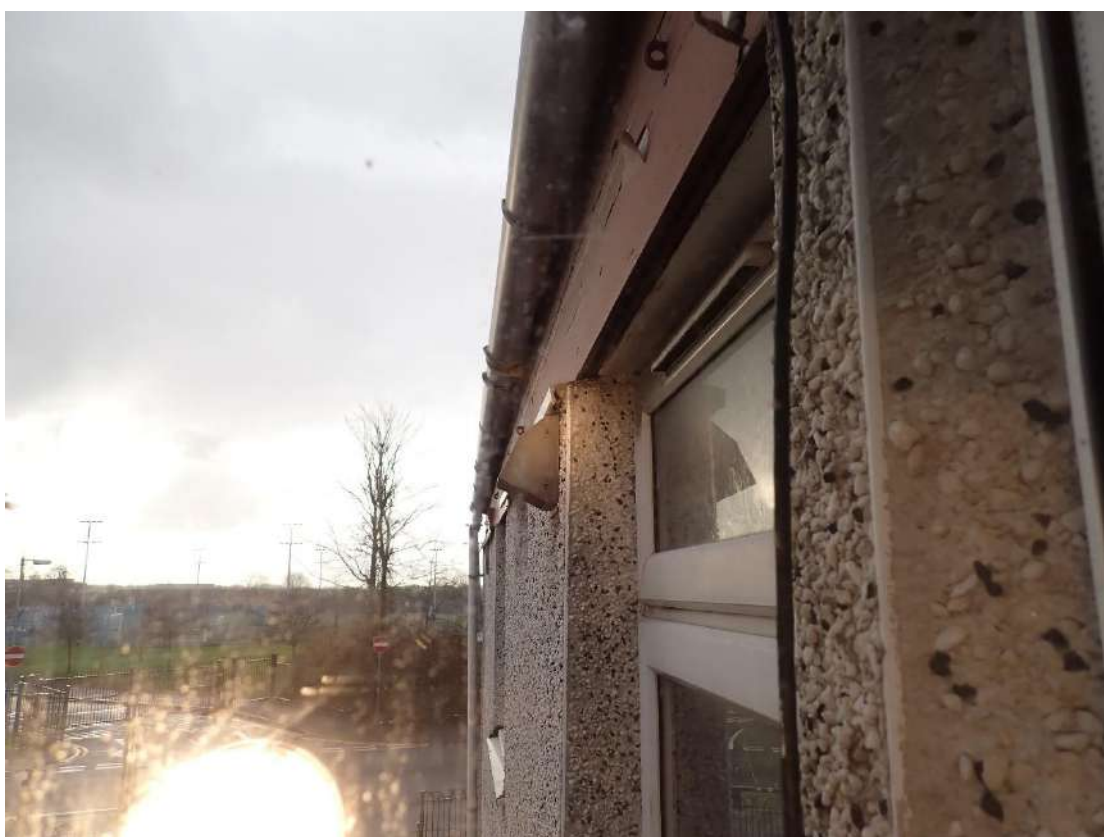
Photograph 6. The gap between the wooden barge board and the top of the wall plate on the eastern aspect of Flat 15. Also, the gap between the PVC capping and the ventilation cover.
