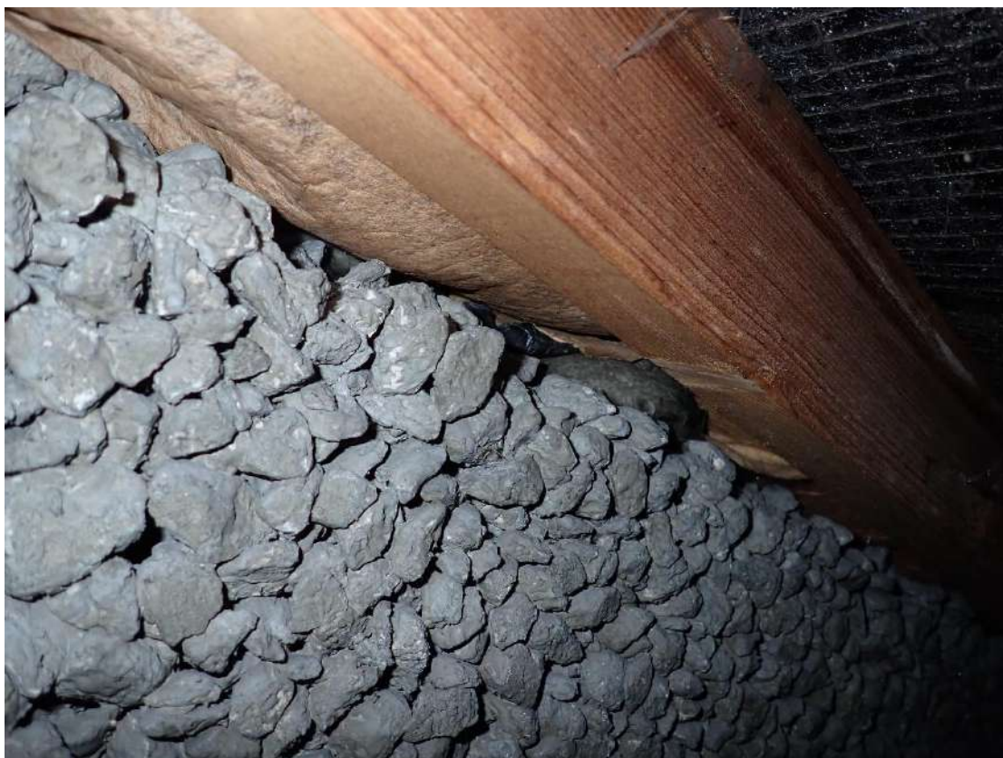
Photograph 23. The gap around the top of the wall plate in the loft space of Flat 15.
