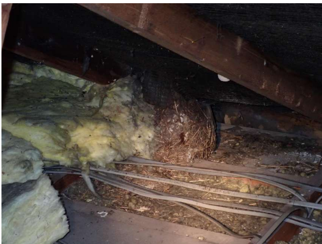
Photograph 16. The bird's nest identified in the loft space of Flat 9.
