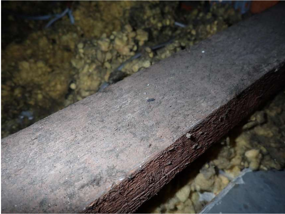
Photograph 21. Mouse droppings identified in the loft space of Flat 11.
