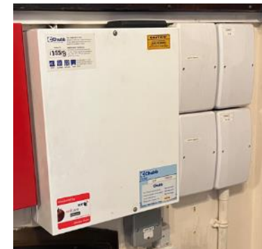
Existing panel located in security hut.
