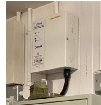
Existing panel located in reception office
