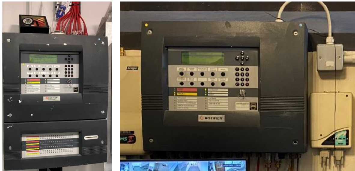
Existing Fire panel in extension
