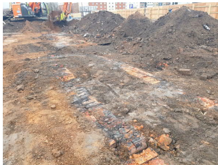
Photograph 4. Evidence of sub-surface obstructions
