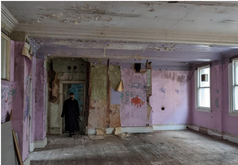
Recent interior views of Level 3, showing signs of water ingress and previous occupation
