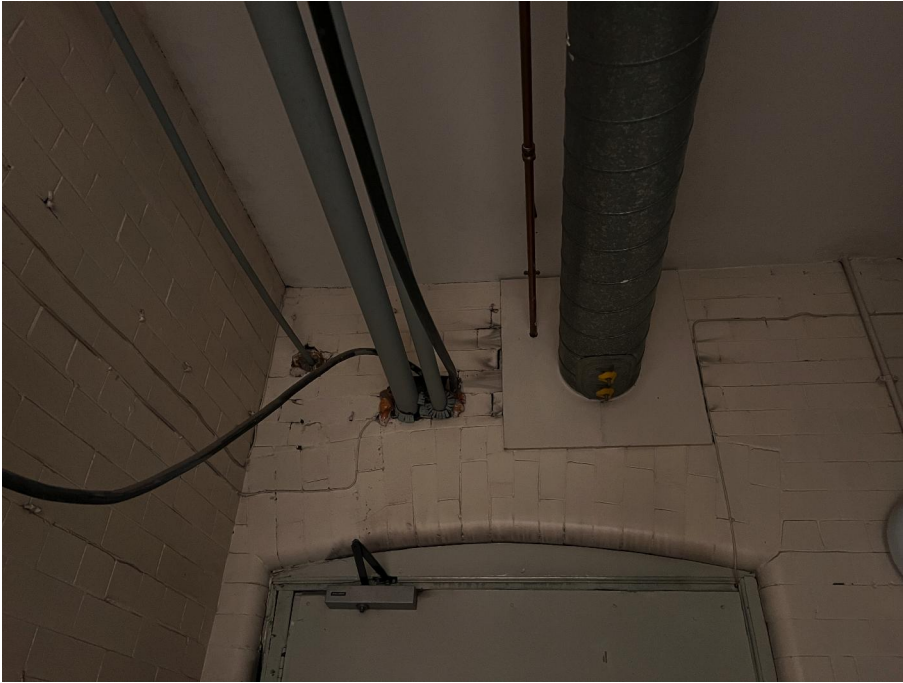
EXISTING DUCT, PIPED SERVICES AND CABLES PASSING THROUGH EXISTING PENETRATIONS IN MASONRY WALL
