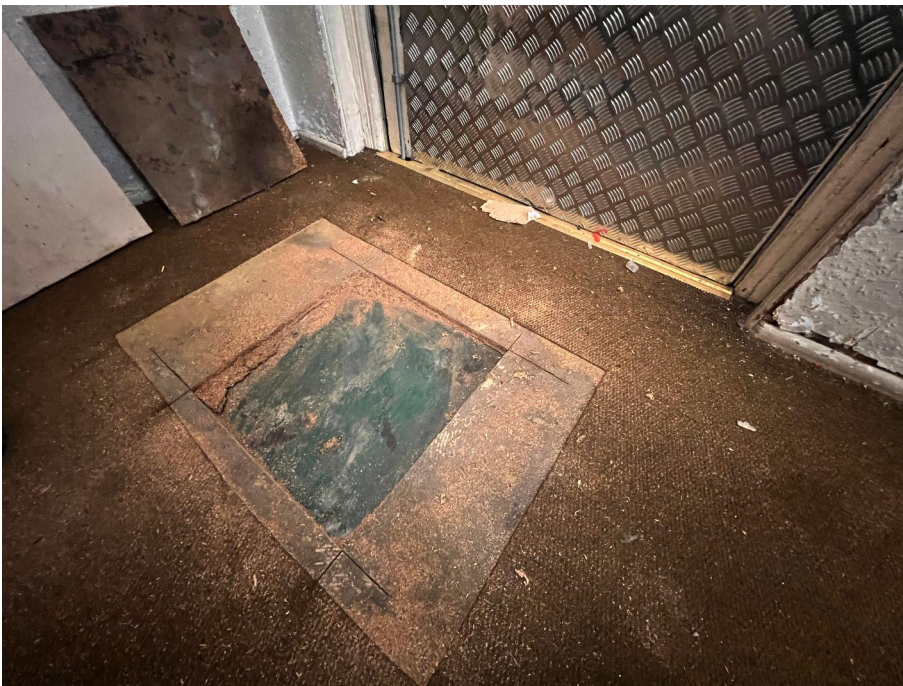
MORE DETAILED PHOTOGRAPH OF THE ABOVE SHOWING THE EXISTING CHIPBOARD BUILD-UP OVER MASTIC ASPHALT SUBFLOOR
