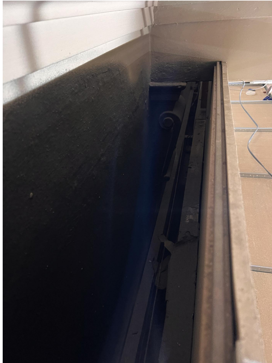
PHOTOGRAPH SHOWING VOID BEHIND EXISTING WALL LININGS
