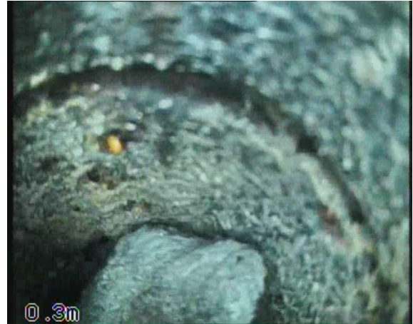
HOLX_766d2511-d82f-4ba7-818f-dfc7d98f24ac_20230911_094402_437.jpg, 00:00:21, 0.40 m Other obstacles from 12 o'clock to 12 o'clock, 90% cross-sectional area loss, Rock
