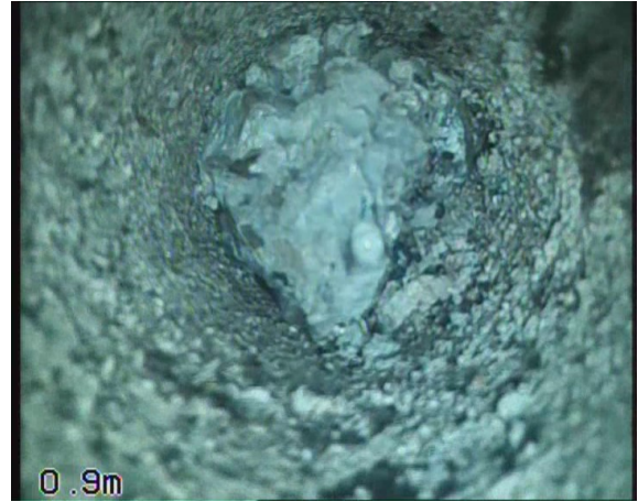
HOLX_35e16080-5ab1-4555-b8e7-b6d411affb86_20230911_093055_456.jpg, 00:00:22, 1.00 m Other obstacles from 12 o'clock to 12 o'clock, 100% cross-sectional area loss, Concrete / Obstruction
