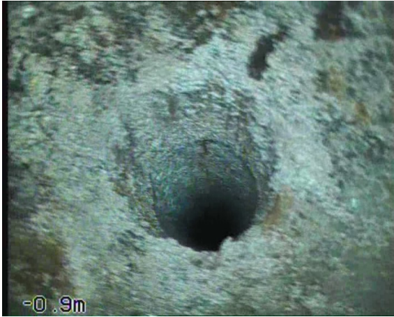
RWDP5 (F1)X_efb2363e-2886-444a-8997-af438b027e44_20230911_093240_631.jpg, 00:00:00, 0.00 m Start node, major connection without manhole, reference: RWDP5 (F1)
