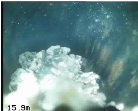
HOLX_fd5669b4-efff-4b5d-9077-7f1b6216390f_20230908_113147_577.jpg, 00:01:14, 15.90 m Settled deposits, coarse, 25% cross-sectional area loss, Stones
