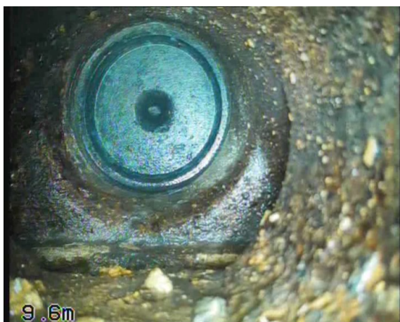
HOLX_635b2e72-483c-4576-8c41-43bc37262ae1_20230908_103307_029.jpg, 00:00:51, 9.80 m Finish node, gully, reference: HOL
