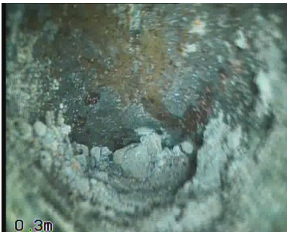
HOLX_73bb7369-ef62-467b-b60c-dcb347e2b7a8_20230911_092255_247.jpg, 00:00:22, 0.30 m Attached deposits, encrustation from 3 o'clock to 9 o'clock, 50% cross-sectional area loss
