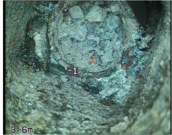
HOLX_d7430d71-9515-436e-bcef-ad2dbcc7a75a_20230911_090507_425.jpg, 00:00:34, 3.60 m Finish node, major connection without manhole, reference: HOL
