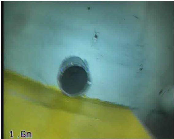
HOLX_3f5dec2a-b118-4d63-a779-dbe6a11a6328_20230911_091508_674.jpg, 00:00:00, 0.00 m Start node, major connection without manhole, reference: RWDP1 (F1)
