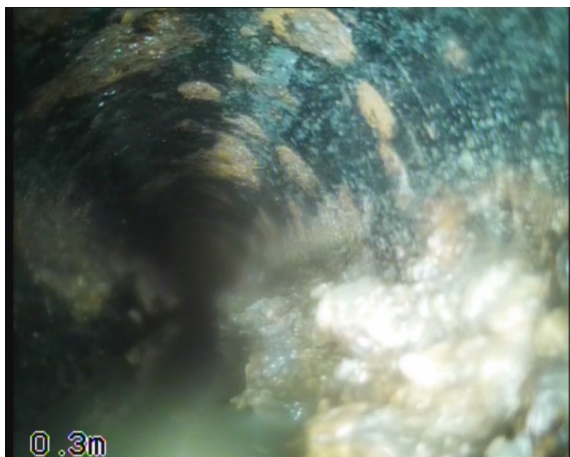
MH7X_05b1cd5e-9e6c-4792-83ce-61d97ae24e37_20230908_122529_746.jpg, 00:00:08, 0.30 m Attached deposits, encrustation from 3 o'clock to 6 o'clock, 25% cross-sectional area loss
