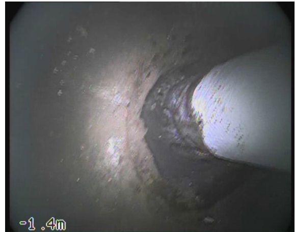
RWDP5 (L1)X_c49708bb-b0a7-49dd-b10f-ea25c05b995b_20230908_101722_352.jpg, 00:00:00, 0.00 m Start node, major connection without manhole, reference: RWDP5 (L1)
