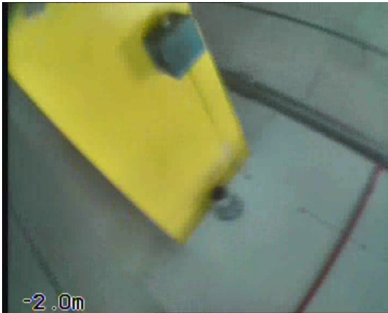
HOLX_971db663-340b-43c1-ab77-c51e8f2cf3ec_20230911_092157_832.jpg, 00:00:00, 0.00 m Start node, major connection without manhole, reference: RWDP2 (F1)
