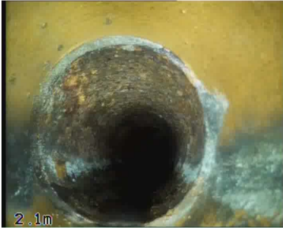
HOLX_ebed43cd-c34f-4d7b-b7d4-5a171220b17d_20230908_105219_386.jpg, 00:00:14, 0.20 m Pipe material changes to cast iron at this point
