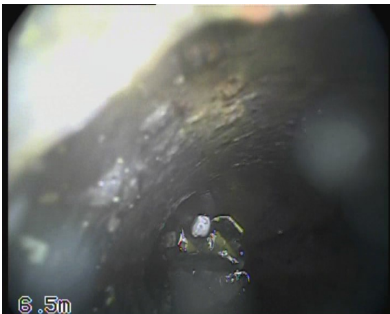
RWDP6 (L1)X_c24db34c-f1e1-4a54-bbe5-7b7f02461667_20230908_1 02538_566.jpg, 00:00:54, 6.50 m Other obstacles from 12 o'clock to 12 o'clock, 75% cross-sectional area loss, Obstruction
