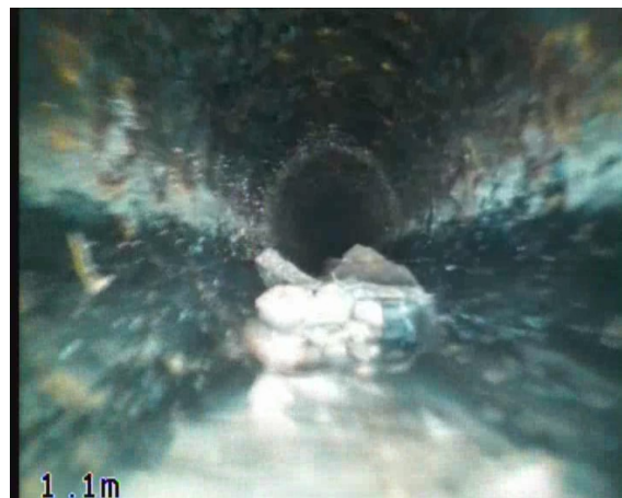
HOLX_7026859b-40d0-4aca-84e8-937f54658df8_20230908_103745_461.jpg, 00:00:13, 1.20 m Settled deposits, coarse, 20% cross-sectional area loss
