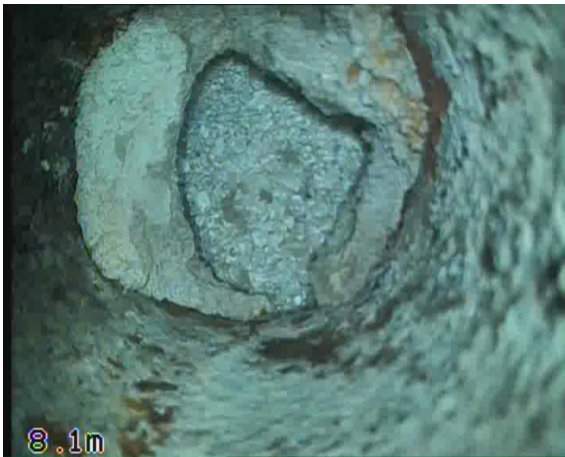
HOLX_3025dfa4-df78-46f9-8c50-3b51d50e22d2_20230911_090250_497.jpg, 00:00:54, 8.20 m Other obstacles from 12 o'clock to 12 o'clock, 100% cross-sectional area loss, Obstruction
