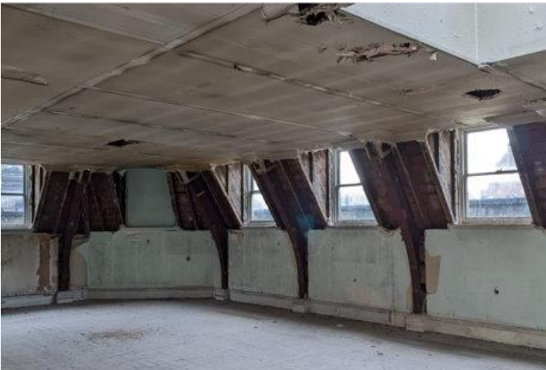
Recent interior views of Level 4, showing signs of water ingress.
