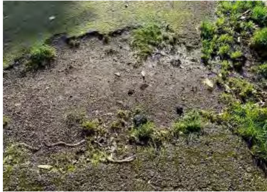
Condition of areas of macadam footpaths
