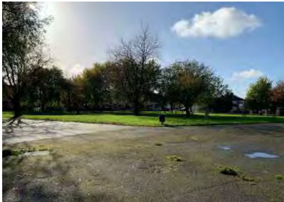
Macadam to central area showing signs of disrepair
