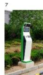
7 2no EV charging points
