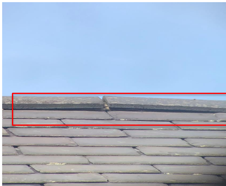
PLATE 7 SHOWING GAPS UNDER RIDGE TILES
