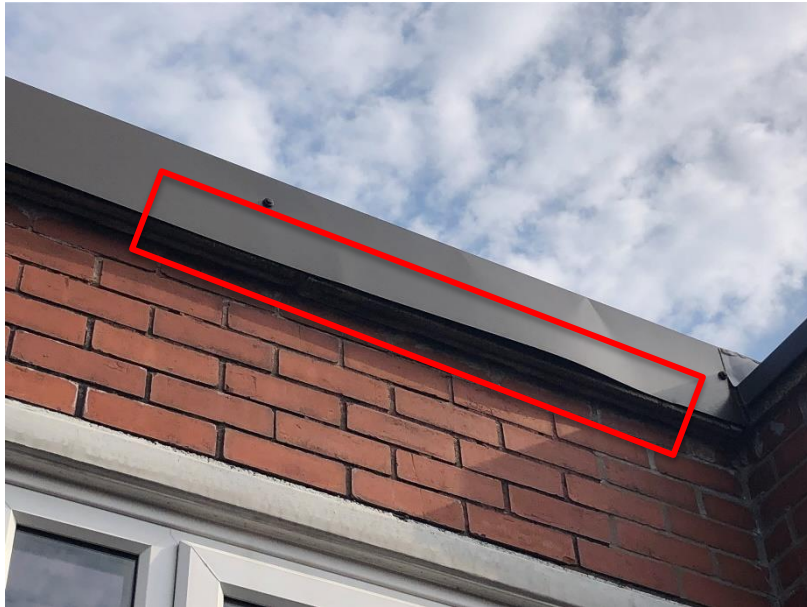
PLATE 2 SHOWING GAPS PRESENT ON SOUTHERN ASPECT OF WESTERN EXTENSION
