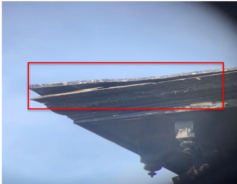
PLATE 11 SHOWING SPLIT ON SOUTH-WESTERN ASPECT OF BUILDING 2
