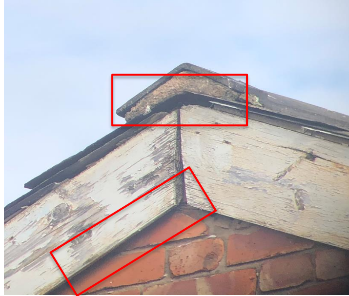
PLATE 8 SHOWING GAPS AT SOUTHERN GABLE END OF SCHOOL HALL
