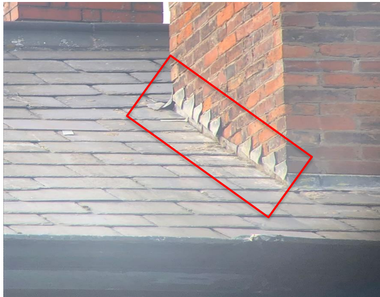
PLATE 12 SHOWING SPLIT ON SOUTH-WESTERN ASPECT OF BUILDING 2
