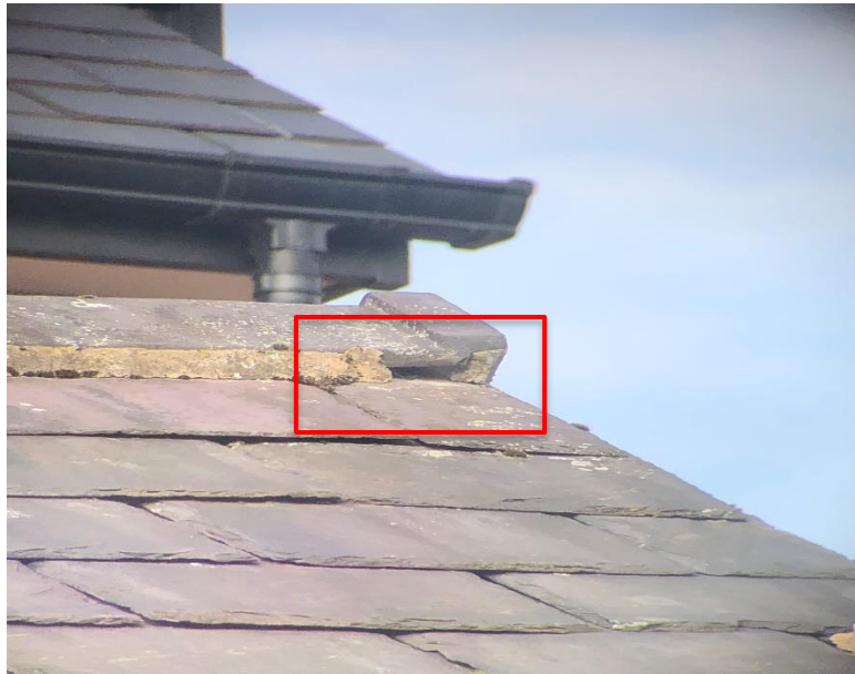
PLATE 10 SHOWING GAP UNDER RIDGE TILE ON BUILDING 2
