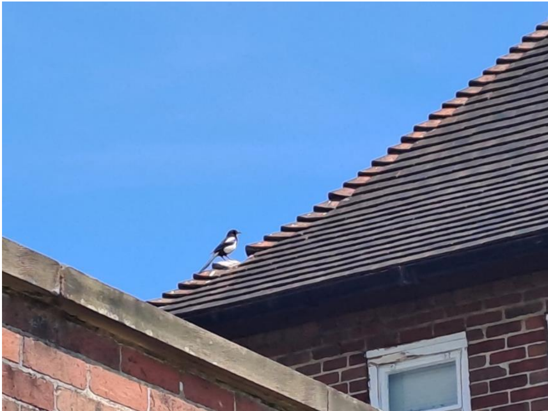
Figure 8: Bird seen looking around the missing tile on the roof
