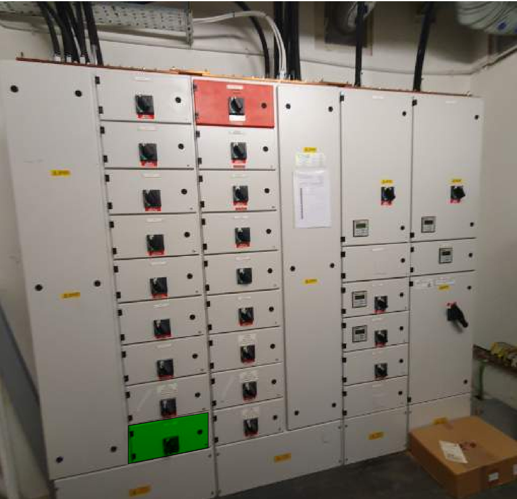
Existing MSP located on ground floor
