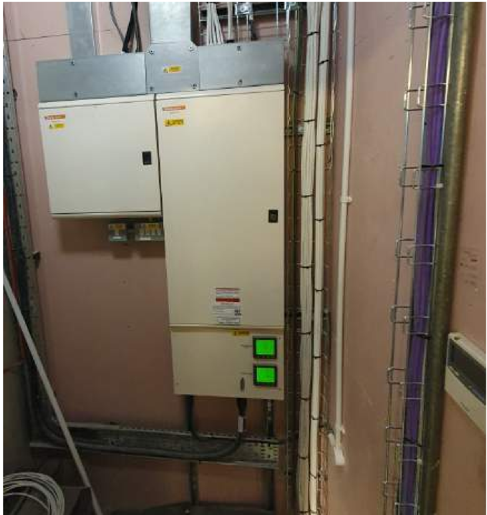
Existing electrical riser located on ground floor
