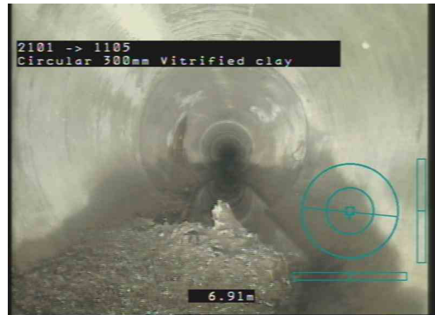
2101X_85f62e90-ec19-4acf-bf4b-1e2a8c9373ba_20191218_23414_189.jpg, 00:04:15, 6.91 m Roots, mass, 15% cross-sectional area loss
