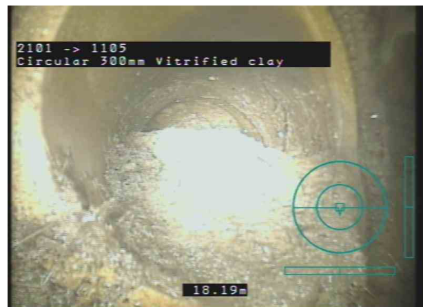
2101X_9fe4bb4f-b1f3-436e-af08-a8c4b31ad9c4_20191218_223833_574.jpg, 00:08:34, 18.19 m Connection defective, connecting pipe is blocked at 10 o'clock, diameter: 150mm
