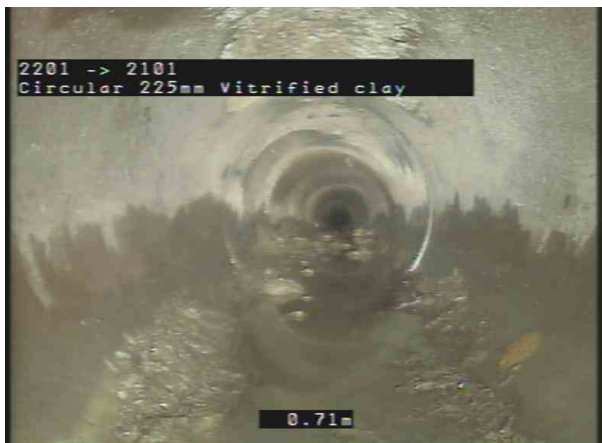
2201X_c32e63fd-8186-41f6-893a-d2db77e82397_20191219_010729_212.jpg, 00:01:27, 0.71 m Settled deposits, fine, 20% cross-sectional area loss, start
