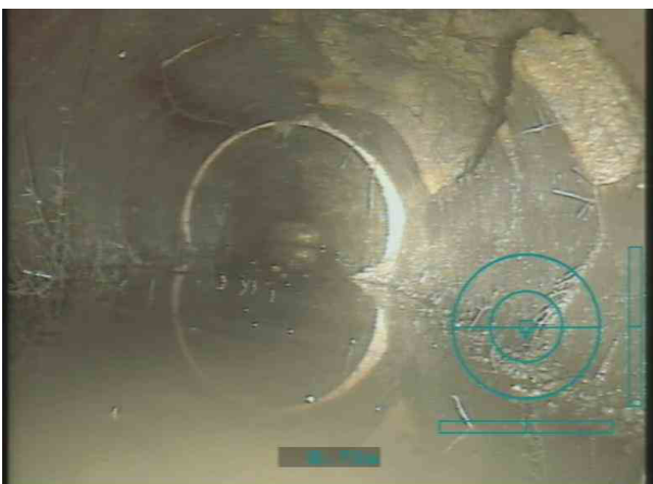
2202X_b55a91f6-0b21-421b-91b1-69a9cd8ff5c3_20191219_202515_216.jpg, 00:02:05, 0.78 m Hole in drain or sewer from 12 o'clock to 2 o'clock
