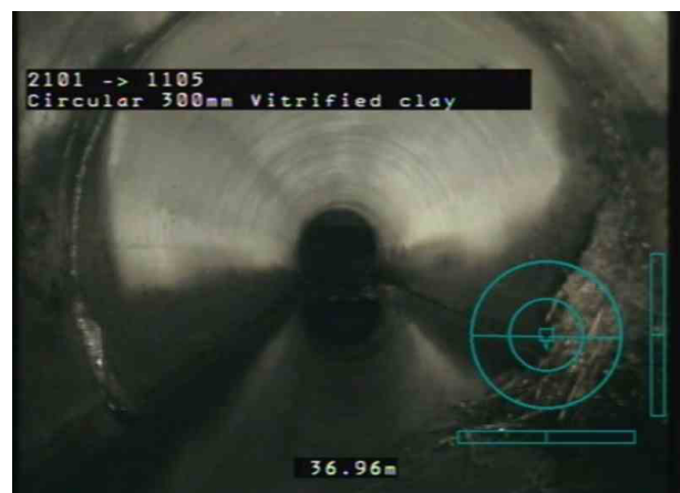
2101X_f35292fb-46e6-4677-ab75-0143026b05cf_20200109_082912_167.jpg, 00:21:47, 36.96 m Roots, fine at joint
