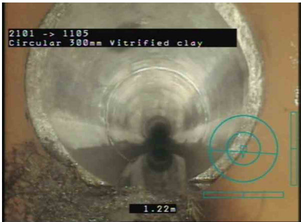
2101X_30833b35-4960-4fdf-87b4-f3dfb2c9e443_20200109_082820_479.jpg, 00:00:55, 1.22 m Roots, fine at joint
