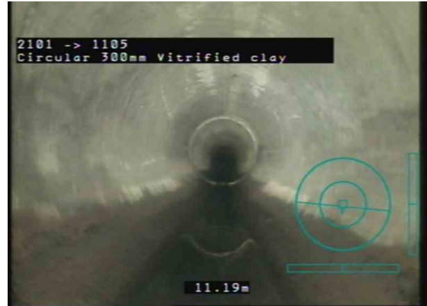
2101X_09cd2e99-ddea-4d5f-996f-3bdd47d71097_20200109_082838_512.jpg, 00:07:11, 11.19 m Roots, fine at joint
