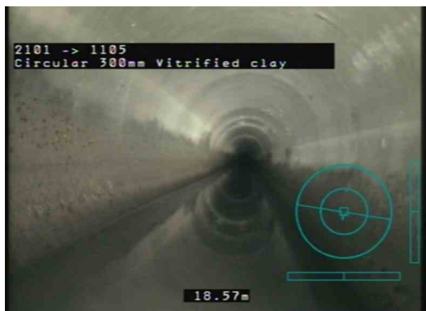
2101X_25967ed6-0ff3-4572-8178-528241cc09ad_20200109_082843_723.jpg, 00:09:05, 18.57 m Roots, mass, 20% cross-sectional area loss, finish
