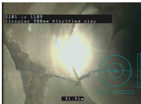
2101X_02ef41d3-5402-44b2-b7ed-a30fa3ddc12a_20191218_224405_257.jpg, 00:14:04, 31.31 m Fractures, multiple from 7 o'clock to 5 o'clock
