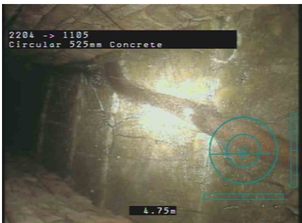
2204X_e5c0bd09-637c-4e47-992c-48e38db5ee44_20191218_220928_242.jpg, 00:07:33, 4.75 m Roots, tap
