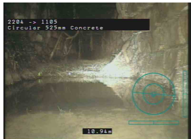
2204X_e5699ea4-ddc3-40d9-9bc6-c4ec7cdbcfff_20191218_221433_046.jpg, 00:11:40, 10.94 m Dropped invert, gap: 300mm from 5 o'clock to 7 o'clock
