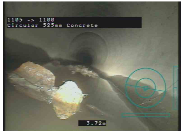
1105X_3996a299-04be-4035-bd44-1a8446a09a23_20191218_213009_115.jpg, 00:01:47, 3.72 m Settled deposits, coarse, 15% cross-sectional area loss, start
