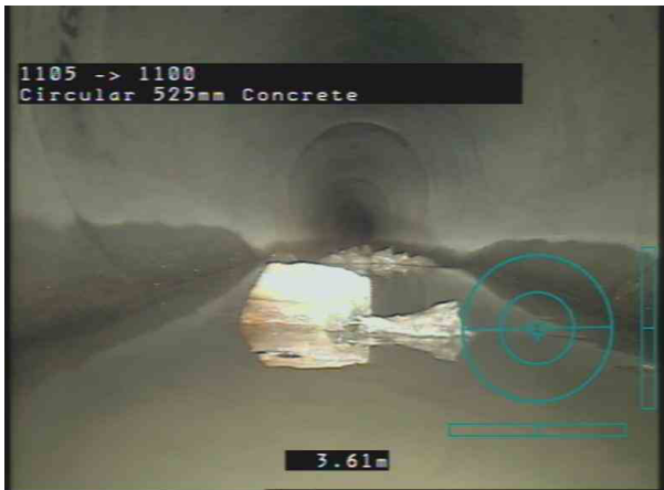
1105X_e58a2646-c911-4907-860f-02568851a08a_20191218_213155_710.jpg, 00:03:32, 3.61 m Other obstacles, brick or masonry in invert from 6 o'clock to 7 o'clock, 10% cross-sectional area loss
