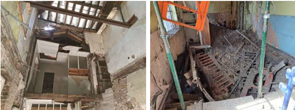
Images of collapse
