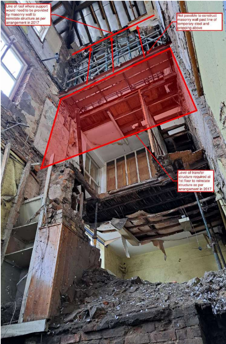
Renaissance collapse annotation
