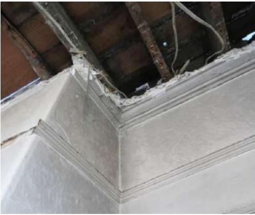
An area of partially surviving cornice to the alcove and small area of removed picture rail.
