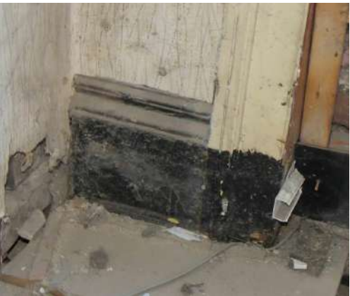
A small example of surviving original timber skirting to be used as a template for other areas.
