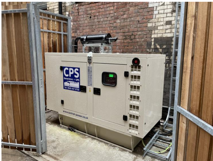
Figure 2 Photograph of generator installed at 40-46 Princess Street
