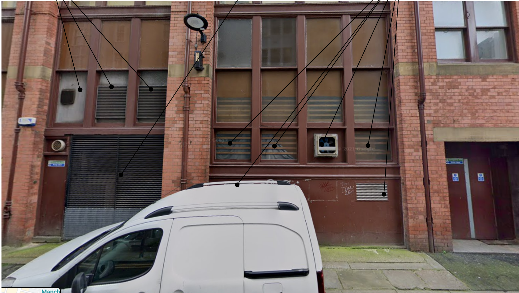
Image 1 External Ground Floor Elevation Facing Quay Street - Existing Supply & Extract Louvre Locations
