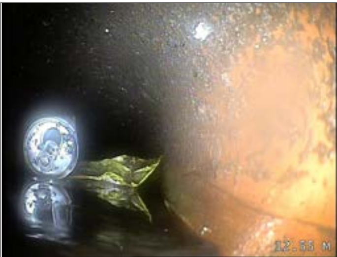
Other settled deposits 25% cross-sectional area loss - Remark: DEBRIS
