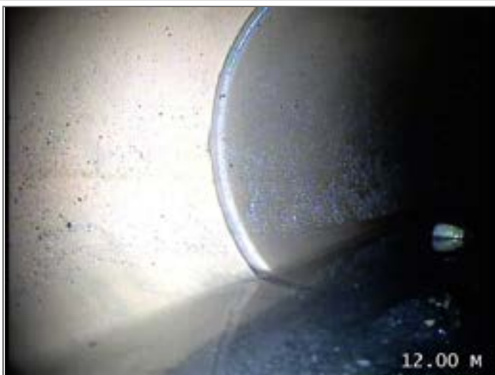
Line of drain/sewer deviates right
