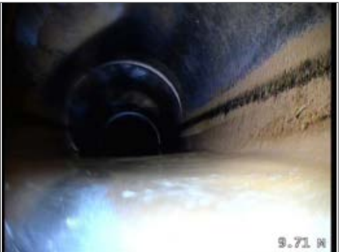
Water level 10% height/diameter - Remark: DIP IN PIPE
