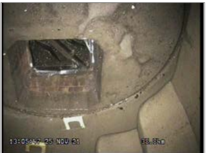
Finish node type, manhole, reference MH S13
