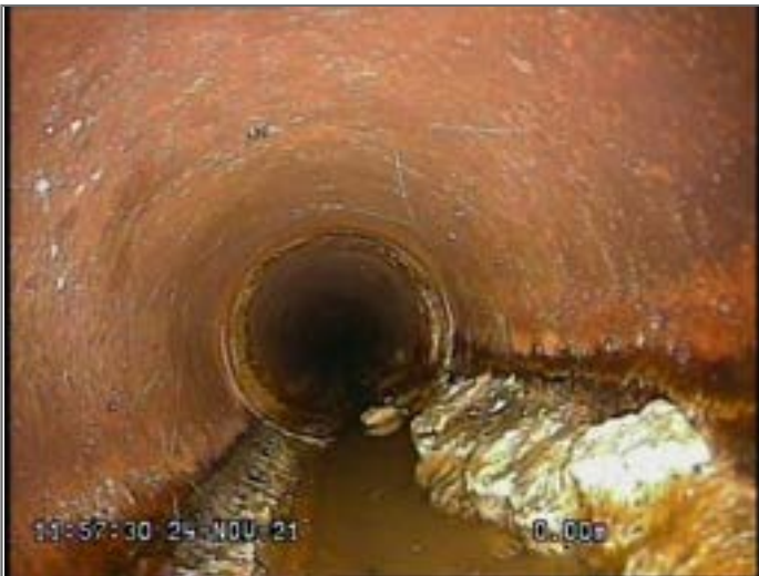
Attached deposits, fouling at 4 o'clock 10% cross-sectional area loss
