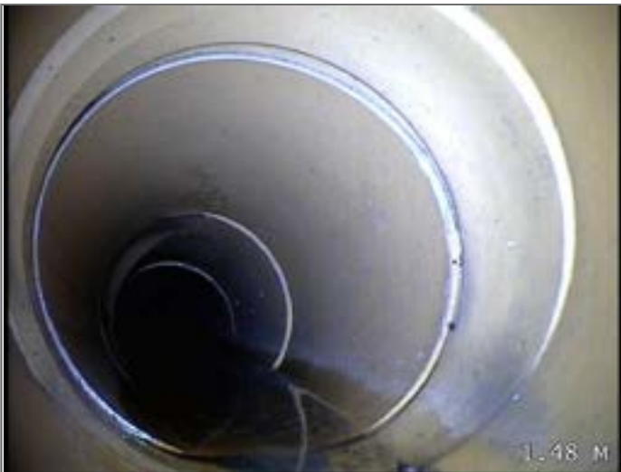
Line of drain/sewer deviates left
