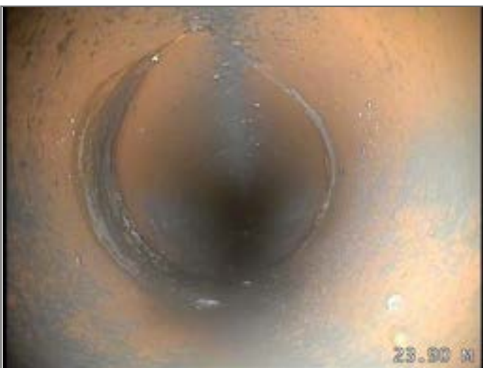
Fracture circumferential from 12 to 12 o'clock
