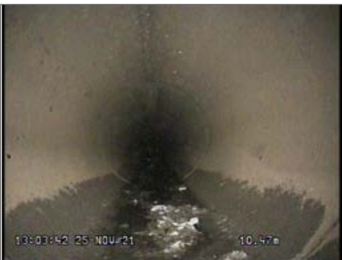
Settled deposits fine 5% cross-sectional area loss
