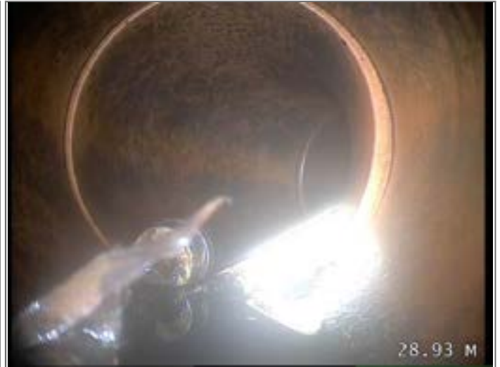
Line of drain/sewer deviates right
