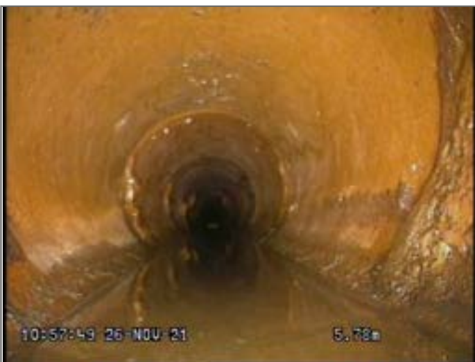
Settled deposits fine 5% cross-sectional area loss
