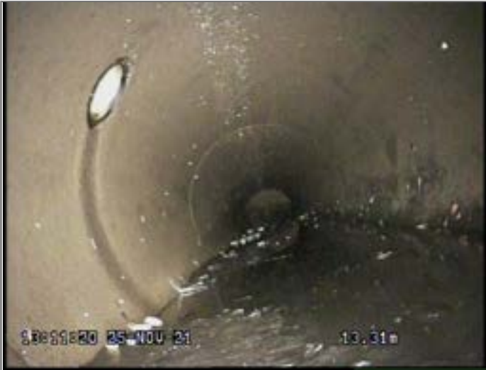
Settled deposits fine 10% cross-sectional area loss, Finished
