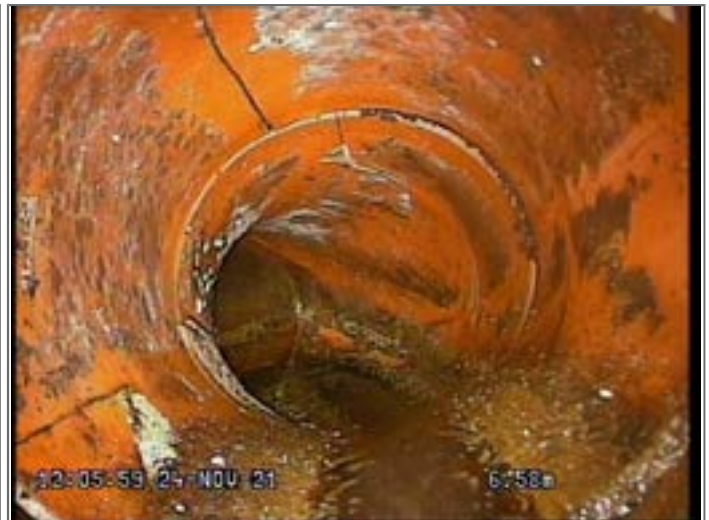
Line of drain/sewer deviates down
