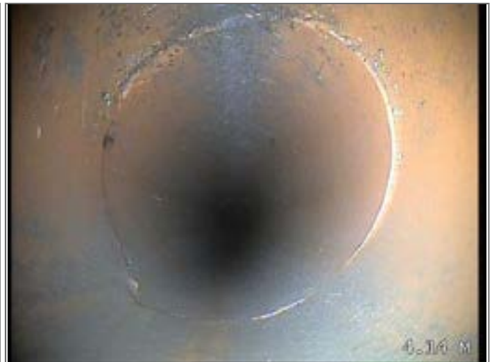
Crack circumferential from 12 to 12 o'clock
