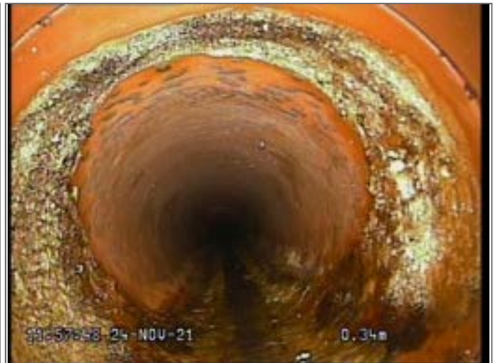
Attached deposits, encrustation from 7 to 5 o'clock 5% cross-sectional area loss
