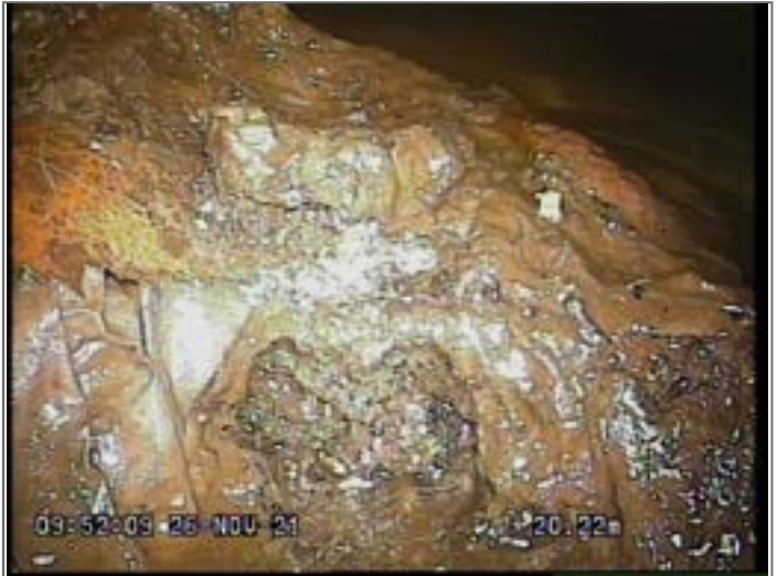
Survey abandoned - Remark: OBSTRUCTION - UNABLE TO PASS DUE TO FOUL AND COARSE DEPOSITS
