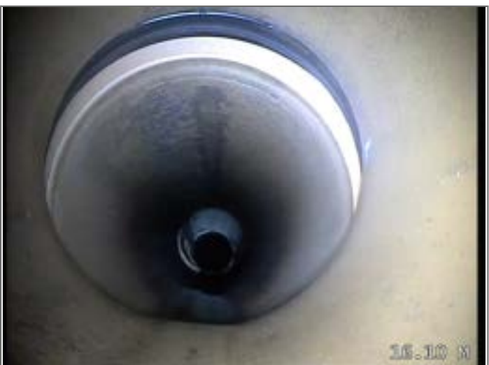
Joint displaced medium
