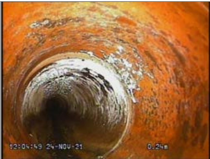
Line of drain/sewer deviates left
