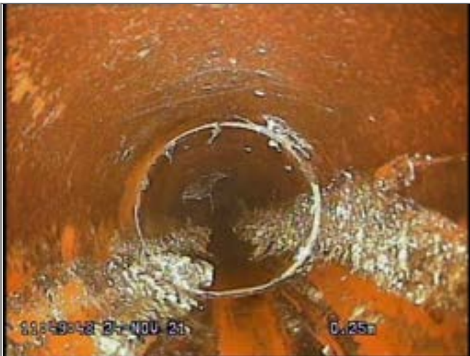
Attached deposits, fouling at 7 o'clock 5% cross-sectional area loss
