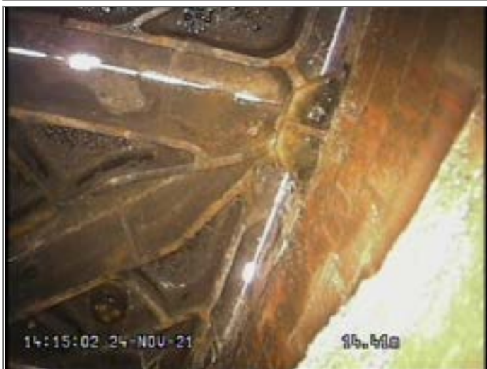
Finish node type, manhole, reference MH S8
