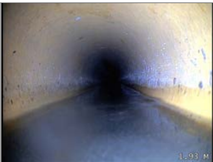
Settled deposits fine 5% cross-sectional area loss
