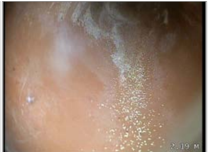
Line of drain/sewer deviates up
