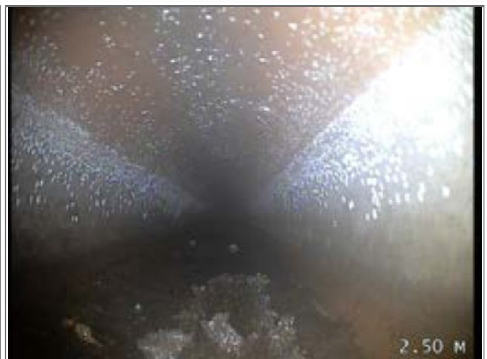
Settled deposits fine 5% cross-sectional area loss
