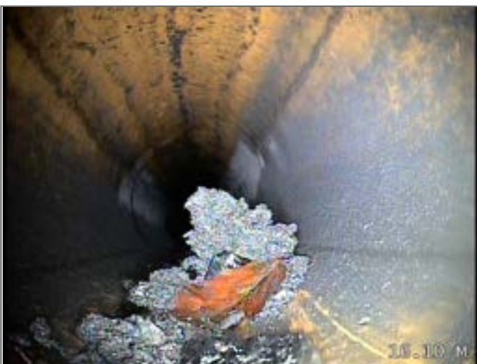
Settled deposits fine 5% cross-sectional area loss
