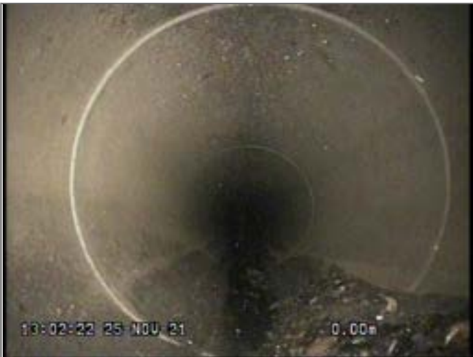
Settled deposits fine 5% cross-sectional area loss
