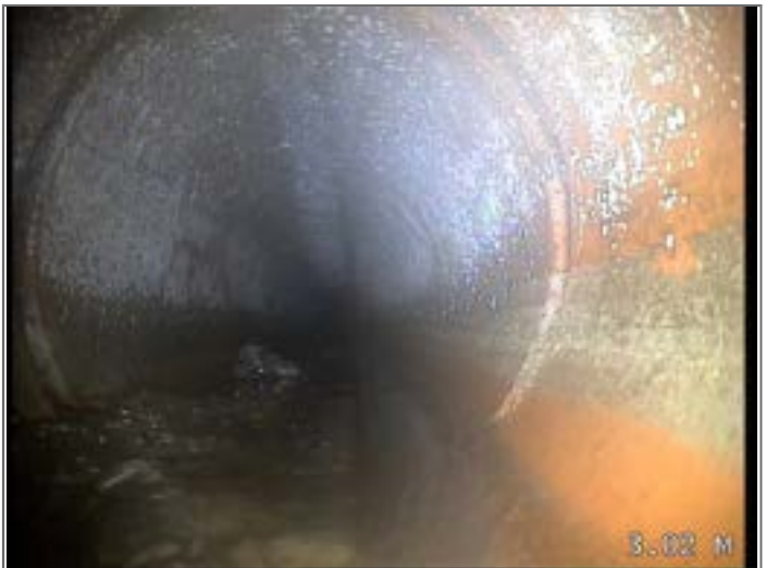
Settled deposits fine 5% cross-sectional area loss
