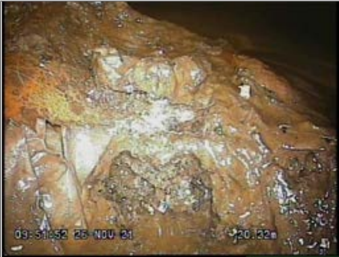
Settled deposits coarse 15% cross-sectional area loss
