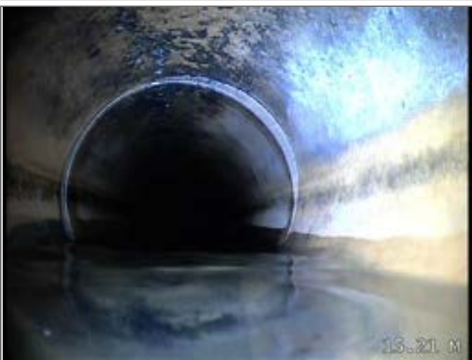
Water level 10% height/diameter - Remark: DIP ON PIPE
