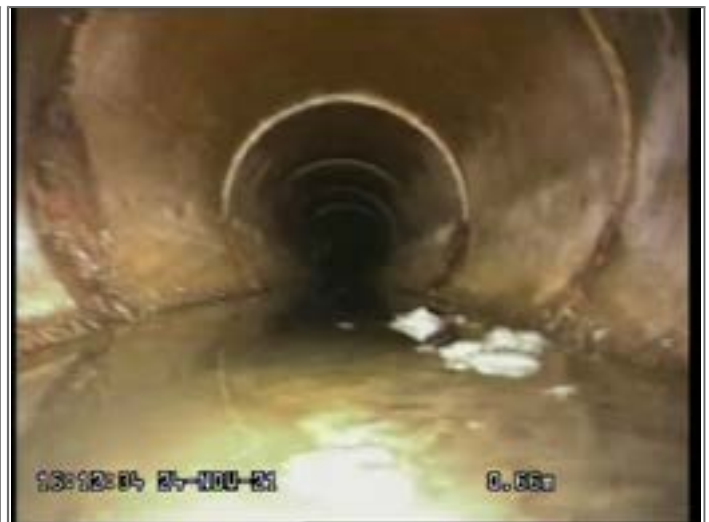
Attached deposits, encrustation from 7 to 10 o'clock 5% cross-sectional area loss - Remark: THIS IS A CONTINUOUS DEFECT UPSTREAM TO UU 1304 , Start
