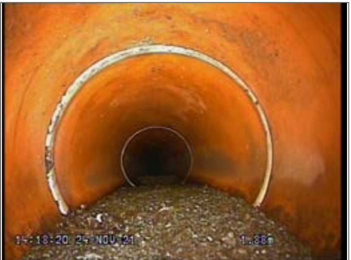
Settled deposits fine 20% cross-sectional area loss
