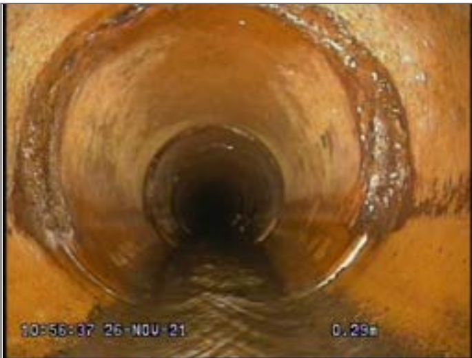
Attached deposits, encrustation from 8 to 4 o'clock 5% cross-sectional area loss
