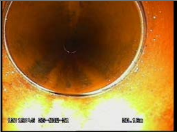
Finish node type, gully, reference UNABLE TO PASS DUE TO CHANGE OF PIPE SIZE - REST BEND IN VIEW A FEW METERS U/S
