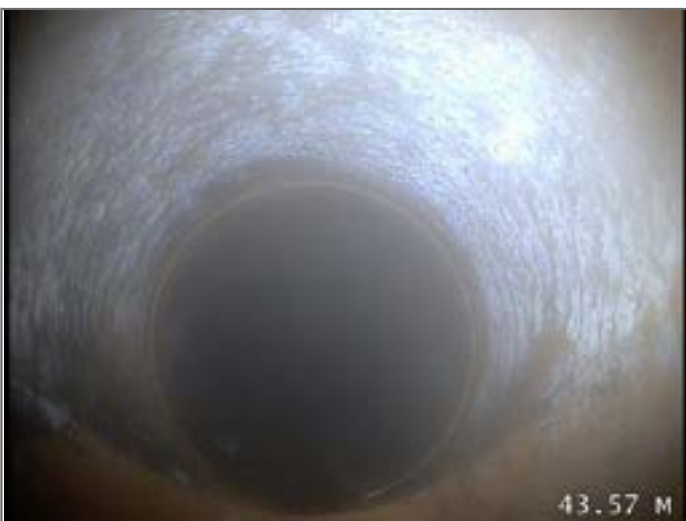
Line of drain/sewer deviates down - Remark: BACK DROP
