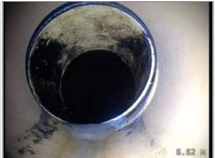
Joint displaced medium
