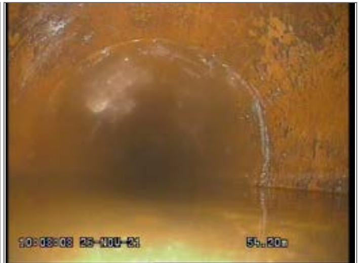
Survey abandoned - Remark: OBSTRUCTION UNABLE TO PASS DUE TO ATTACHED DEPOSITS UNDER WATER
