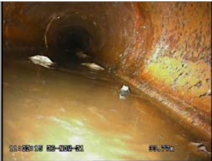
Settled deposits fine 10% cross-sectional area loss
