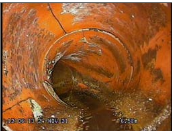
Fracture multiple from 12 to 12 o'clock
