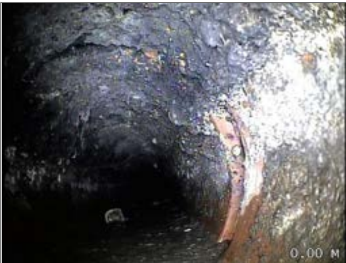
Settled deposits fine 10% cross-sectional area loss
