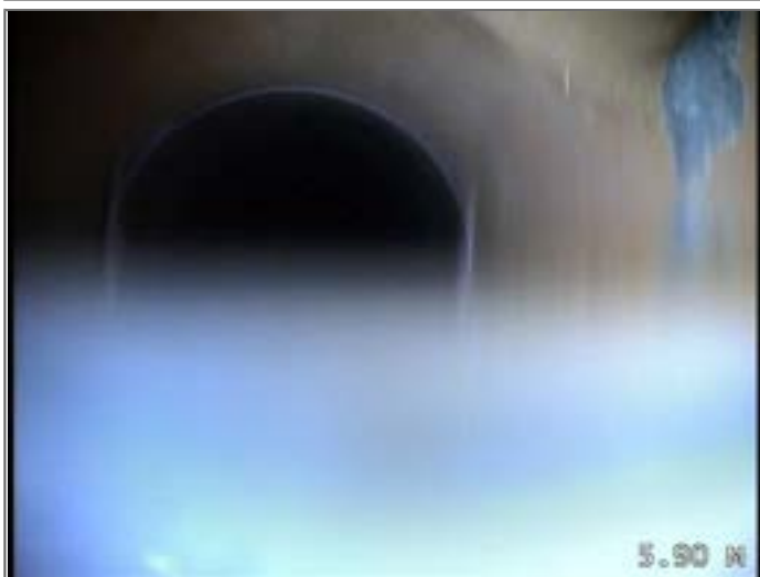
Water level 10% height/diameter - Remark: DIP IN PIPE
