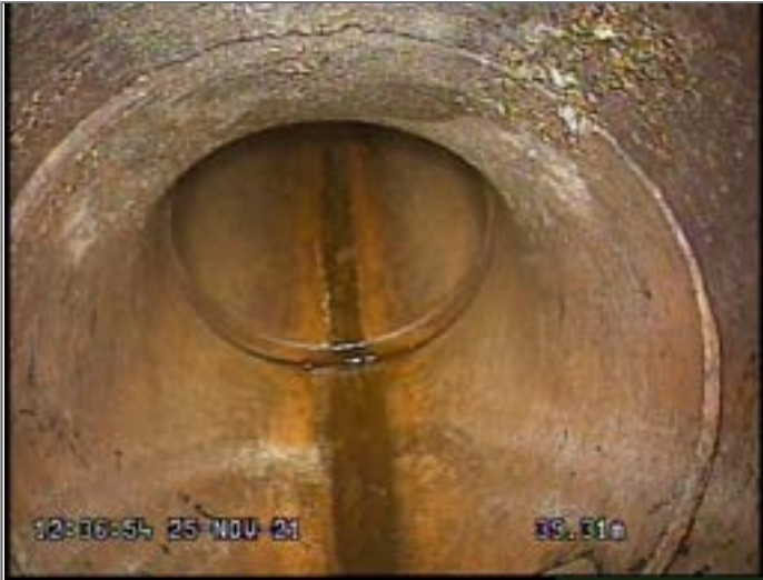
Line of drain/sewer deviates up
