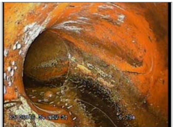
Line of drain/sewer deviates left
