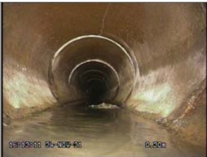
Crack longitudinal at 12 o'clock
