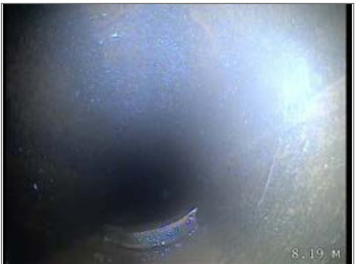
Settled deposits coarse 5% cross-sectional area loss - Remark: PIECE OF PIPE
