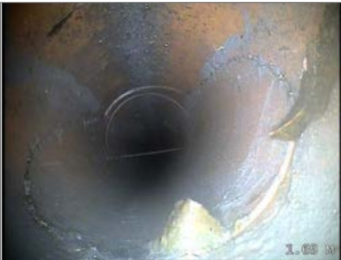
Crack spiral from 1 to 9 o'clock
