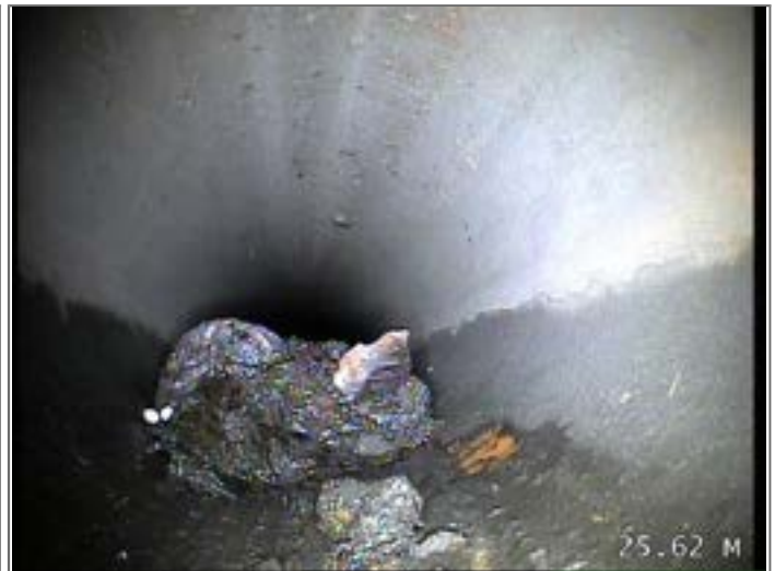
Settled deposits fine 10% cross-sectional area loss
