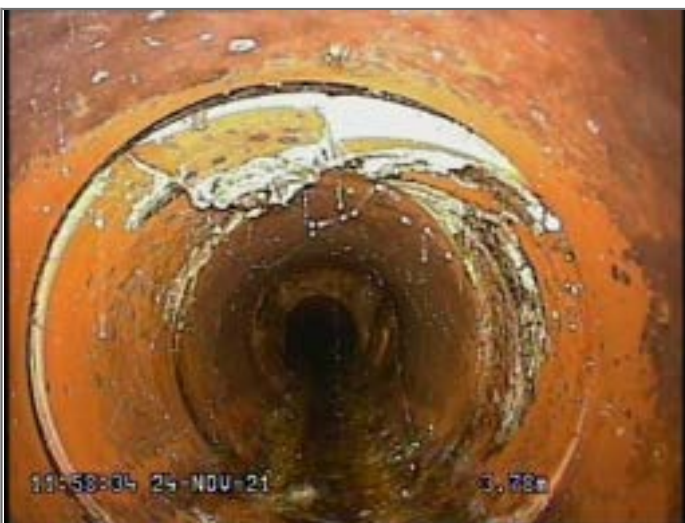
Fracture multiple from 10 to 2 o'clock
