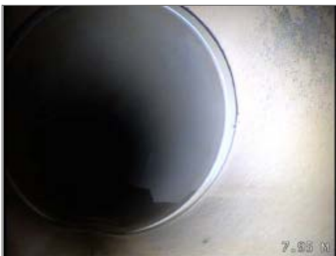
Line of drain/sewer deviates left
