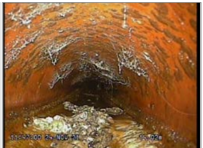
Attached deposits, fouling from 5 to 7 o'clock 10% cross-sectional area loss
