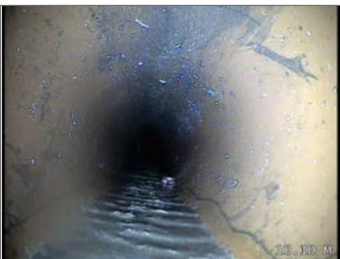
Settled deposits fine 5% cross-sectional area loss
