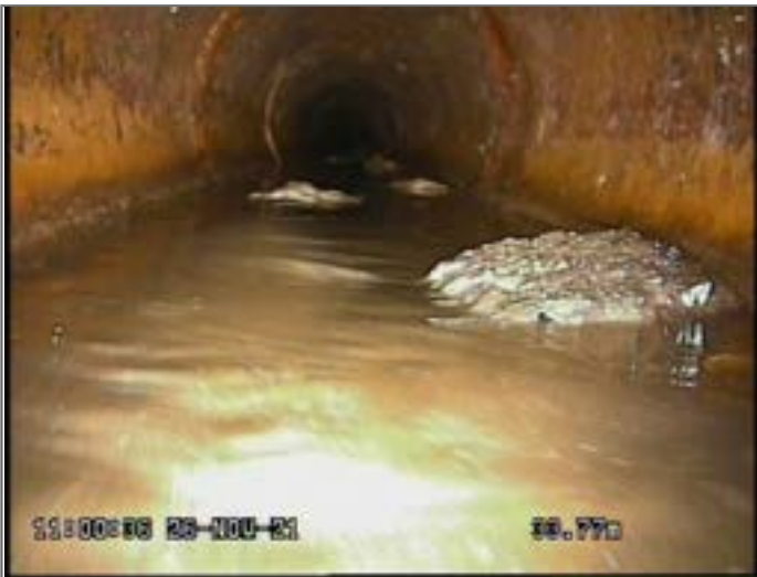
Settled deposits coarse 5% cross-sectional area loss
