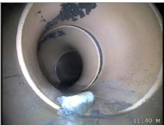
Line of drain/sewer deviates left
