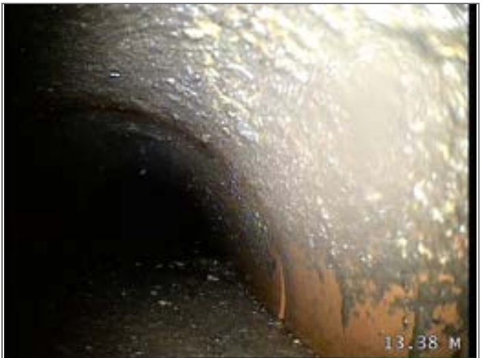
Settled deposits fine 25% cross-sectional area loss
