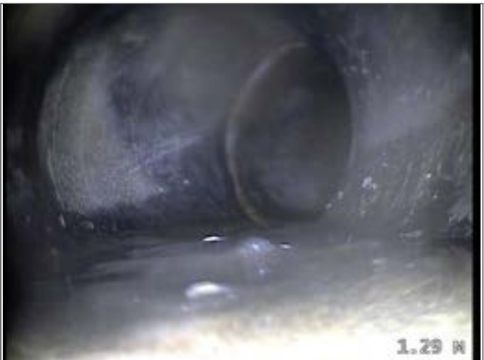
Line of drain/sewer deviates right
