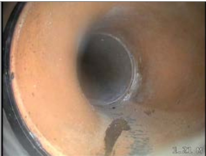
Line of drain/sewer deviates left
