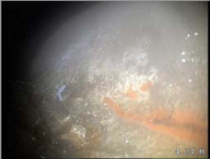
Finish node type, manhole, reference MH S1
