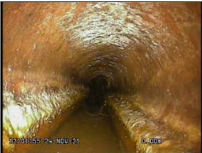
Attached deposits, fouling at 5 o'clock 5% cross-sectional area loss
