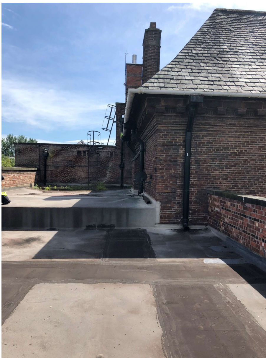
Photo 6: View of roofs 2 & 3 towards roof 4 parapets and hooped ladder. Note RWPs discharging onto flat, altered to suit raised flat roof level.
