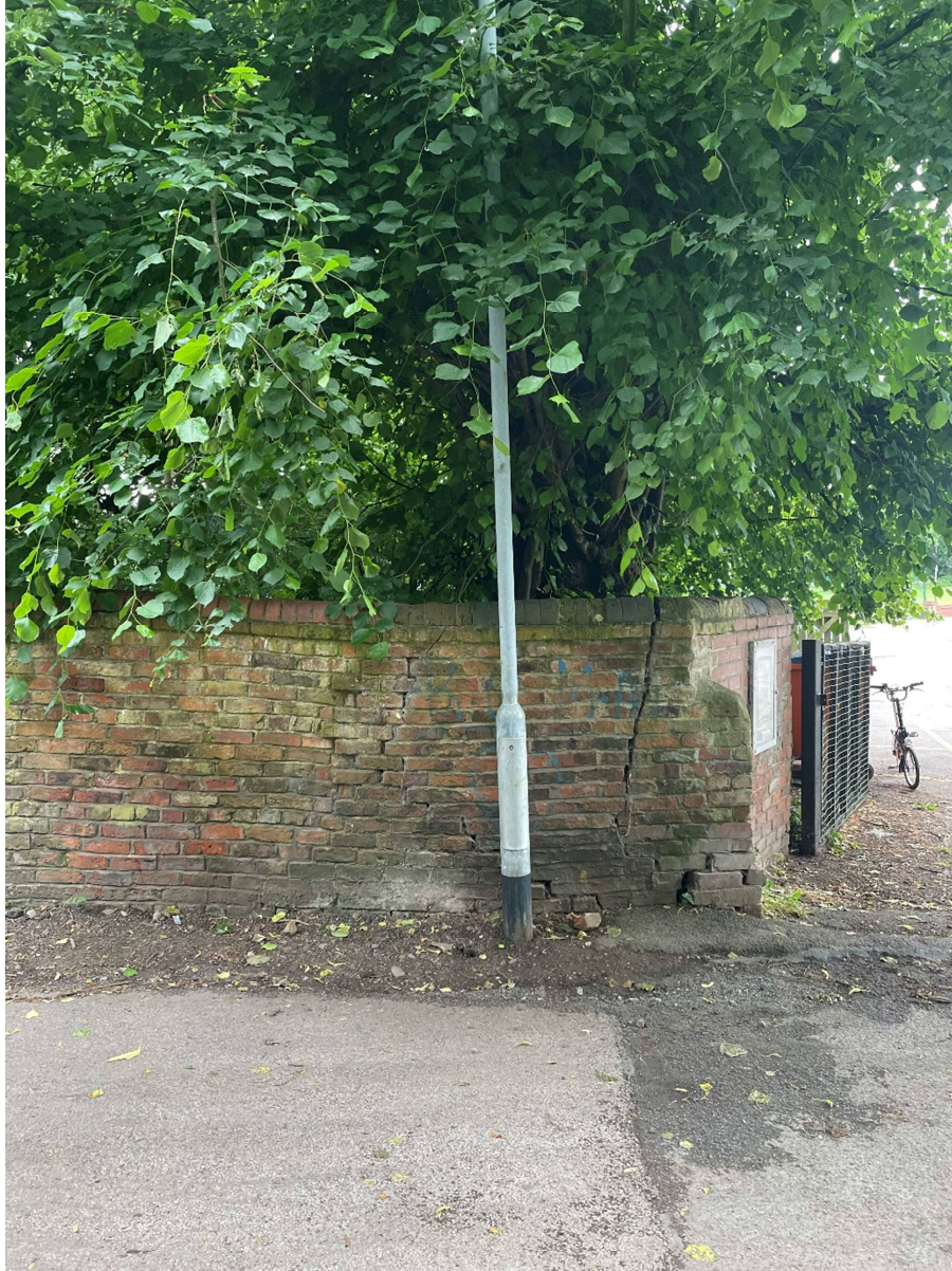
Photo 1. Damaged wall section along Ford Lane
