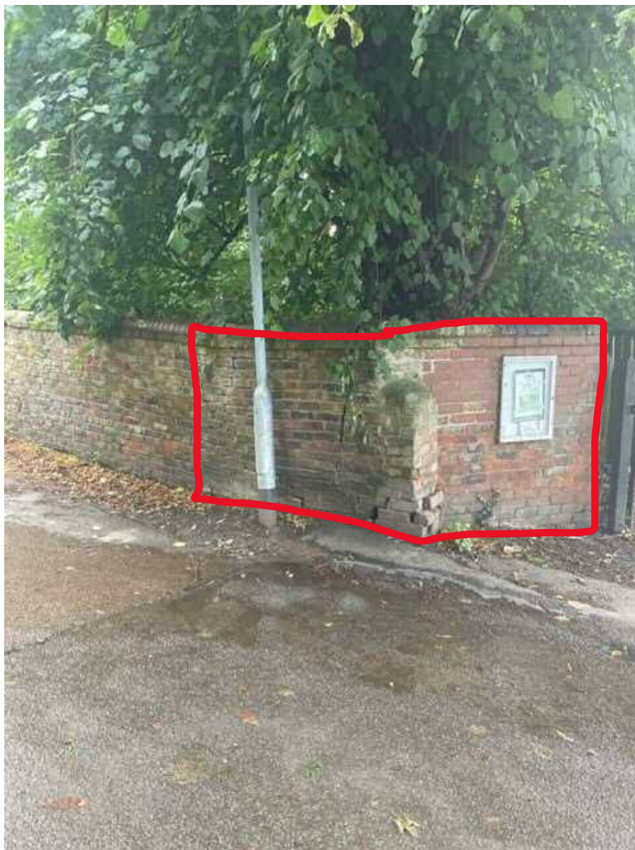
Photo 4. Red outline shows the proposed wall section to be removed
