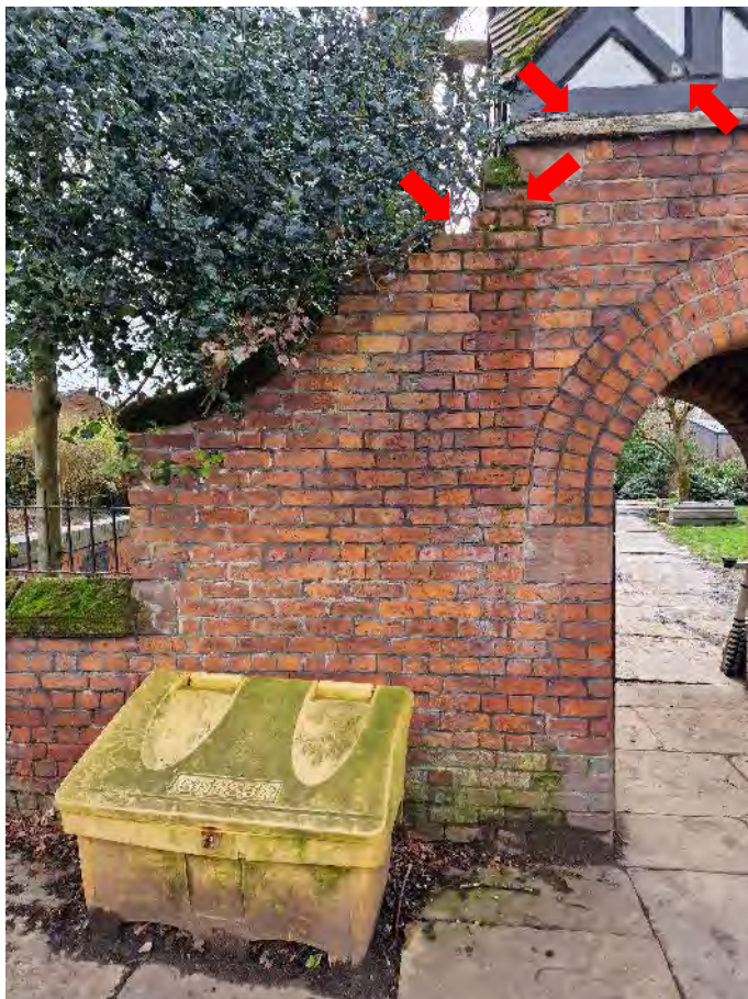
Figure 10: Bell Tower Turret, view from north-east. Extensive timber decay is present and visible. Existing coping stone is missing, and water ingress is visible on the masonry wall. Existing trees' branch has caused damaged to the building fabric.
