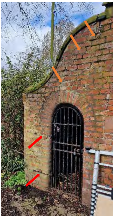
Figure 6: Orange colour arrows on top show the diagonal cracks on top of the door arch. Corrosion of metal wall anchors (red colour arrows) have caused the expansion of the joint and pushed the bricks up. The metal gate is not operational due to structural movement of the masonry wall. Internal timber barded door was left open and not operation, and it resulted in the chamber to be filled with debris, leaves and rubbish.
