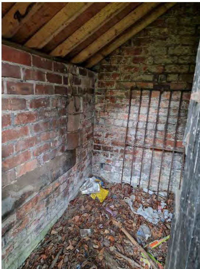
Figure 12: View to the inside of the Lych Gate's access chamber. Leaves and debris accumulated inside the space as the internal timber-boarded door is not operational and left open.
