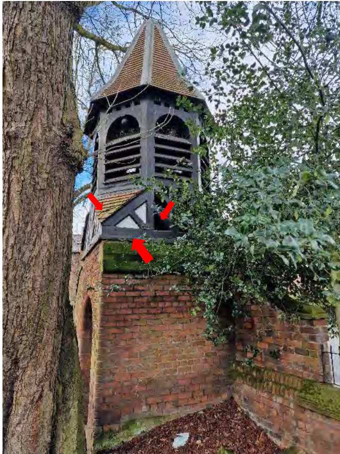
Figure 9: Bell Tower Turret, view from south-east. Extensive timber decay is present and visible. Roof tiles and infill panels are missing. The tree's branches caused damaged to the building fabric.
