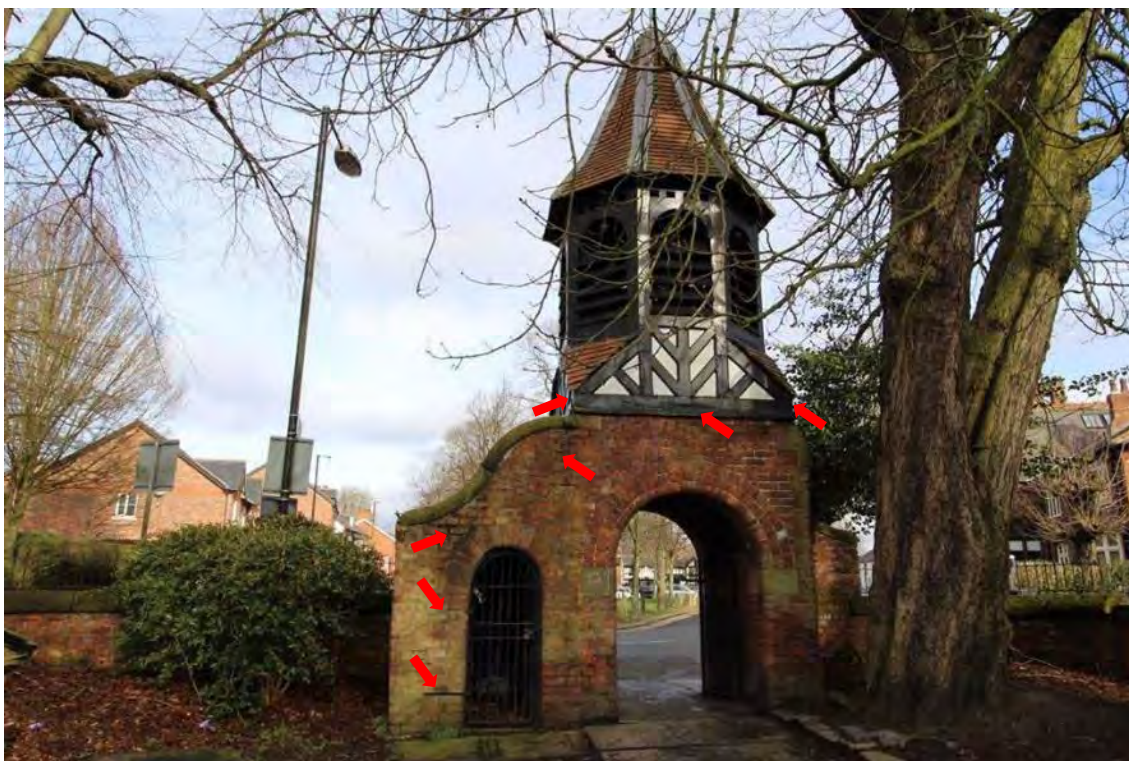
Figure 5: Lych Gate, South elevation. Water stain is visible on the masonry wall surface due lack of water disposal system from the small triangular shape roof. Pointing to the masonry in poor condition due to water run off on the wall surface. Significant timber decays (dry/wet rot) identified. Diagonal cracks were identified which caused by the corroded metal anchors.
