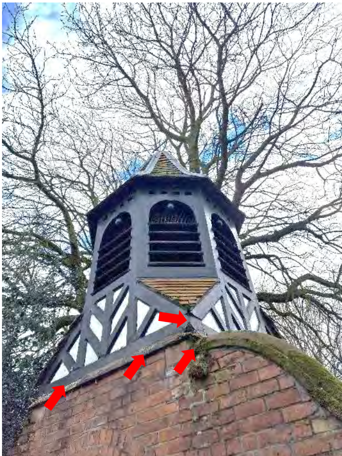
Figure 8: Bell Tower Turret, view from north-west. Extensive timber decay is present and visible (see red colour arrows). Absence of appropriate water collection/disposal from the small triangular shape tiled roof resulted in excessive water run-off and subsequently caused extensive decay and rot to the timber and building fabric.
