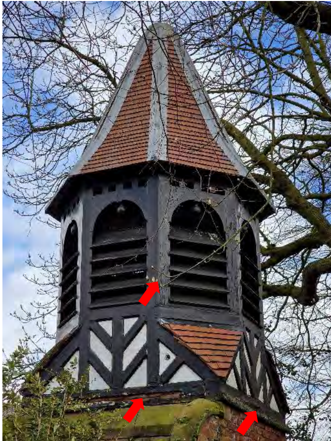
Figure 7: Bell Tower Turret, view from south -west. Extensive timber decay is present and visible on multiple places. The infill panels are built of plywood and painted in white which need to be removed and appropriate infill panels to be placed (Lath & Lime render)
