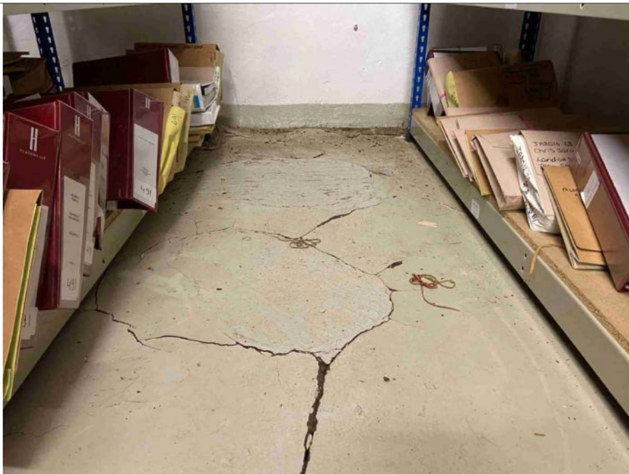
38: Saturated and delaminated floor screed to basement store room 6
