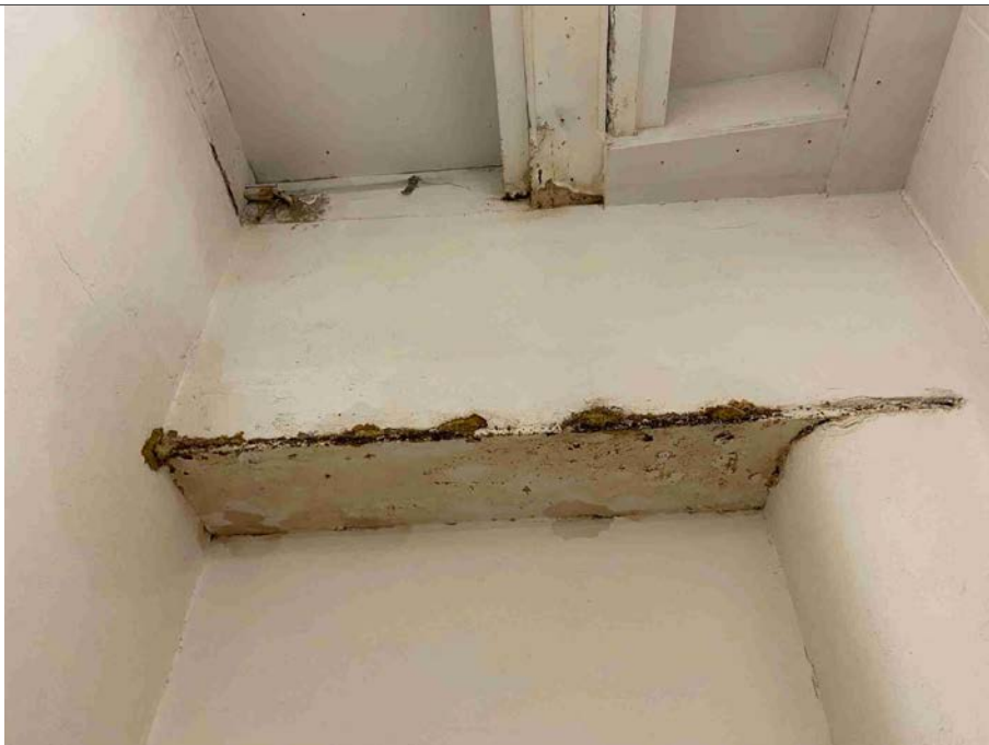
36: Typical water ingress at basement at high level Peter Street elevation
