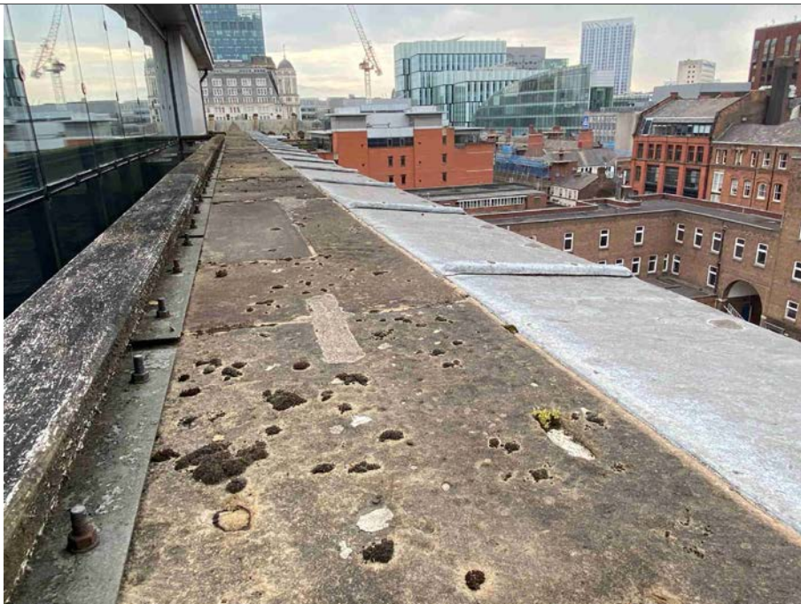
28: Stone coping to Bootle Street parapet (note partial lead capping)
