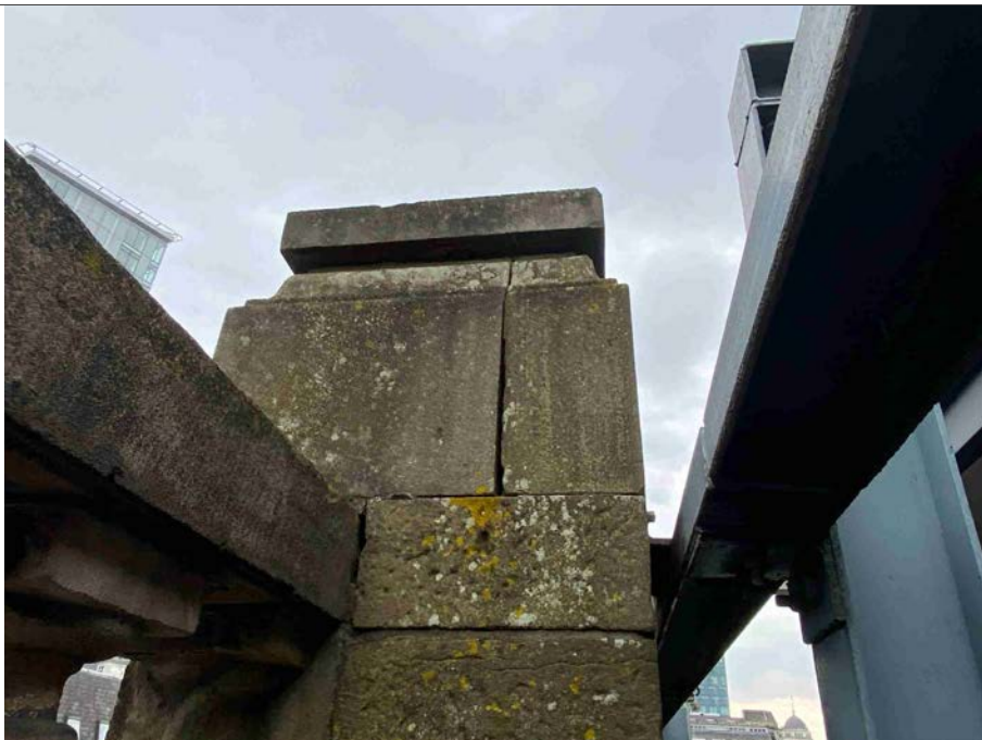
26: Example open joints to parapet level stonework (note steel restraint ties)
