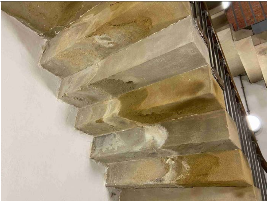
32: Salt staining and efflorescence to rear stairs between ground and lower ground floor
