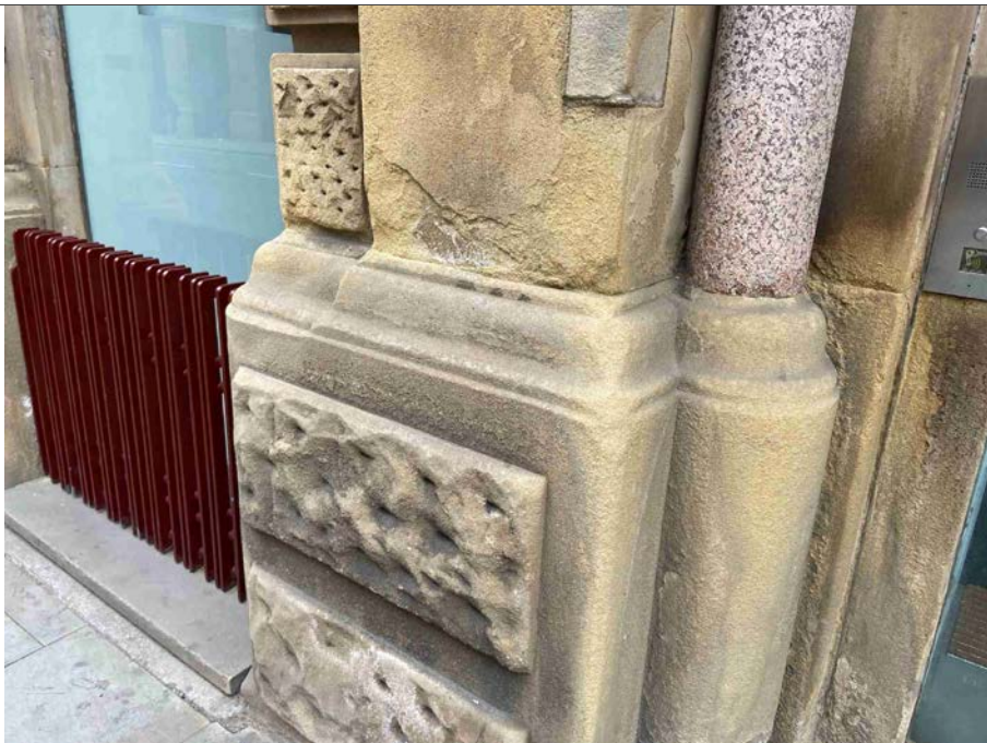
40: Example historic erosion to stonework at street level.
