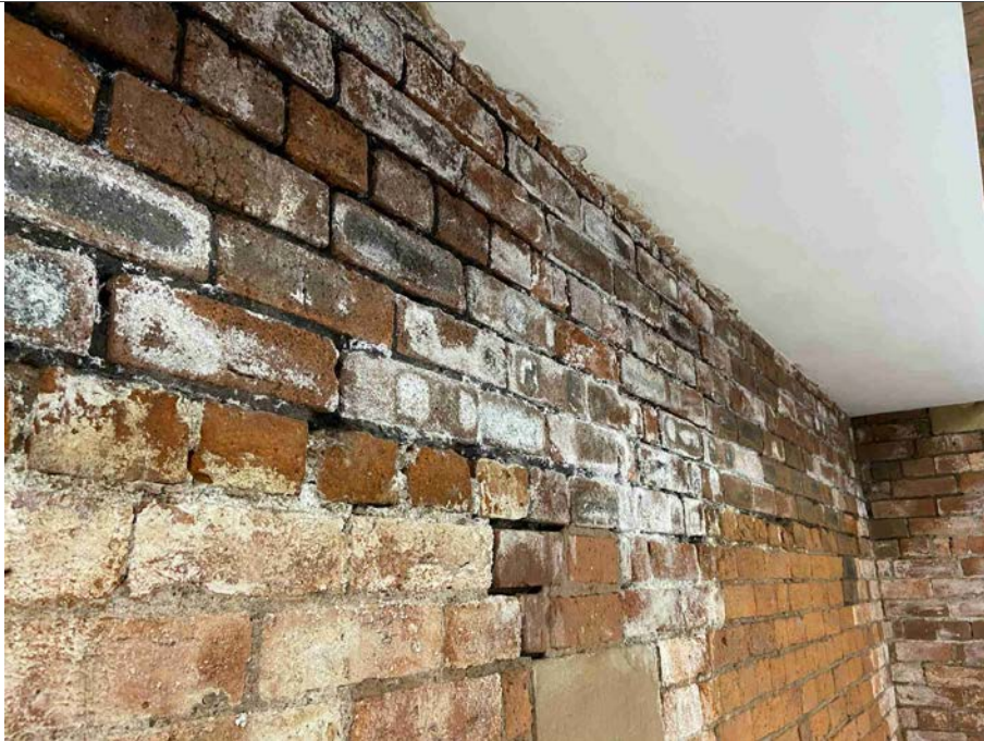
31: Salt staining and efflorescence to eaves level brickwork rear staircase
