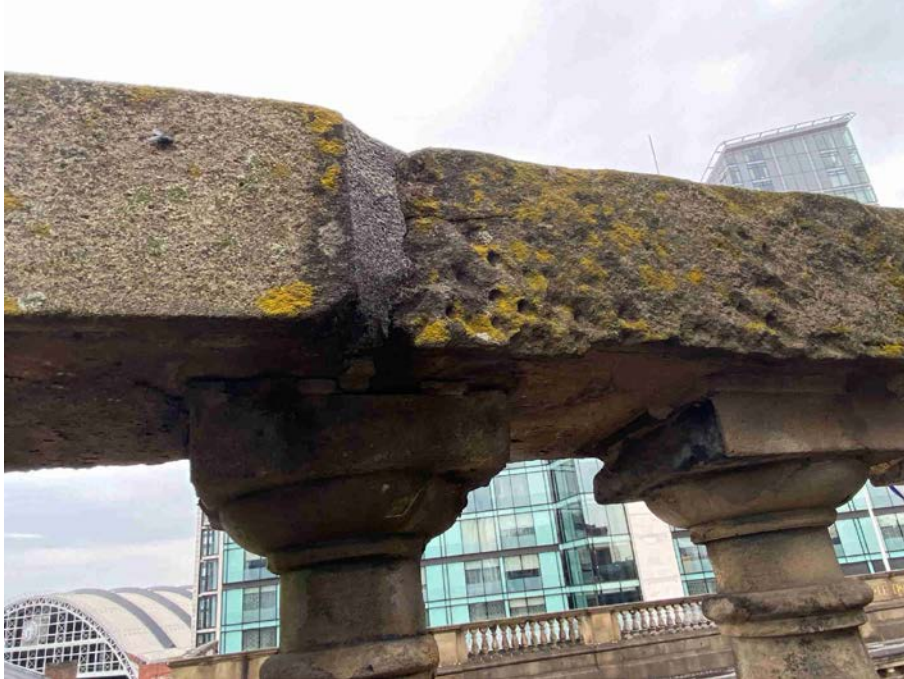
23: Example of historic displacement of stonework prior to restraint ties
