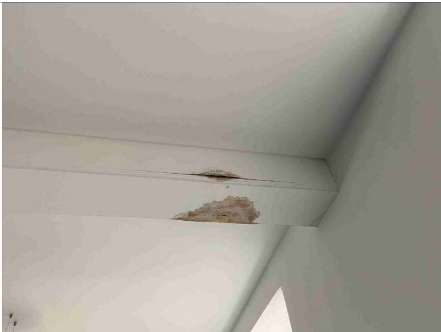
30: Internal water ingress to fourth floor office via fifth floor balcony walkway
