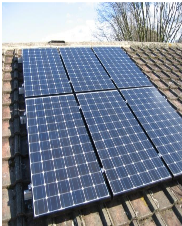
Figure 4 - Photovoltaic array on a pitched roof
