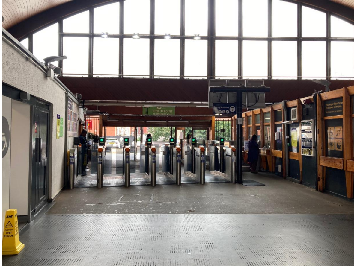
Ticket gate line ATG's as existing
