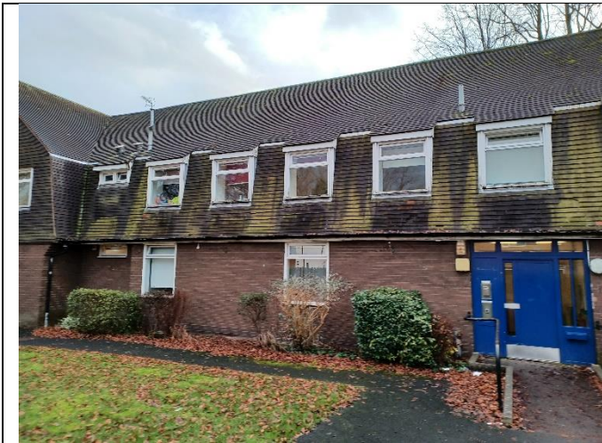
Windows & doors to be renewed
