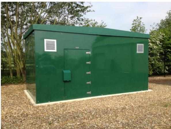
Figure 1: Security Rated CRP Housing
