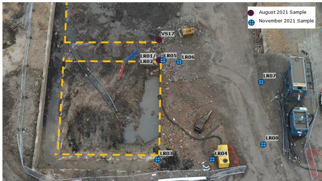
Figure 3: Approximate sampling locations in the Basement Area (LR03 to LR08) extending away from the unexpected contamination encountered in August 2021. Aerial image taken facing the north-east. Dashed line depicts the concrete slab edges.
