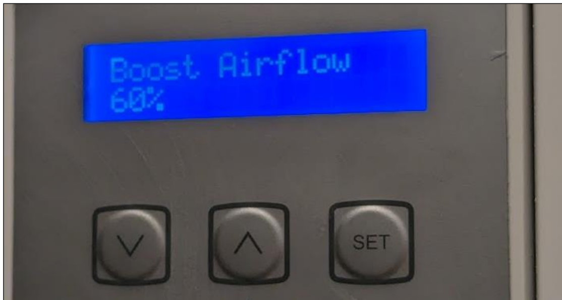
Photo taken on-site of one of the MVHR units in operation.
