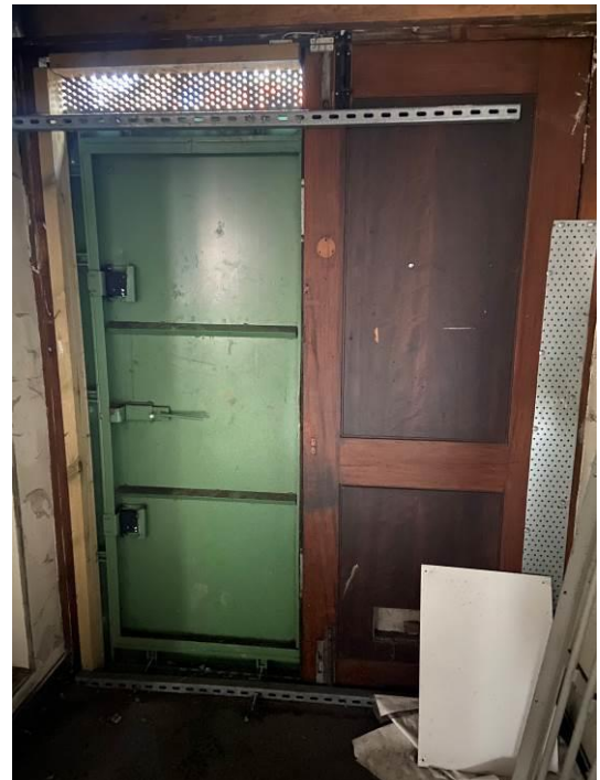
Figure 17: Interior side of primary entrance from the corner of Piccadilly and Chatham Street. Temporary measures have been installed to improve the security of the building.
