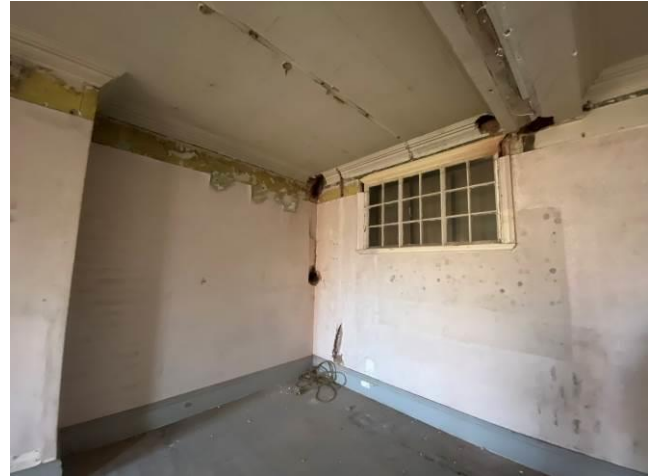
Figure 31: Upper level room. Removal of suspended ceiling has caused some damage to historic cornice.
