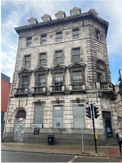
Figure 14: Primary elevation of the listed building to Piccadilly. Temporary grilles have been placed over window openings to protect the building from further damage and deterioration.
