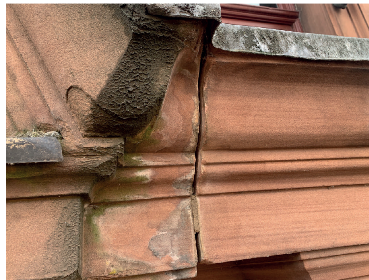
Examples of failing pointing.
