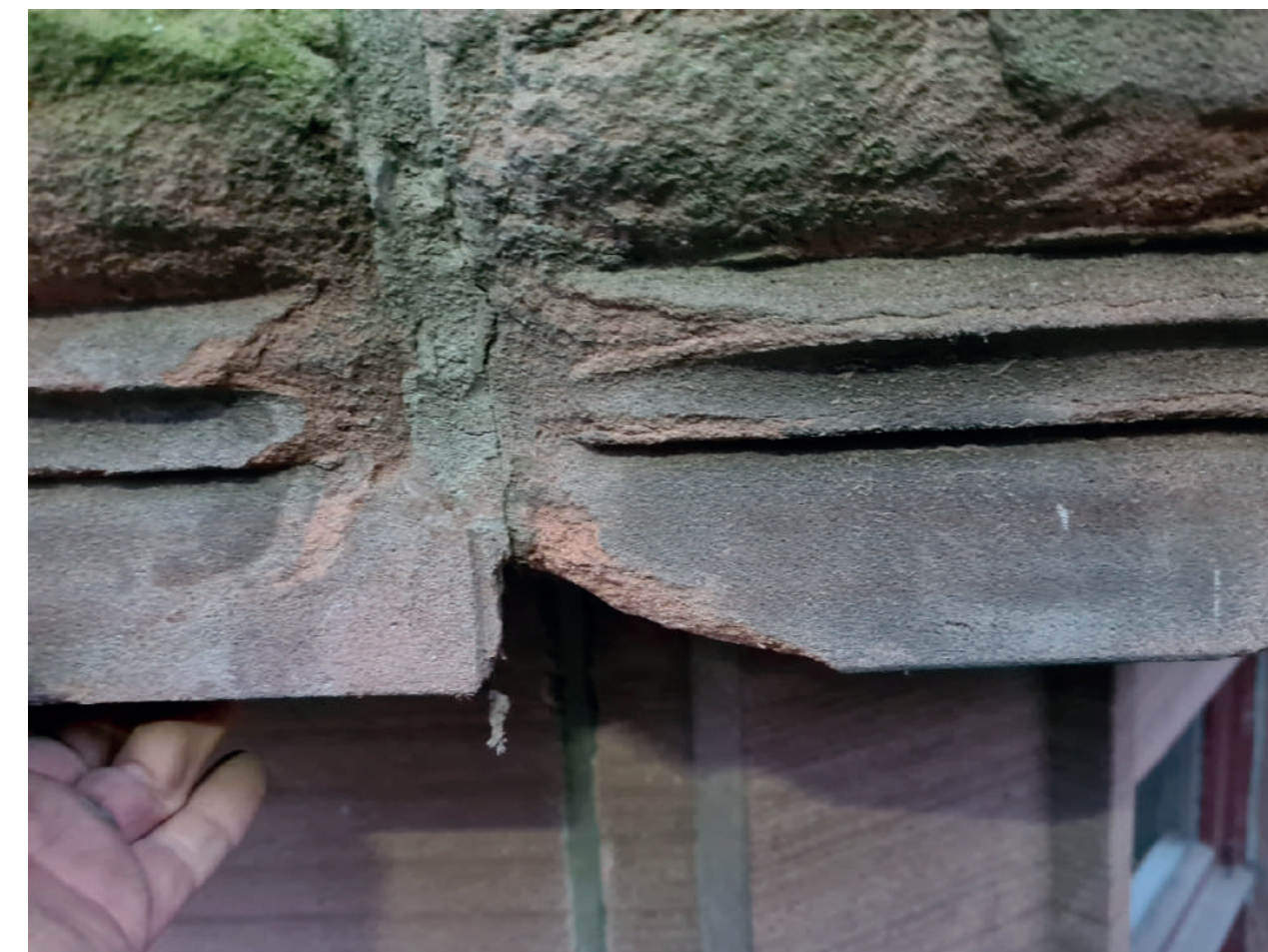
B01, 3 - Stone broken away. Stone indent proposed, followed by repointing.
