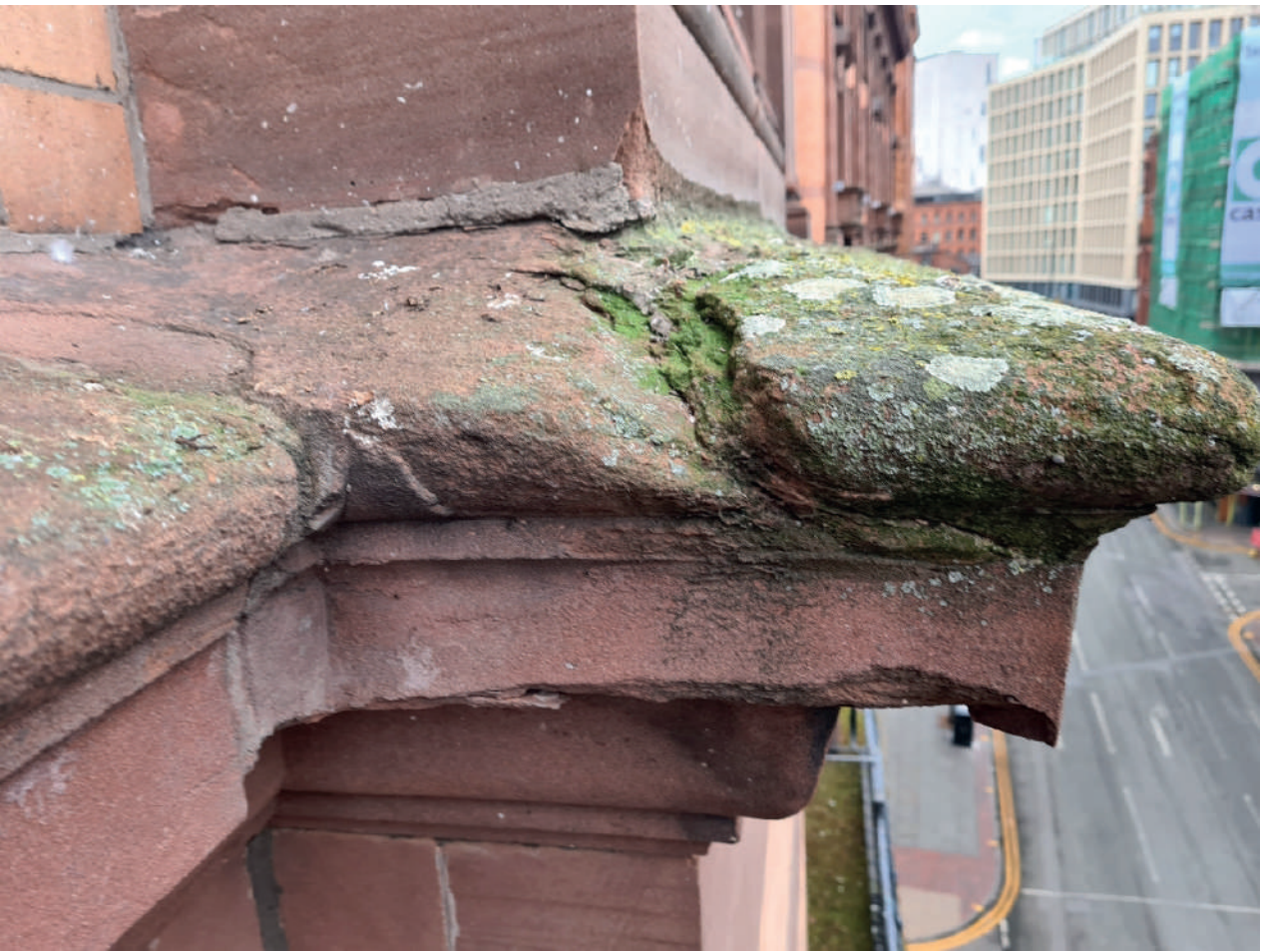
Location A02,5 - stone at risk of detaching.
