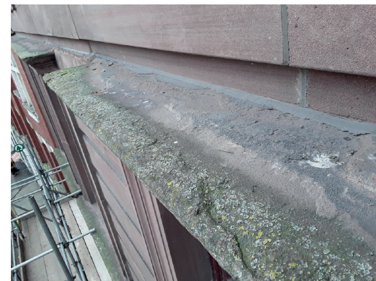
Example of potential atmospheric dirt crust to be cleaned off - pending close inspection.
