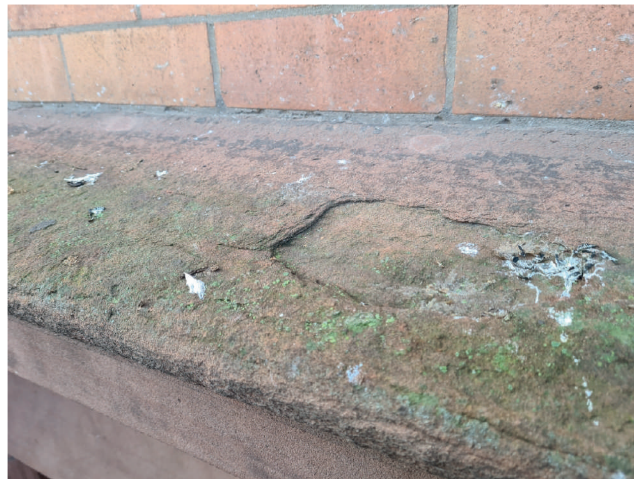
A07,5 - stone surface delaminating, risking accelerated freeze/thaw erosion. Stone indent proposed.
