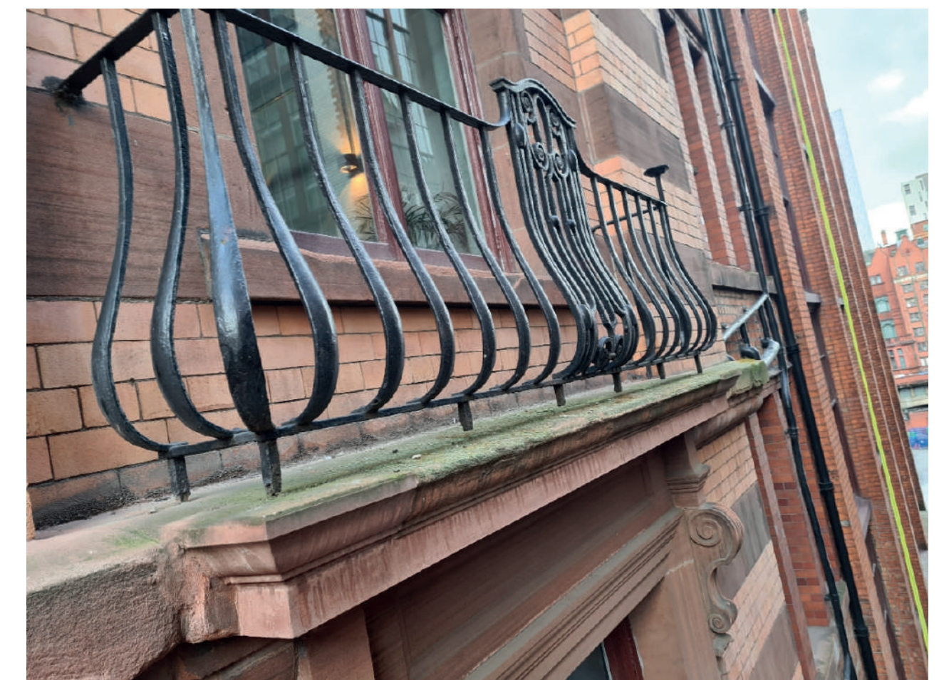
Insufficient falls contributing to biological soiling.
