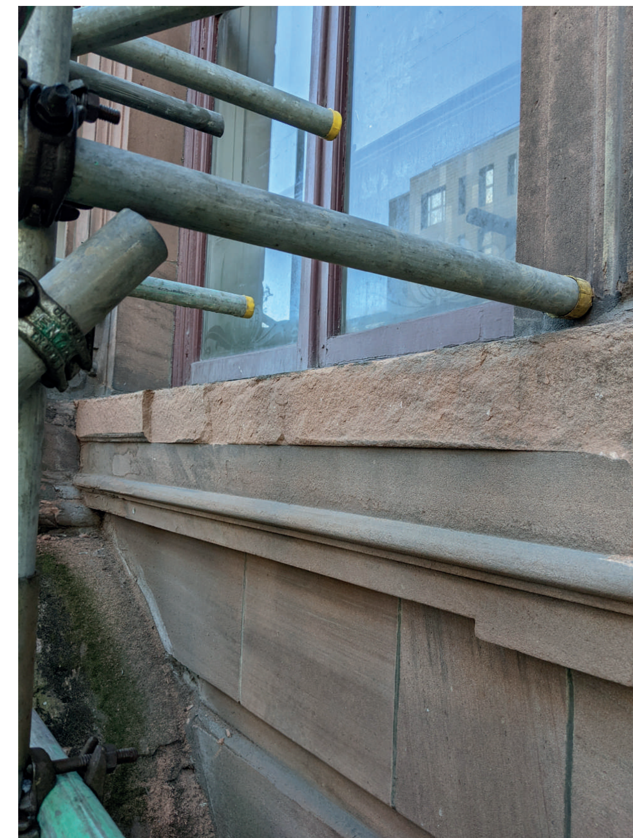
Location A05.2 - Sill face sheared off the building. This is thought to be due to the original stone having been face bedded.
