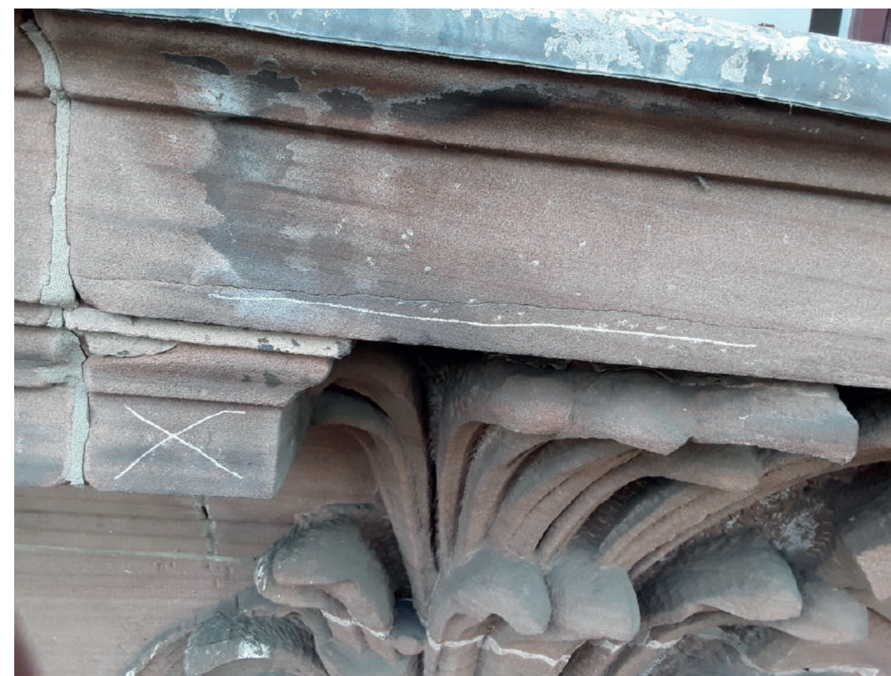
Location A04.7 - Loose stone marked with an 'x'.
