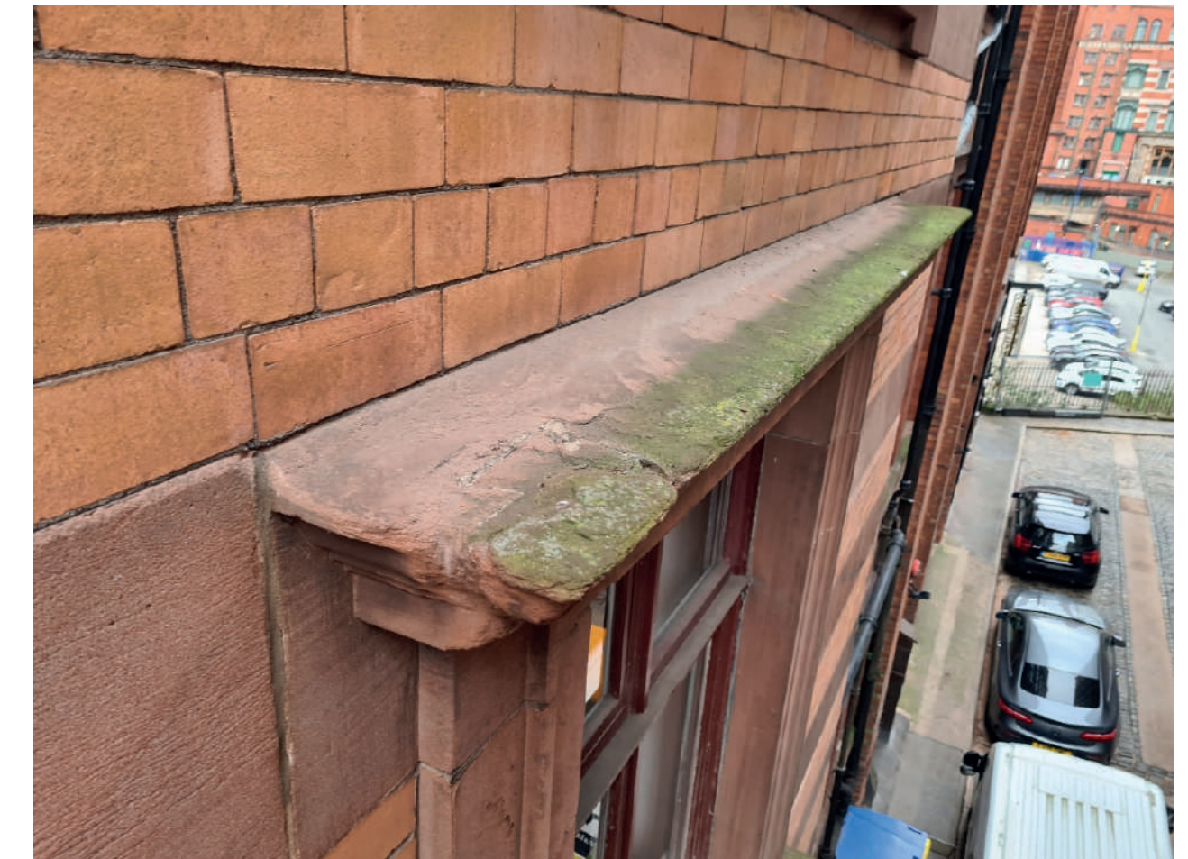
Examples of exposed horizontally bedded stone delaminating.
