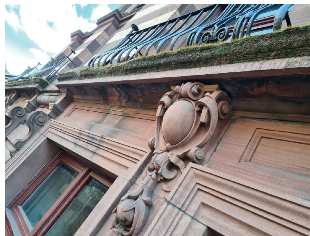
Example of biological deposits to be cleaned off.
