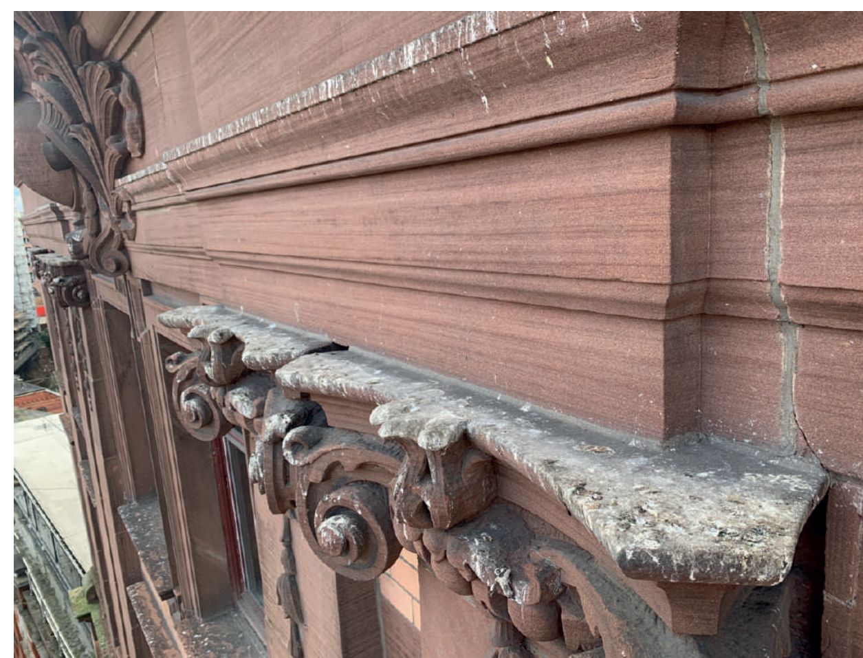
Example of guano deposits to be cleaned off.
