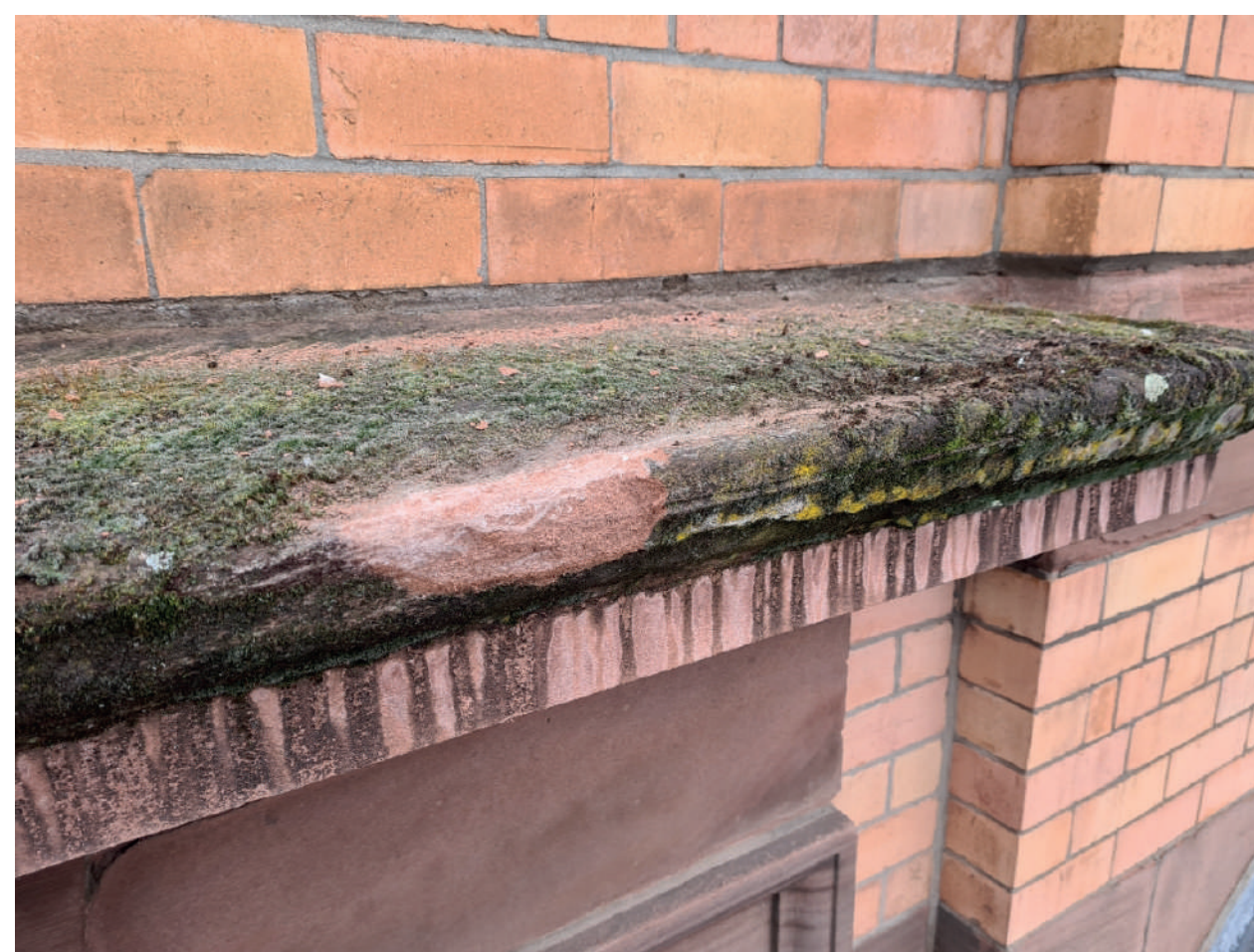
A02,8 - Significant areas of delaminated stone, and loss of original surface. Replacement proposed.
