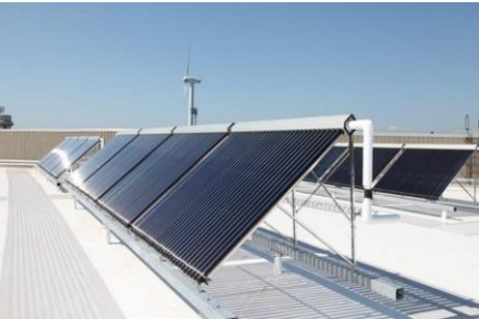
Image 6 - Solar Hot Water
