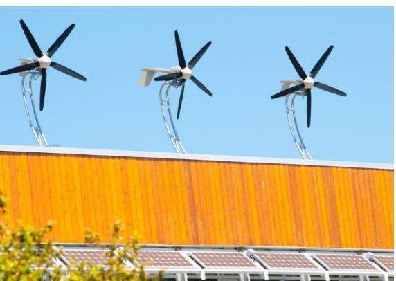
Image 10 - Roof-mounted small-scale wind turbine
