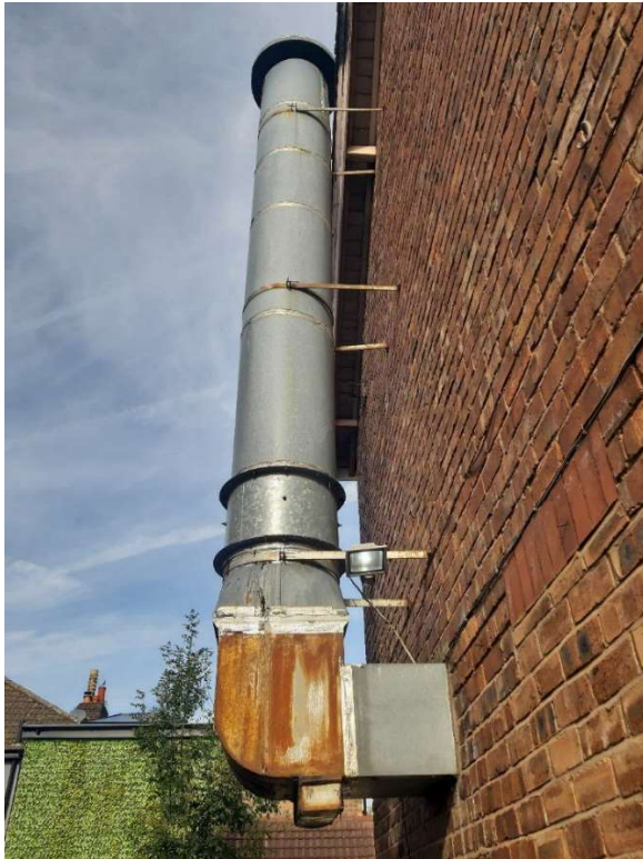
Fig 4 Existing Exhaust Flue
