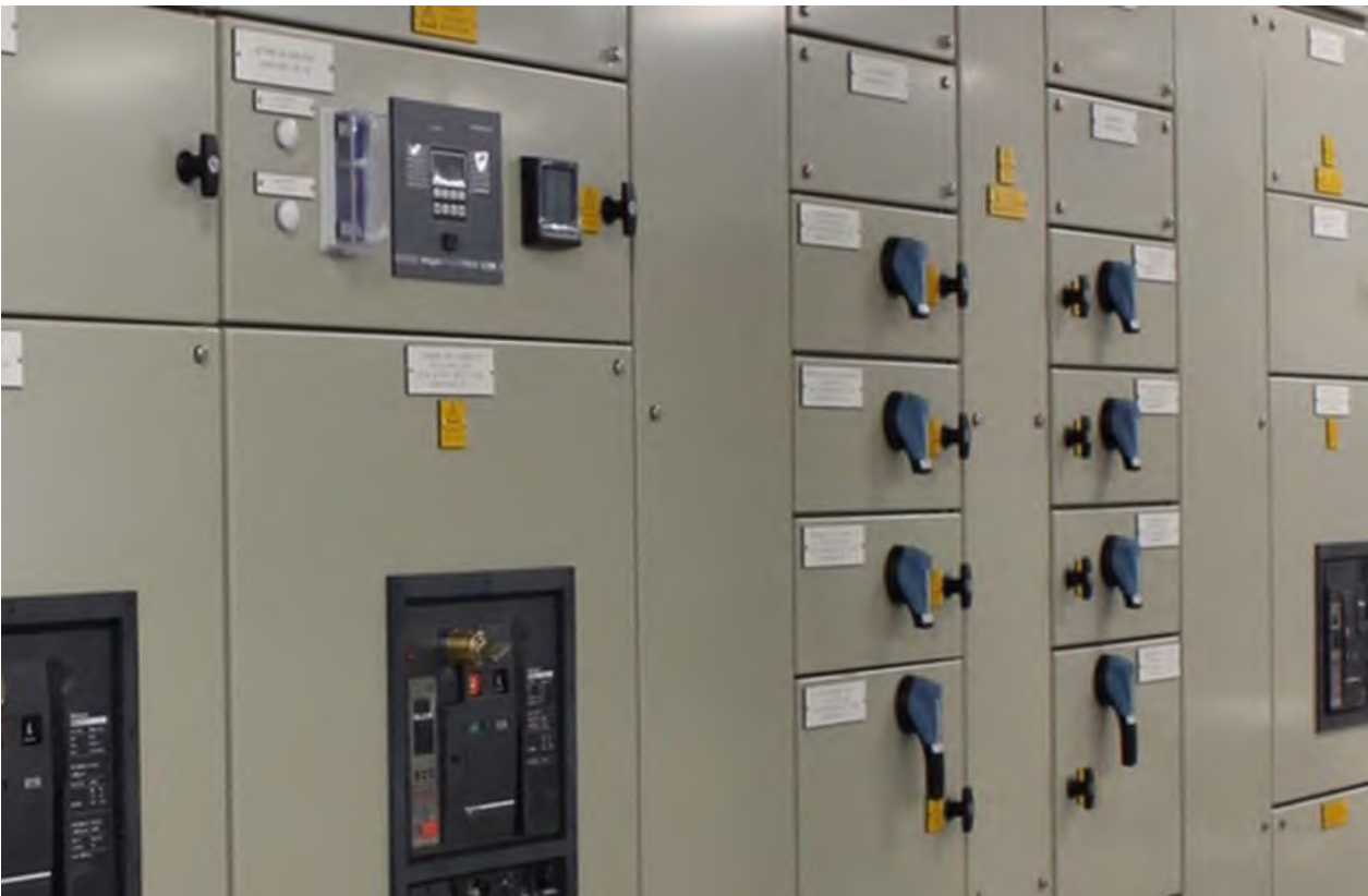
Figure 6.4.1 - Typical LV Switchboard
