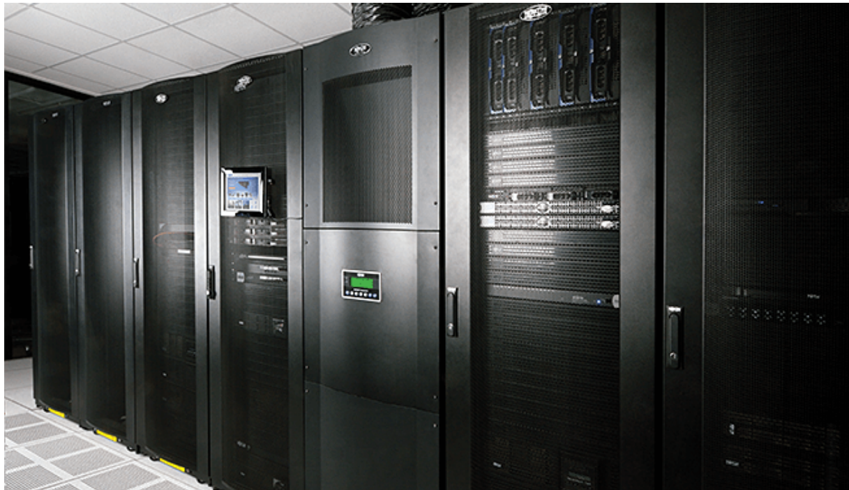
Figure 6.9.1 - Typical Comms Cabinets
