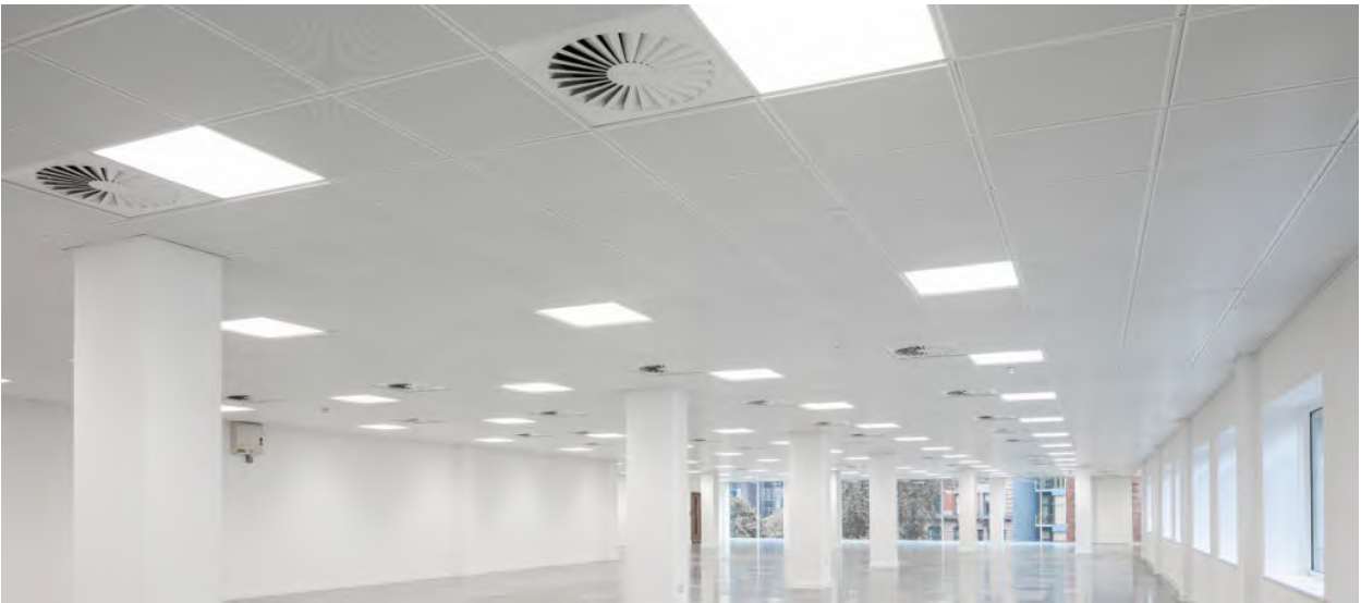
Figure 6.10.1 - Typical Cat A Office Lighting
