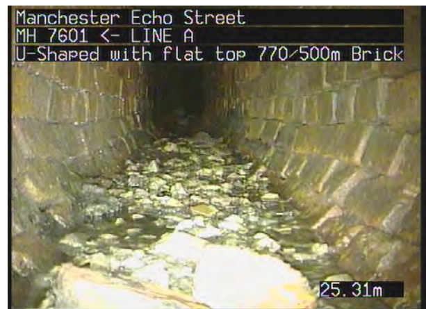
LINE A X_1350f6e7-f18e-4c30-83de-8ed6a1d86ebb_20230717_1054 47_510.jpg, 00:05:46, 25.31 m Settled deposits, fine, 25% cross-sectional area loss
