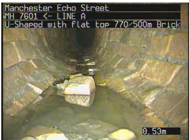
LINE A X_5350beea-e6e5-429d-901b-f2beae4cb2f4_20230717_1049 14_399.jpg, 00:01:23, 8.53 m Settled deposits, fine, 10% cross-sectional area loss, BRICK N STONE
