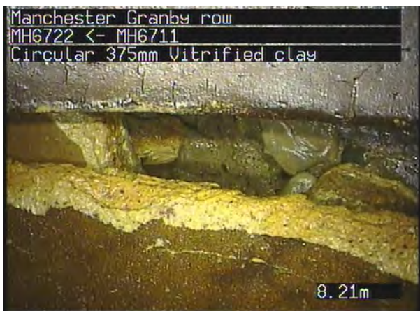
MH6711X_4194830b-2646-4cd5-b88a-7ae2284d648e_20230718_115225_973.jpg, 00:01:45, 8.21 m Broken pipe at joint from 12 o'clock to 12 o'clock
