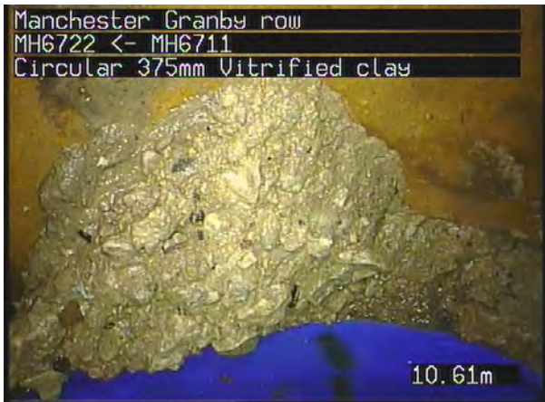
MH6711X_18627ed7-fa88-4966-898e-cf427f35350c_20230718_115342_972.jpg, 00:02:33, 10.61 m Other obstacles from 06 o'clock to 07 o'clock, 20% cross-sectional area loss, CONCRETE
