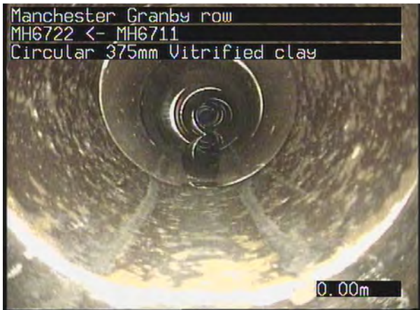
MH6711X_665136cc-919f-4a2c-8dd5-025d4d30ea0d_202307 18_115011_487.jpg, 00:00:02, 0.00 m Water level, 5% of the vertical dimension
