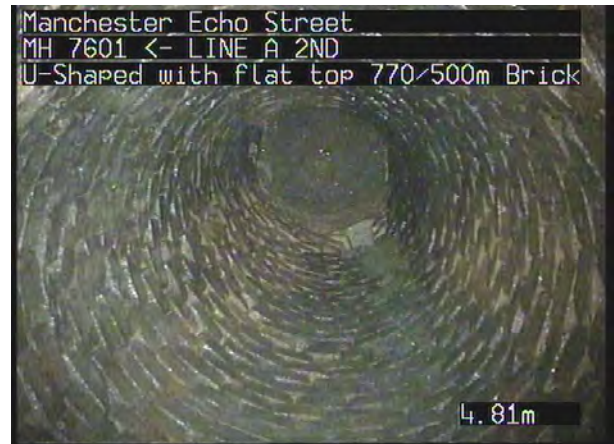
LINE A 2NDX_72aad229-d09f-4c65-9193-c3c745308ee3_20230717_ 124216_688.jpg, 00:00:42, 4.81 m General remark, BURIED MANHOLE NO LID
