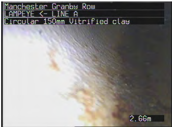
LINE A X_e83d5d0e-b85d-4e82-85ed-4c2053a91ff6_20230718_1027 14_115.jpg, 00:00:30, 2.66 m Joint displaced, medium
