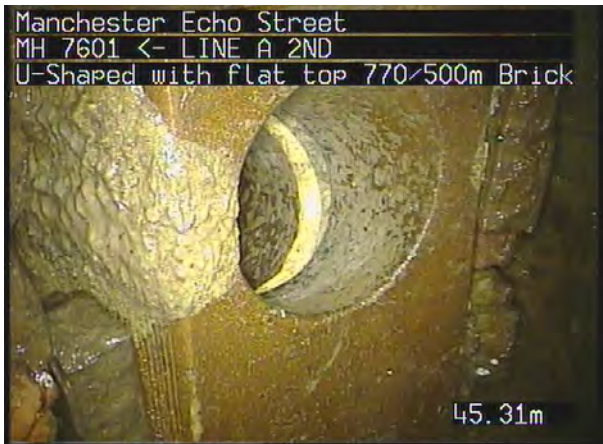
LINE A 2NDX_be57e9d6-ea52-4e9a-86f1-f9aa1cefe8f1_20230717_1 25606_134.jpg, 00:11:45, 45.31 m Connection other than junction at 11 o'clock, 150mm dia
