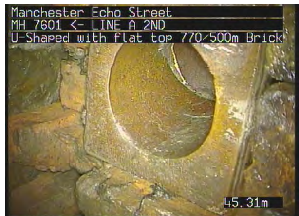
LINE A 2NDX_b5cbccc8-cd79-4971-8270-115101e578cc_20230717_125551_650.jpg, 00:11:37, 45.31 m Connection other than junction at 02 o'clock, 150mm dia
