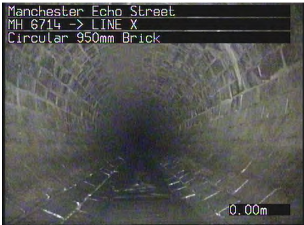
MH 6714X_a527af0a-b09e-46ec-98d4-a8c2dfa3826c_20230717_141915_249.jpg, 00:00:03, 0.00 m Water level, 10% of the vertical dimension
