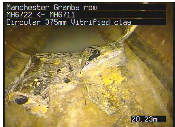
MH6711X_d5c9e128-2e23-44c6-8aa5-0bb95df380d9_20230718_120130_540.jpg, 00:06:41, 20.23 m Attached deposits, other from 04 o'clock to 07 o'clock, 10% cross-sectional area loss, CONCRETE
