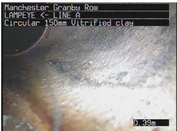
LINE A X_cd60ad08-4552-4b50-a58e-7e1d777acc8a_20230718_102 653_269.jpg, 00:00:16, 0.39 m Line deviates up
