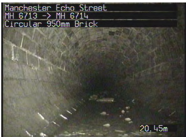
MH 6713X_8906f02f-ce2e-4482-b2a9-311778d20603_20230717_141045_442.jpg, 00:01:41, 21.27 m Settled deposits, fine, 20% cross-sectional area loss
