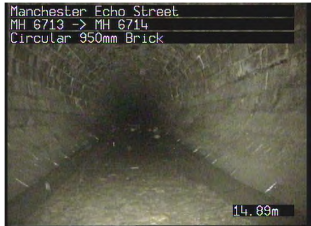
MH 6713X_613f8e99-0517-4a19-a1ff-ee0e771b08de_20230717_141011_224.jpg, 00:01:12, 14.90 m Settled deposits, fine, 15% cross-sectional area loss
