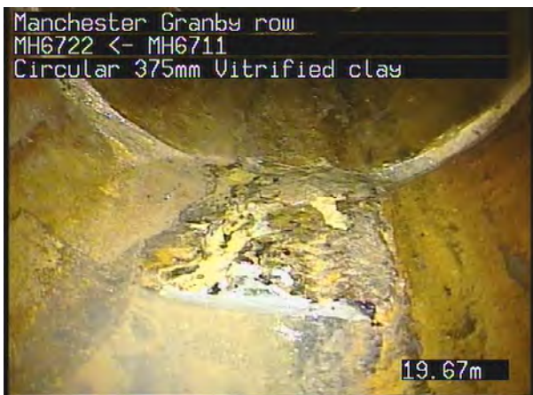
MH6711X_55bc5f45-bd57-4dbc-92d4-6759f58b6a2f_20230718_120059_276.jpg, 00:06:30, 19.67 m Attached deposits, other at 09 o'clock, 5% cross-sectional area loss, CONCRETE
