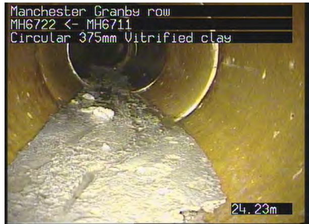
MH6711X_59fe7c64-8d6d-46d2-bdf0-cf9b3594be25_20230718_120249_679.jpg, 00:07:34, 24.23 m Attached deposits, other from 04 o'clock to 07 o'clock, 20% cross-sectional area loss, CONCRETE
