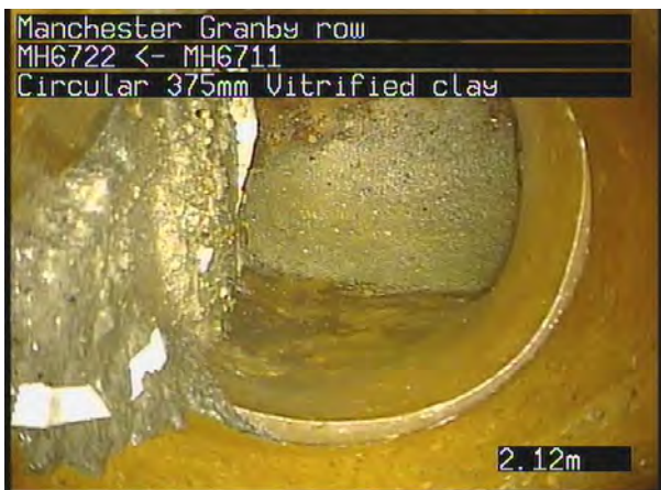
MH6711X_e4dfaa13-8daa-4022-b960-b2f4b1205e42_202307 18_115046_229.jpg, 00:00:29, 2.12 m Junction at 09 o'clock, 150mm dia
