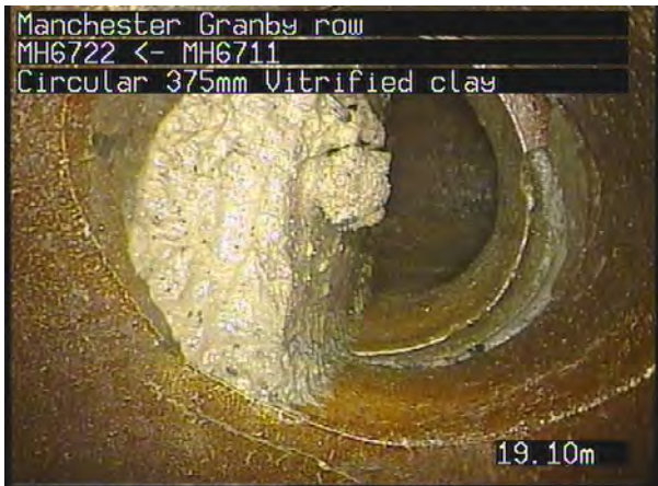
MH6711X_fa476d7c-e33d-4136-9587-b13d9317a760_20230718_115915_685.jpg, 00:05:45, 19.10 m Junction at 09 o'clock, 150mm dia
