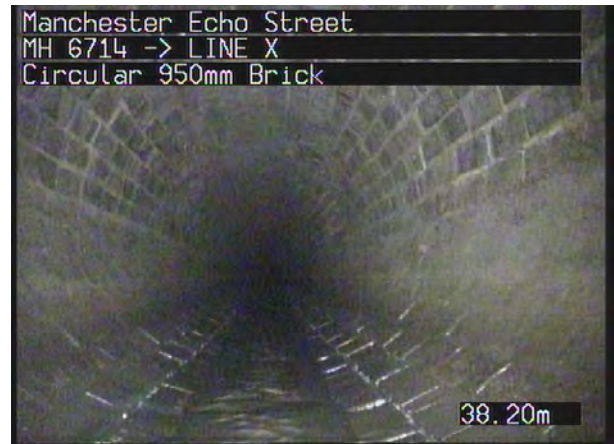
MH 6714X_b2d108cc-3c43-4efa-bb00-41c72b0d2543_20230717_142206_134.jpg, 00:02:37, 38.20 m Survey abandoned, OFF BOUNDARY LINE
