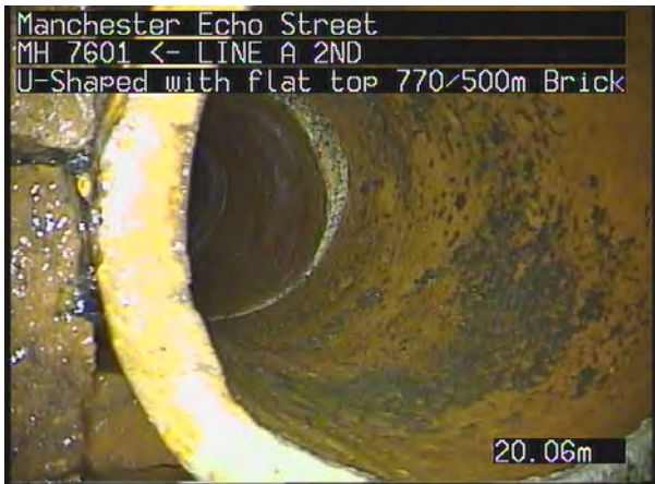
LINE A 2NDX_8f6a7a56-df09-4f09-a727-39e1557c3611_20230717_1 24528_952.jpg, 00:02:45, 20.06 m Connection other than junction at 10 o'clock, 225mm dia
