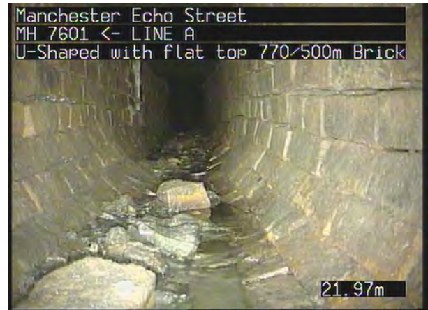
LINE A X_270a0a84-9673-494f-8284-e51a4adb76ea_20230717_105 214_410.jpg, 00:03:28, 21.97 m Settled deposits, fine, 20% cross-sectional area loss, STONE N BRICK
