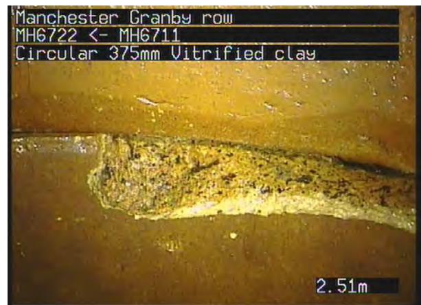
MH6711X_c14feb4c-a9ec-450a-93ac-521bec3bd889_202307 18_115111_329.jpg, 00:00:47, 2.51 m Broken pipe at joint from 02 o'clock to 04 o'clock
