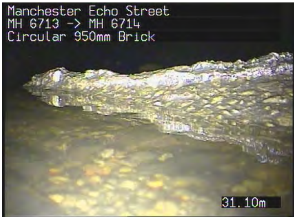
MH 6713X_a1e33c7e-6ee3-4ae8-9263-8819fb3a78da_20230717_141424_346.jpg, 00:04:19, 31.10 m Other obstacles from 05 o'clock to 06 o'clock, 10% cross-sectional area loss, PIECE OF TARMAC
