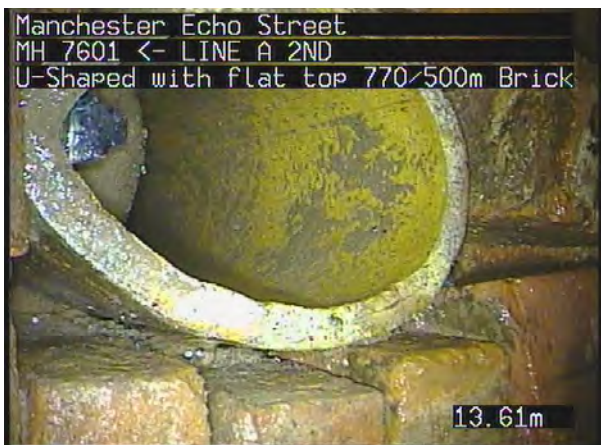
LINE A 2NDX_4c24f6c7-ffb6-411c-abb9-565782ae4efc_20230717_12 4329_034.jpg, 00:01:36, 13.61 m Connection other than junction at 10 o'clock, 225mm dia, EGG VC
