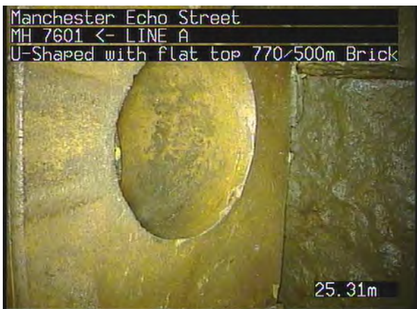
LINE A X_3f42fa24-4b32-4baf-ac52-75a5ba51614b_20230717_10542 7_629.jpg, 00:05:33, 25.31 m Connection other than junction at 11 o'clock, 150mm dia
