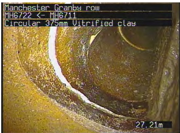
MH6711X_19de32e6-c3e9-482d-8f31-9d2adaa55481_20230718_120350_394.jpg, 00:07:56, 27.21 m Junction, other at 02 o'clock, 150mm dia, CONCRETE COMING FROM JUNCTION
