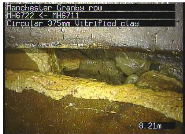
MH6711X_dec4dd89-6f8b-49ac-afbc-482d24593ba9_20230718_115230_455.jpg, 00:01:49, 8.21 m Void visible beyond defect
