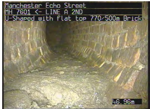
LINE A 2NDX_33b50735-a69f-4a53-95bc-5c75659f7b33_20230717_1 25635_921.jpg, 00:12:07, 46.96 m Settled deposits, fine, 25% cross-sectional area loss
