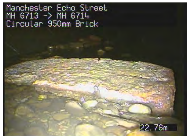
MH 6713X_788a78cf-8aa5-4dda-99ae-20ba25fd7099_20230717_141233_612.jpg, 00:03:08, 22.76 m Other obstacles, brick or masonry in invert at 06 o'clock, 20% cross-sectional area loss
