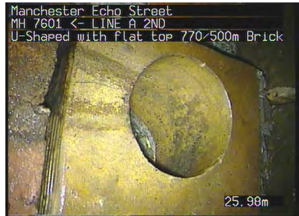
LINE A 2NDX_6abe0f08-0129-4271-9e56-47bc61c8b2ab_20230717_ 124631_366.jpg, 00:03:39, 25.98 m Connection other than junction at 11 o'clock, 150mm dia
