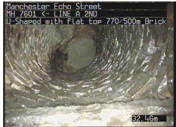
LINE A 2NDX_0f67b30e-fd9b-496a-92bf-a2917fef1d4c_20230717_125301_977.jpg, 00:09:01, 32.46 m General remark, BURIED MANHOLE NO LID
