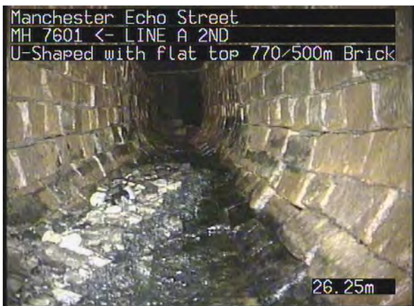
LINE A 2NDX_048f4e84-3533-4ece-b2e2-b7602a37bc85_20230717_ 124706_211.jpg, 00:03:54, 26.25 m Settled deposits, fine, 15% cross-sectional area loss, STONE NSILT
