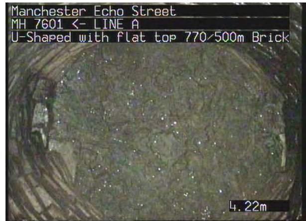
LINE A X_c8a0c224-e695-4ad6-b4af-debe01c157fc_20230717_1048 15_819.jpg, 00:00:43, 4.22 m General remark, BURIED MANHOLE NO LID
