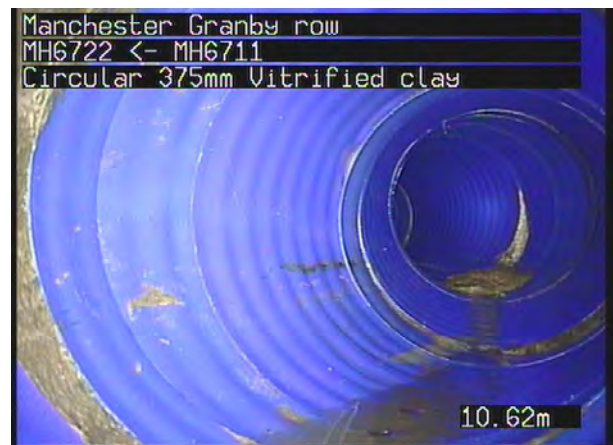
MH6711X_beefbb52-6744-4688-80d0-1fd9b7b21494_20230718_115415_508.jpg, 00:02:55, 10.62 m Pipe material changes to polyvinyl chloride at this point
