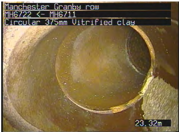
MH6711X_7201a499-521a-46db-af01-6402e3fec686_20230718_120219_418.jpg, 00:07:19, 23.32 m Connection other than junction at 02 o'clock, 225mm dia
