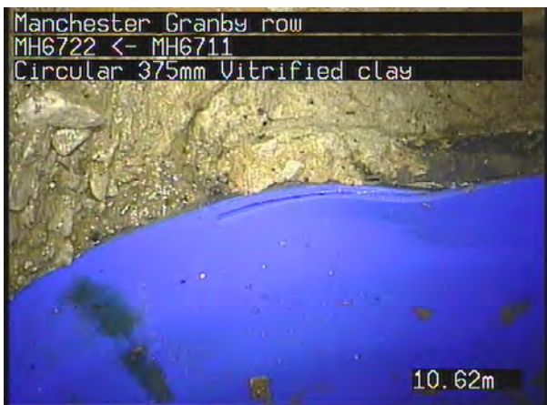
MH6711X_7c12078a-cc50-4b70-8bd7-e067bc56a60d_20230718_115400_760.jpg, 00:02:45, 10.62 m Void visible beyond defect
