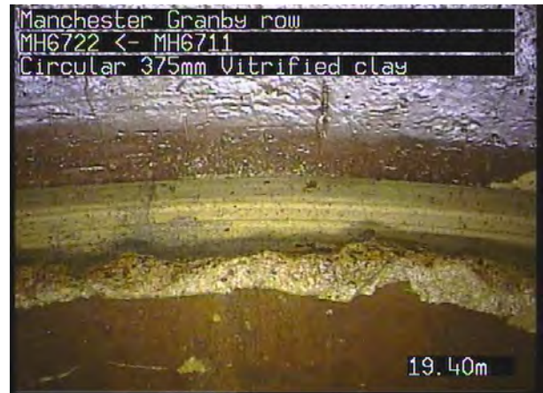
MH6711X_933ac639-f2e9-428c-bb4d-c3b1e01c25b2_20230718_115951_427.jpg, 00:06:15, 19.40 m Broken pipe at joint from 12 o'clock to 12 o'clock
