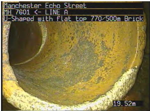
LINE A X_1f4c68be-4d7f-46d6-a618-db3a4450f03e_20230717_10513 2_599.jpg, 00:03:02, 19.52 m Connection other than junction at 10 o'clock, 225mm dia
