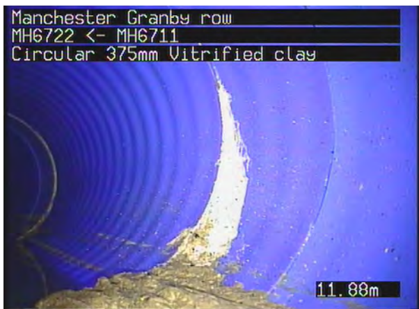
MH6711X_d0cd7441-7a70-40d8-9414-5019e0961be7_20230718_115551_290.jpg, 00:03:16, 11.88 m Line deviates left
