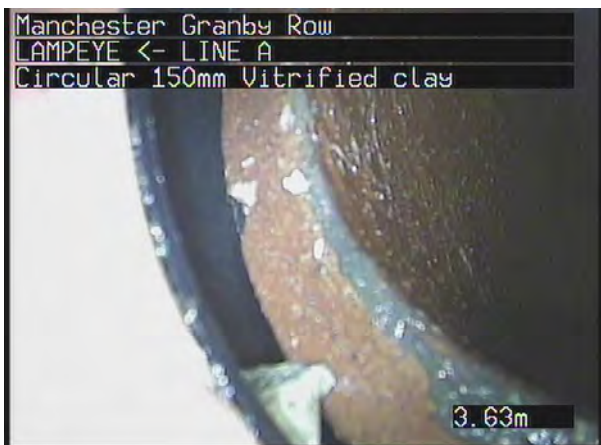
LINE A X_e7d89ef1-3036-4fef-a44e-82615515e760_20230718_1027 36_562.jpg, 00:00:48, 3.63 m Joint displaced, large
