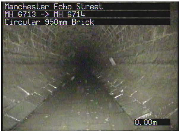
MH 6713X_ab701b4e-8436-4255-a2c0-0e9bc589ab84_20230717_140857_586.jpg, 00:00:04, 0.00 m Water level, 20% of the vertical dimension
