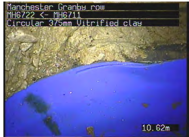
MH6711X_ed51d130-f2d9-42cf-a06b-123c7563c678_20230718_115355_765.jpg, 00:02:41, 10.62 m Open joint, large
