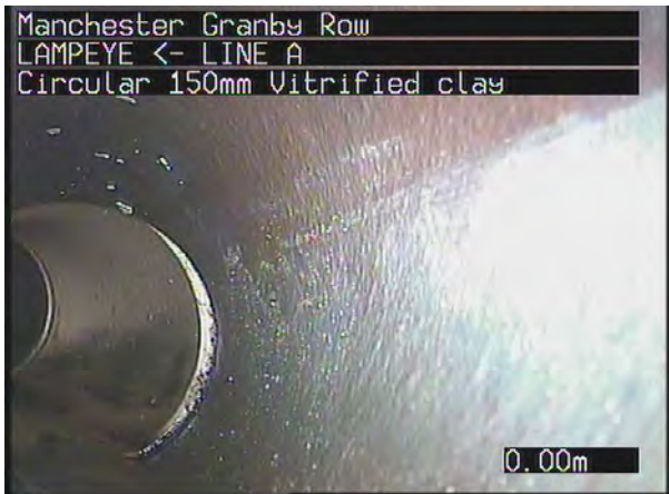
LINE A X_8f9a27bb-62ca-4cf3-85bf-7fc34367e498_20230718_10263 7_718.jpg, 00:00:03, 0.00 m Water level, 5% of the vertical dimension
