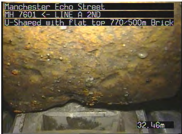
LINE A 2NDX_14d2c551-5794-427a-b58b-3bd3f292be7a_20230717_125116_965.jpg, 00:07:32, 32.46 m Other obstacles, brick or masonry in invert from 04 o'clock to 07 o'clock, 35% cross-sectional area loss
