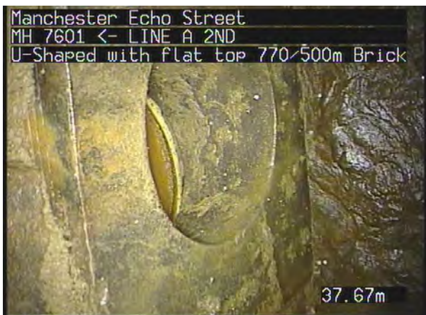
LINE A 2NDX_672b2ed2-a908-4c38-8c6b-618fc1ecfb66_20230717_125454_647.jpg, 00:10:47, 37.67 m Connection other than junction at 11 o'clock, 150mm dia
