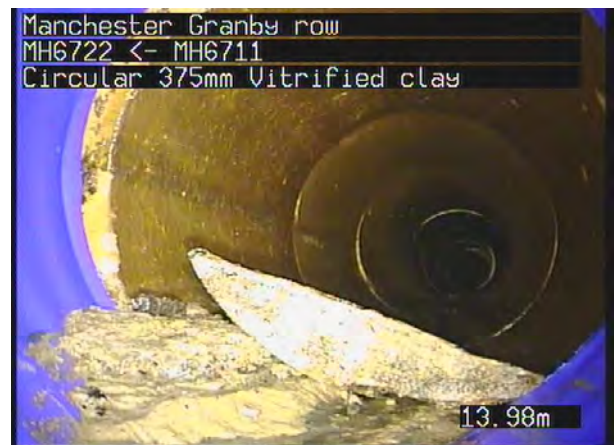
MH6711X_ccf1d9c3-8408-459e-ade5-588497a06963_20230718_115637_060.jpg, 00:03:34, 13.98 m Other obstacles from 04 o'clock to 08 o'clock, 30% cross-sectional area loss, CONCRETE
