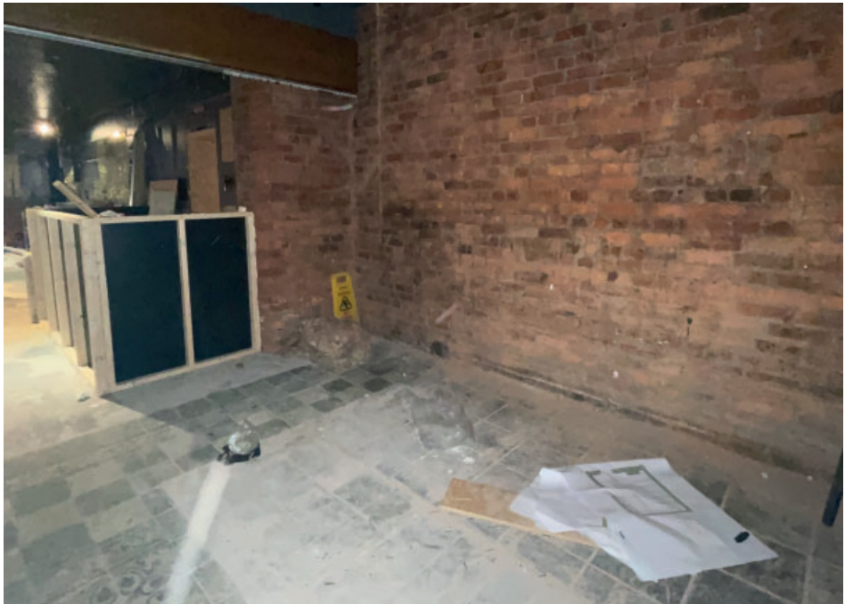
10 View to location of new store. Timber studs to be replaced.
