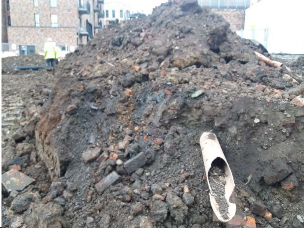
Photograph 5: Ashy excavated soils remaining from the hotspot excavation.
